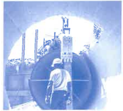
Mokelumne Aqueduct No. 3 is 7 feet 3 inches in diameter. An adult can easily stand up inside a replacement pipe for the aqueduct. Wooden braces keep the heavy pipe round.
