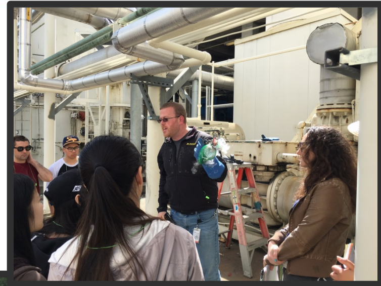
Oxygen plant, SD-1
