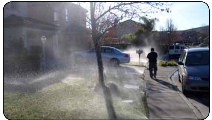
Existing pressure exceeded 100 psi. Pressure regulation devices and rotating nozzles installed on new sprinklers helped to improve irrigation efficiency and to reduce overall water costs.
