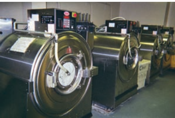
Laundry and kitchen equipment are elements of a water use efficiency assessment completed for the West County Jail facility.
