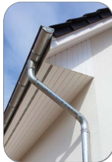
Asphalt shingle roof with Aluminum gutter and downspout Courtesy of Sonoma County
