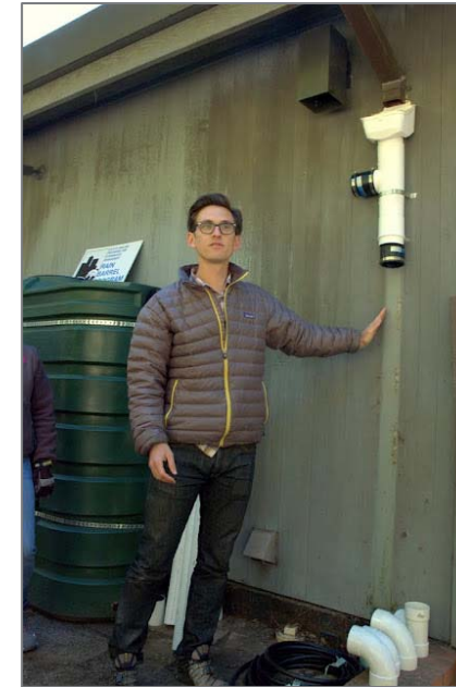
First flush and downspout diverter installation Courtesy of The City of Oakland
