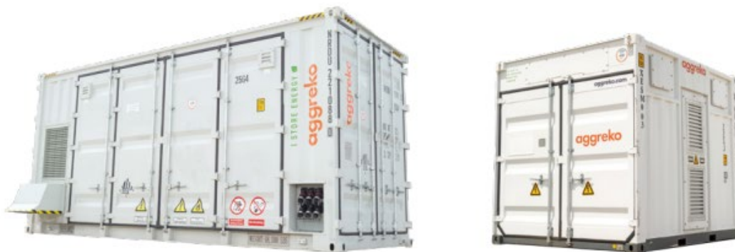
FIGURE 3: LITHIUM-ION BATTERY UNIT AND INVERTER
