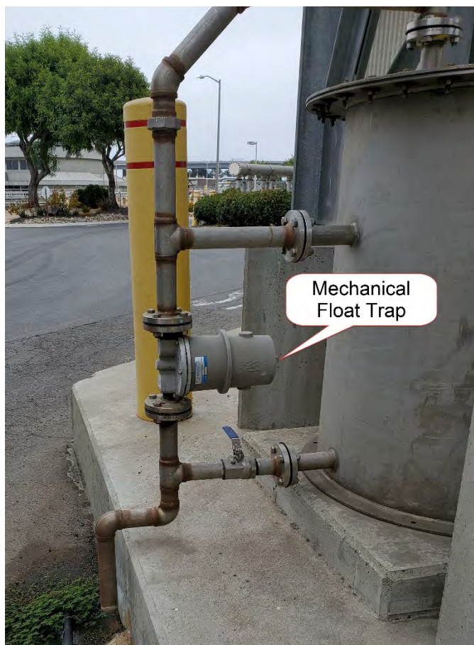
Figure 39 - Similar Condensate Drip Trap with Mechanical Float Installed in Overflow Leg
