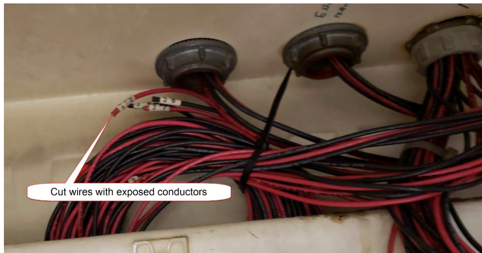
Figure 17: Severed Wires in PGS-1 Fire Detection Panel
