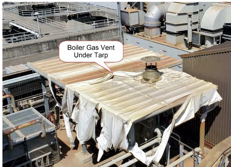
Figure 8 – Boiler Gas Vent Terminates Under Tarp
