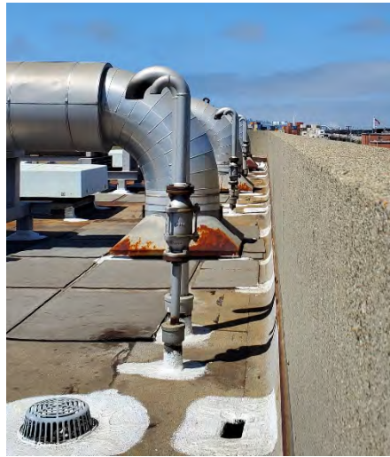
Figure 7 – Engine Vent Piping
