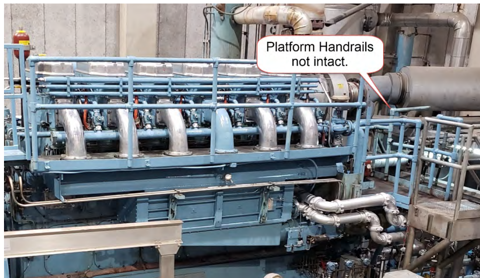
Figure 12 - Platform Handrail not Correctly Installed
