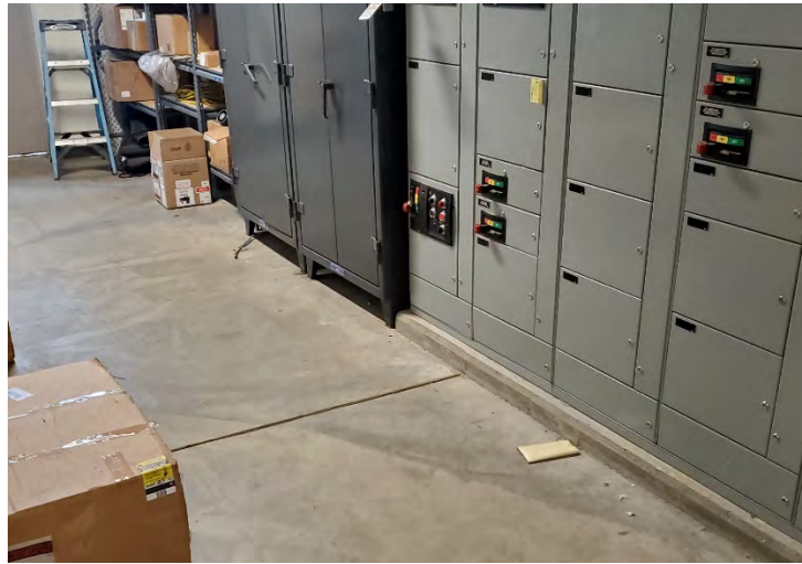
Figure 30 – Panel without Electrical Safety Mat
