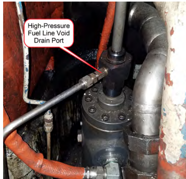
Figure 37: High Pressure Fuel Line with Drain Port (From Another Site)
