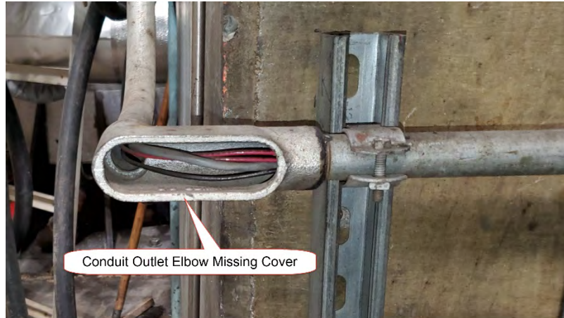
Figure 29 – Conduit Elbow Missing Cover
