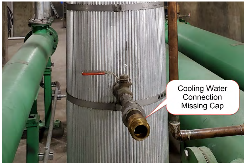
Figure 28 - Cooling Water System Uncapped Connection
