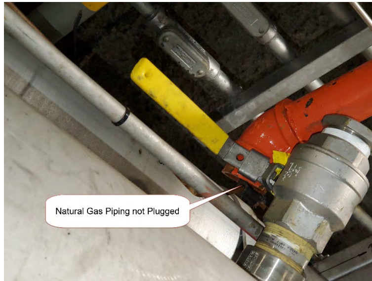
Figure 24 - Natural Gas Piping Open to Engine Room
