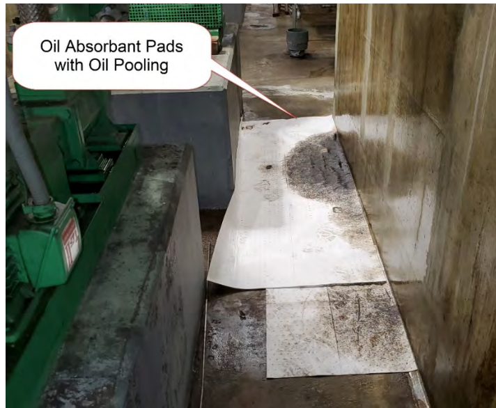
Figure 32 - Oil Absorbent Pads in Basement
