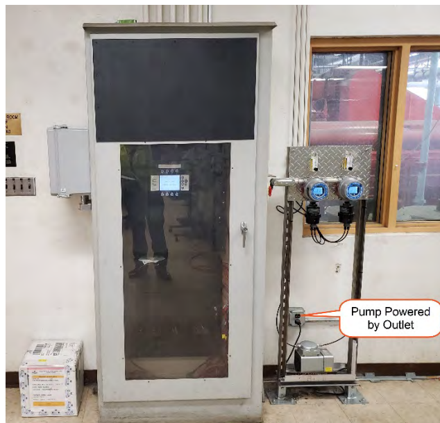
Figure 15: PGS-1 Fire Detection and Gas Detection Panels
