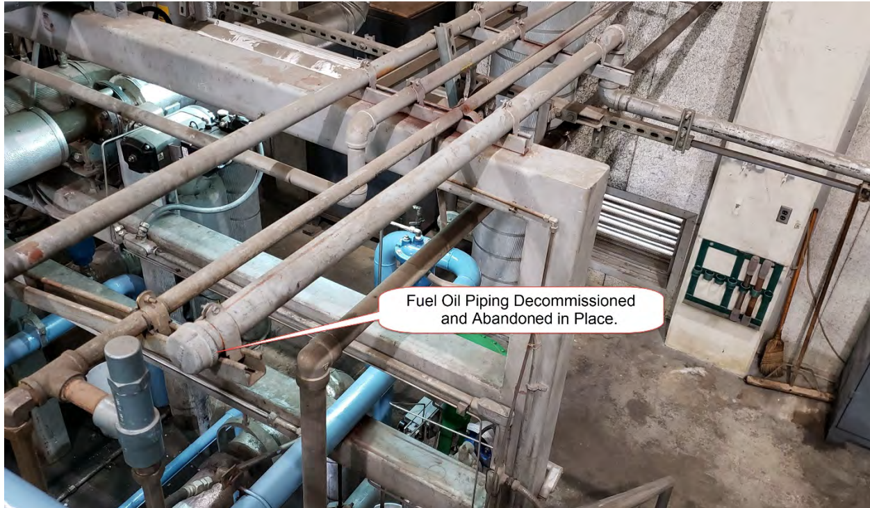
Figure 27 - Decommissioned and Abandoned in Place Piping
