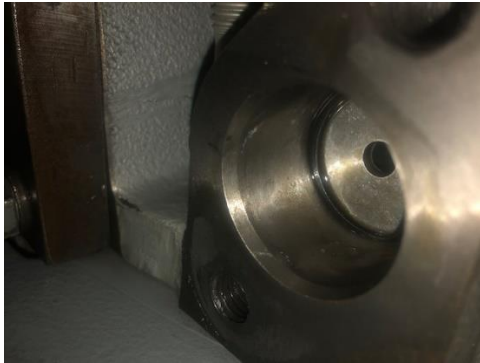
Unit 2 inlet oil supply orifice.
