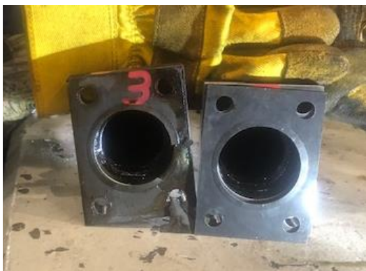
Units #2 and #3 turbocharger drain line pipes.
