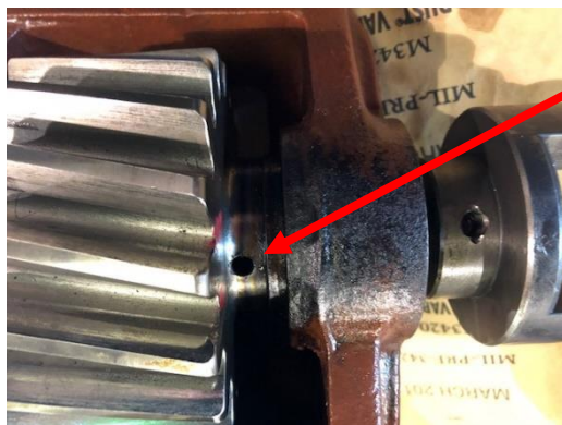
Bushing and gear with coked oil (oil cokes at 260° F) on gear carrier housing.
