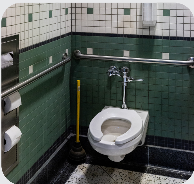
Flush Valve Toilet in a Commercial Bathroom
