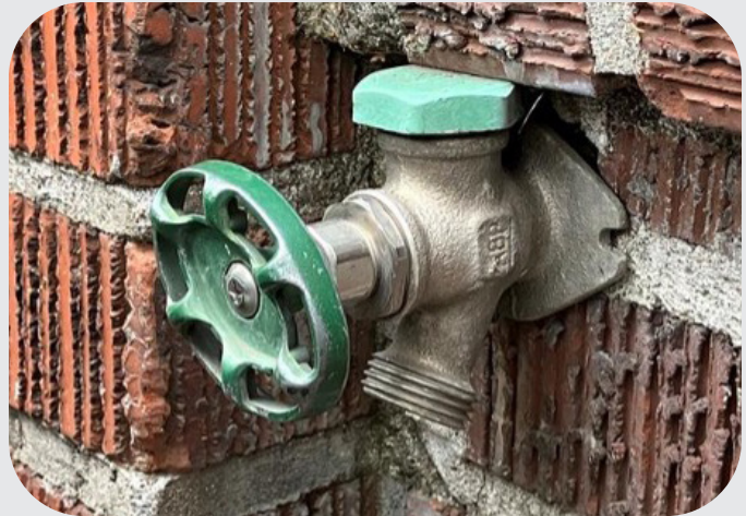
Hose Bib Outside of a Commercial Business
