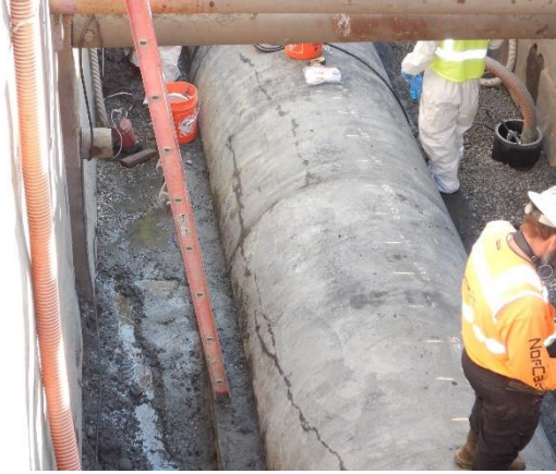
Photo 2-17. Overall view of longitudinal cracks at the 12:00 to 3:00 position from Stn. 0+13 to Stn. 0+36.
