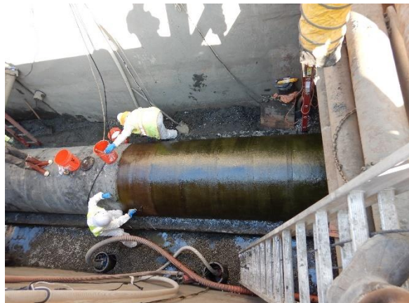
Photo 2-14. Up to 13 feet of pipe were wrapped with 4 layers of fiberglass reinforcing.
