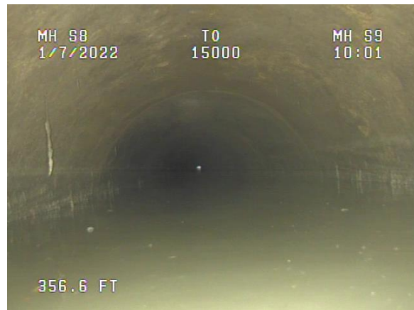
Photo 2-10. The pipe is in VANDA Level 2 condition at Stn. 3+56.6.
