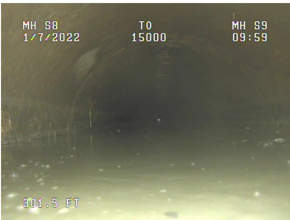
Photo 2-9. The pipe is in VANDA Level 2 condition at Stn. 3+01.5.
