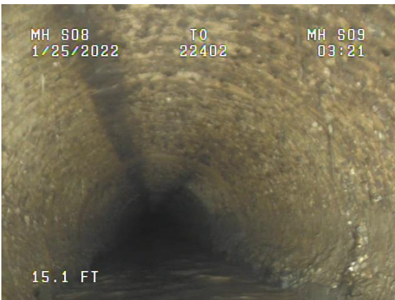
Photo 2-3. VANDA Level 5 condition at Stn. 0+15.1 from the 8:00 to 4:00 position.
