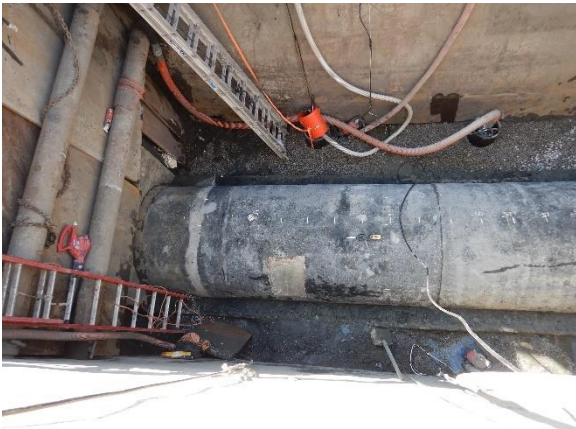
Photo 2-11. The pipe wall at the 2:30 position at Sta. 0+06 was severely deteriorated and damaged.
