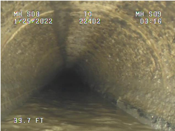
Photo 2-5. The pipe is in VANDA Level 4 condition from the 8:00 to 4:00 position at Stn. 0+39.7.
