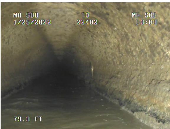
Photo 2-7. The pipe is in VANDA Level 3 condition at Stn. 0+79.3.
