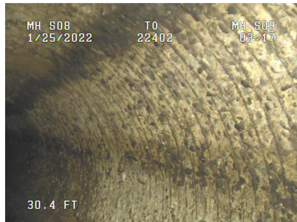
Photo 2-4. Exposed reinforcing steel at the 12:00 at Stn. 0+30.4.
