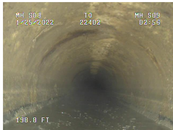
Photo 2-8. The pipe is in VANDA Level 2 condition at Stn. 1+98.8.
