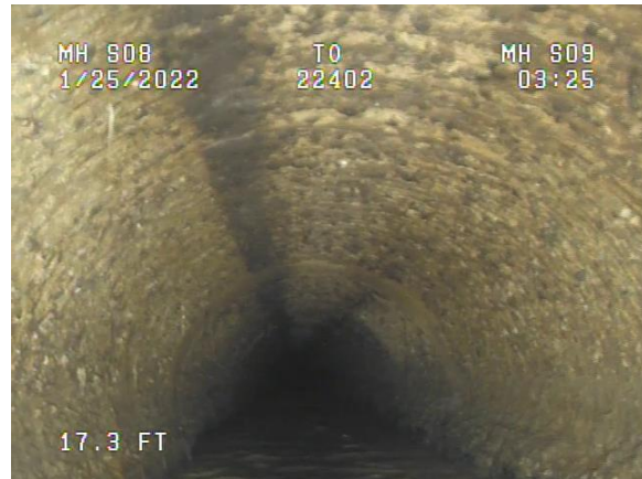
Photo 2-2. The pipe is in VANDA Level 5 condition from the 8:00 to 4:00 position at Stn. 0+17.3.
