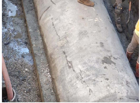
Photo 2-18. Longitudinal cracks at the 1:00 to 2:00 position from Stn. 0+28 to Stn. 0+36.
