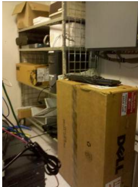
Figure 6. Storage in Computer Room
