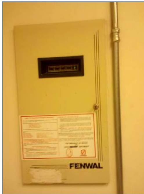
Figure 2. Fenwal Control Unit
