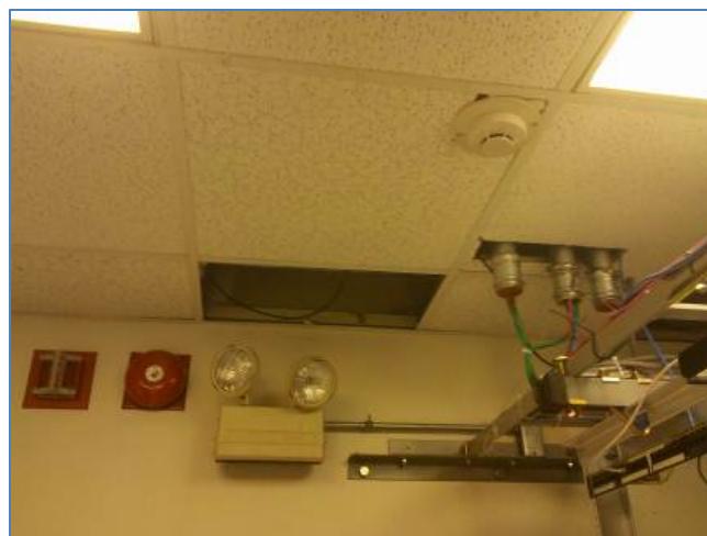
Figure 3. Detector and Notification Equipment
