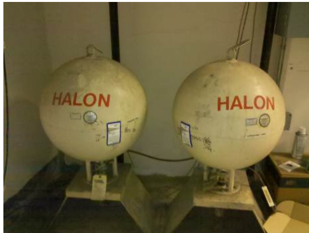
Figure 18. Separate Halon Cylinders for Ops Control and Computer Rooms
