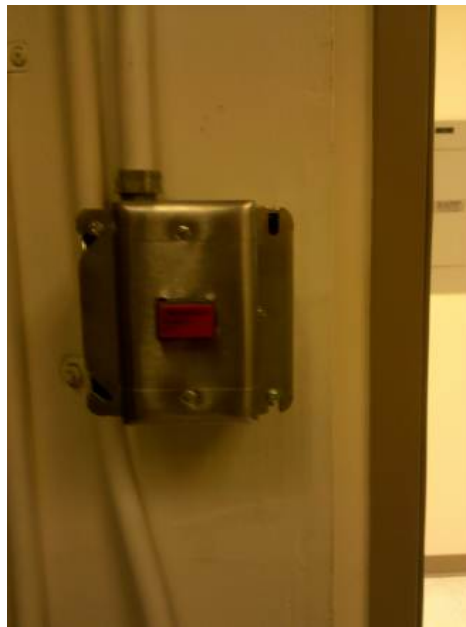
Figure 10. Emergency Power Off/Disconnect
