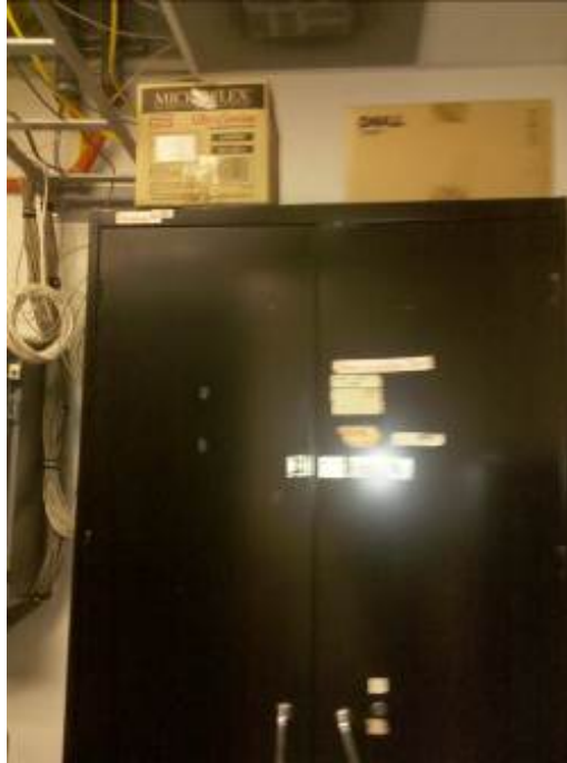
Figure 7. Storage in Computer Room
