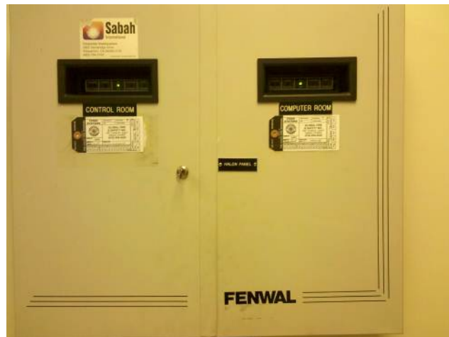
Figure 16. Fenwal Control Units for both Ops Control and Computer Rooms (located in Computer Room)
