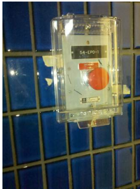
Figure 15. Emergency Power Off (typical for both Ops Control and Computer Rooms)
