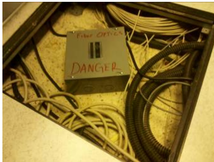
Figure 8. Sub-floor Debris and Cabling
