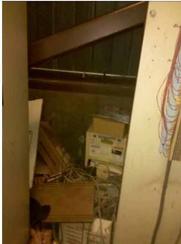
Figure 12. Miscellaneous Debris and Storage
