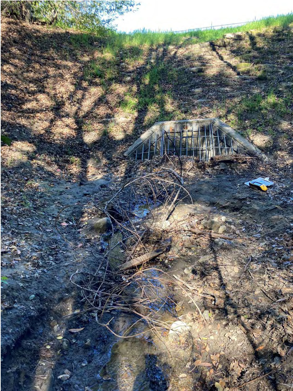
Photo 5. IC-3 is hydrologically connected to IC-1 via a culvert that flows north under the water treatment plant. Photo facing north. March 8, 2022
