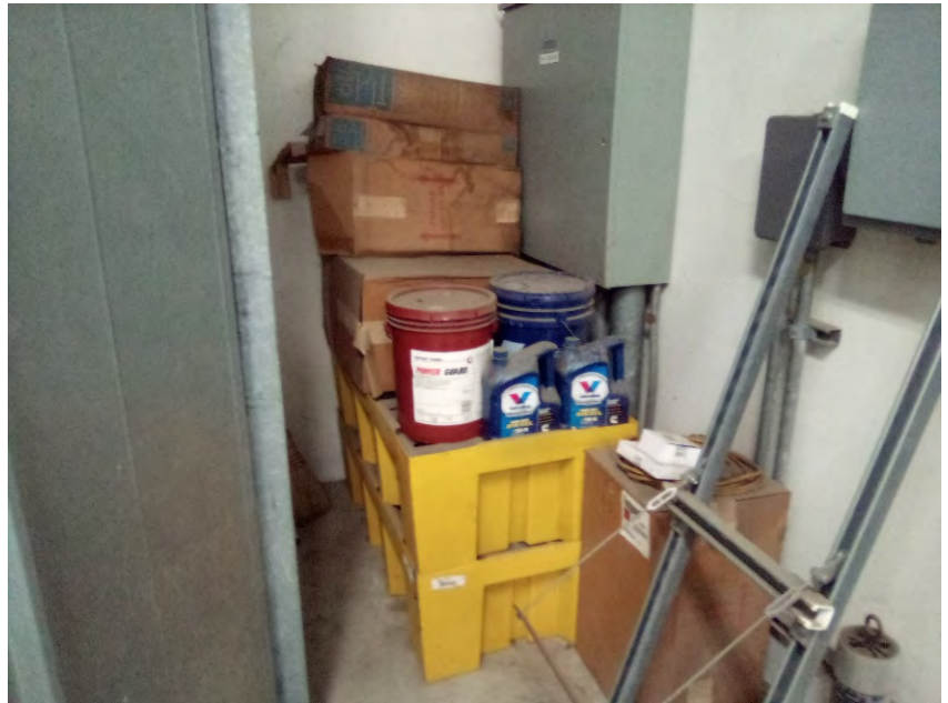
Photo 18: View of motor oil and lubricants stored in secondary containment within the generator building.
