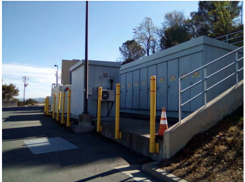
Photo 15: View of the generator building and switchgear building, as viewed from the northwest.
