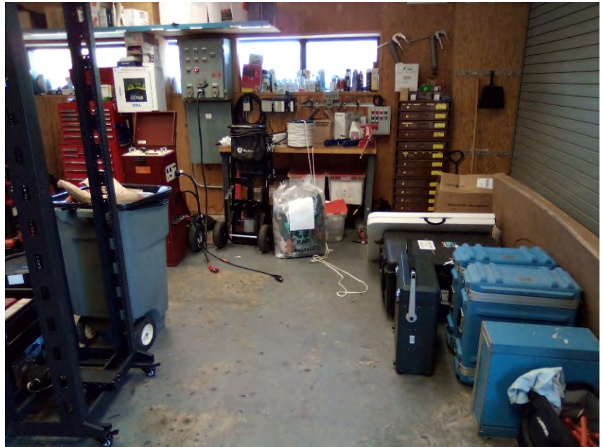
Photo 7: View of the interior of the electrical and instrument control building.
