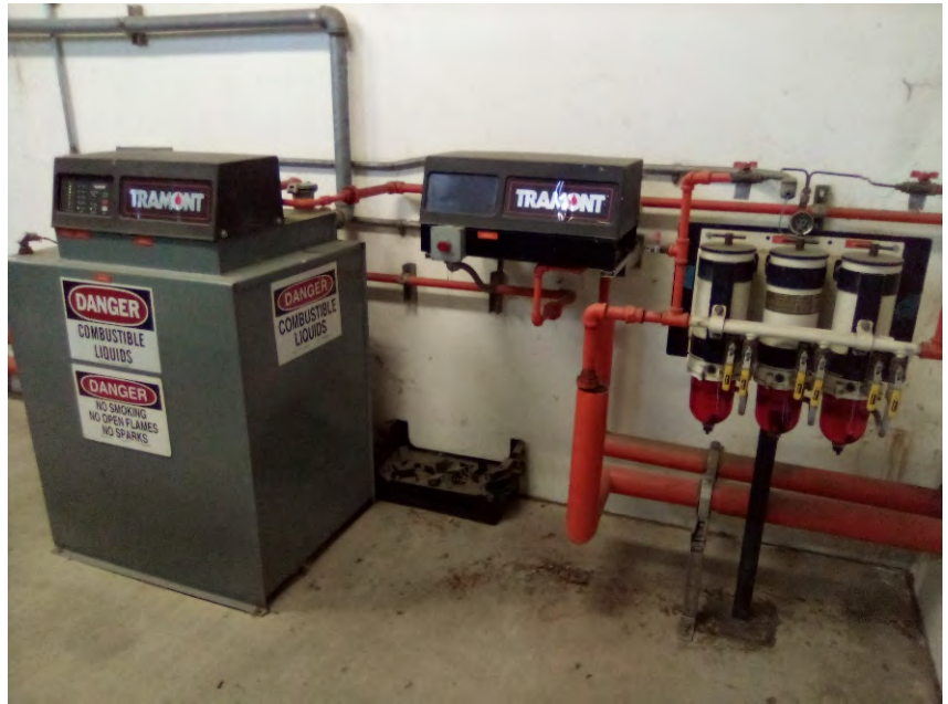
Photo 17: View of the diesel storage tank in the generator building.
