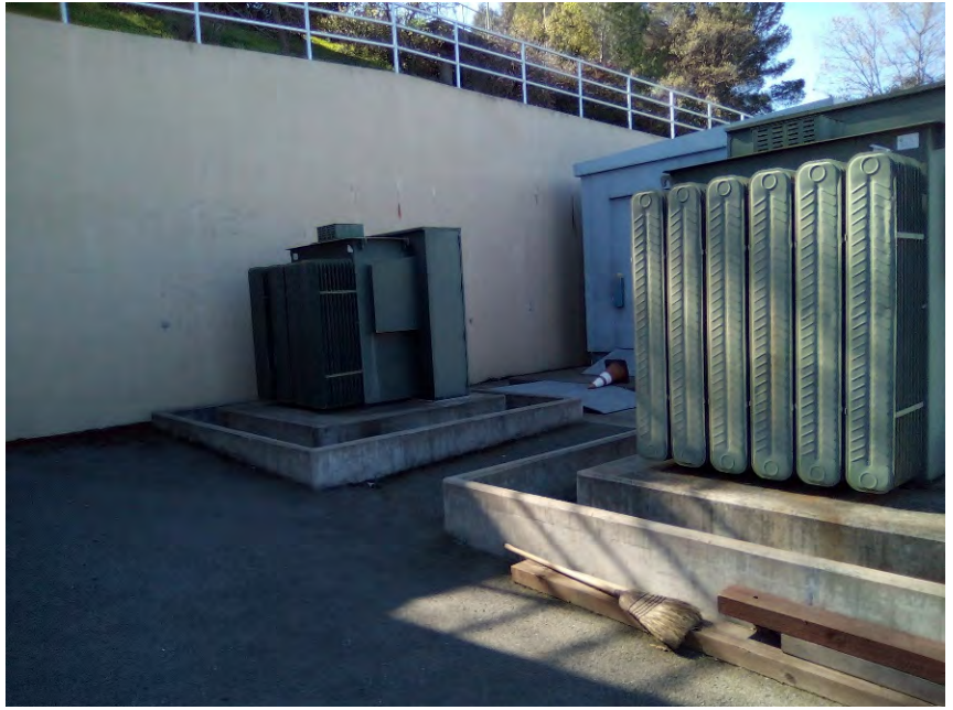
Photo 19: View of two transformers adjacent to the generator building and switchgear building, as viewed from the northwest.
