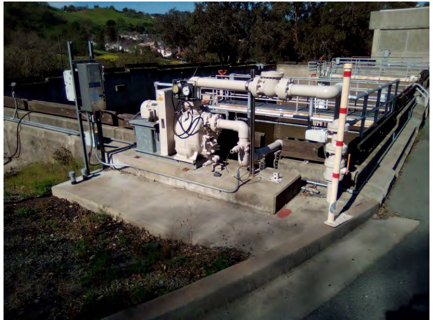
Photo 22: View of the decant pump, as viewed from the south.
