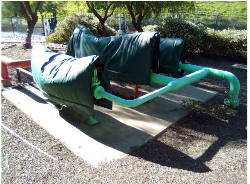
Photo 4: View of the backflow preventers, as viewed from the north.
