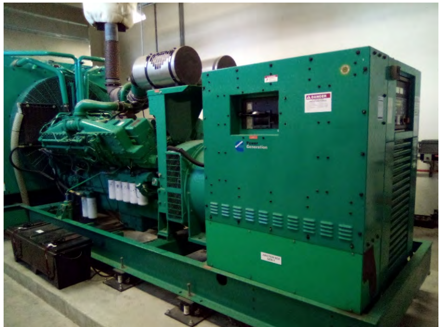
Photo 16: View of the emergency generator in the generator building.
