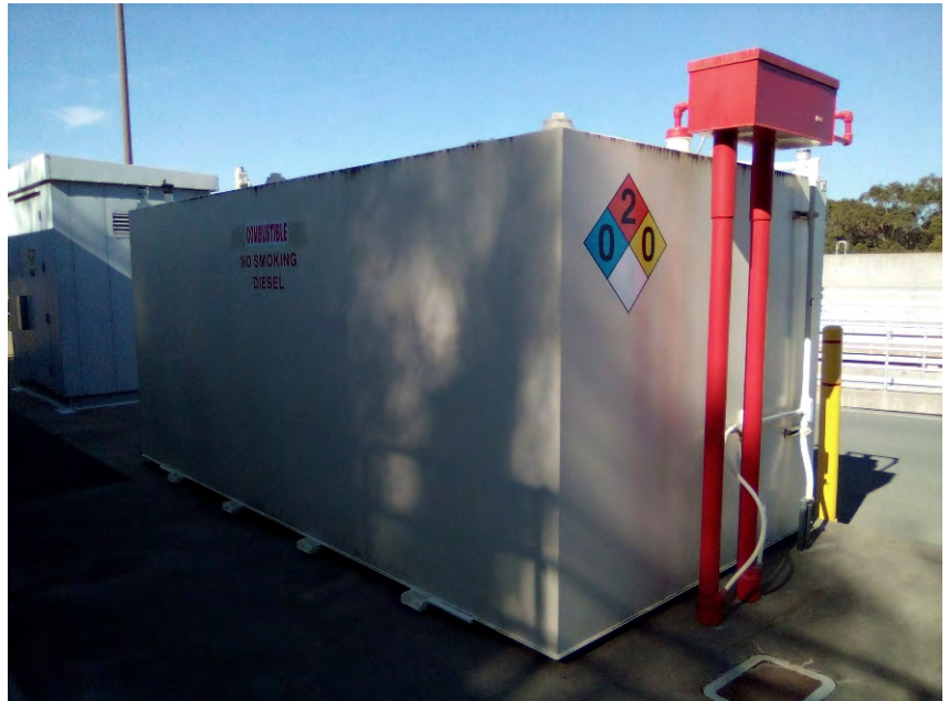
Photo 20: View of the 5,000-gallon aboveground diesel storage tank, as viewed from the south.
