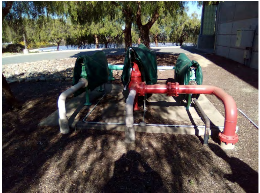
Photo 5: View of the backflow preventers, as viewed from the south.
