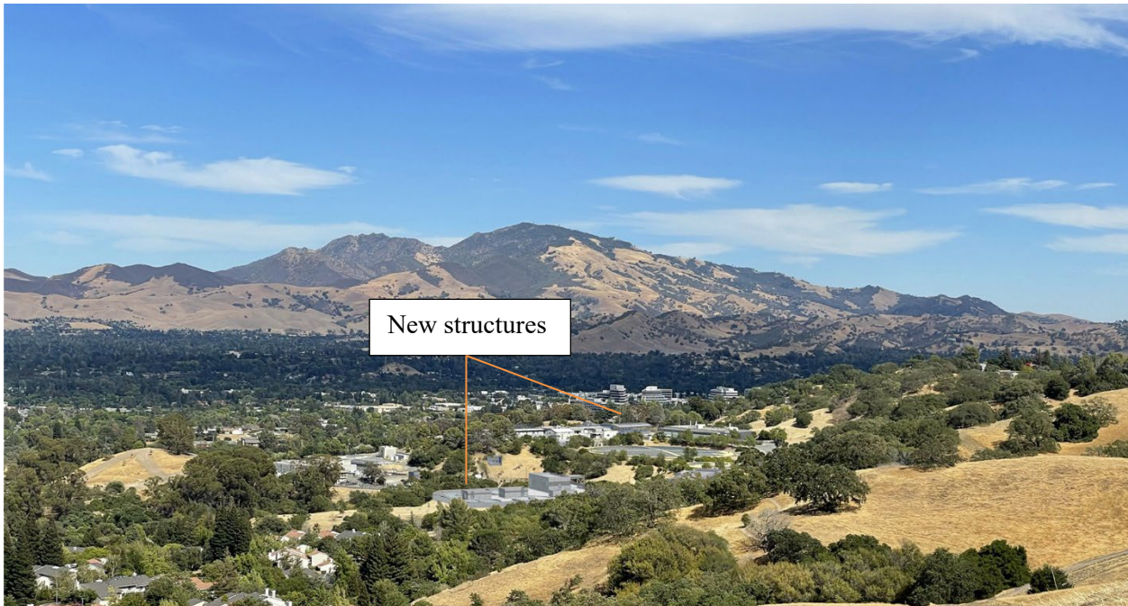
After Construction - Consolidated Maintenance Building, Pre-Ozone Pumping Plant, Thickened Solids Pumping Plant, and Gravity Thickeners, and Ballasted Flocculation structure partially visible
