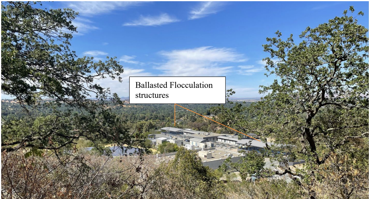
After Construction - Ballasted Flocculation structures on the north and south ends of the existing Operation Building, and partial view of Intermediate Ozone Contactor
