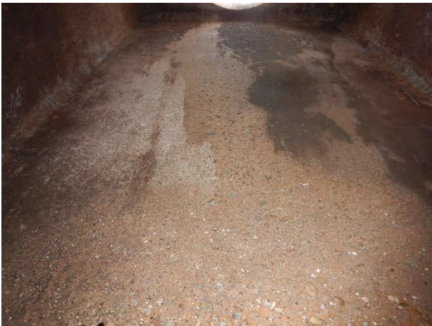
Photo S14 - 5. Bench wall, some exposed aggregate and discoloration.
