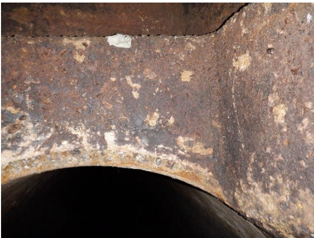
Photo S16 – 3. Crown of downstream pipe, exposed longitudinal reinforcement ends.
