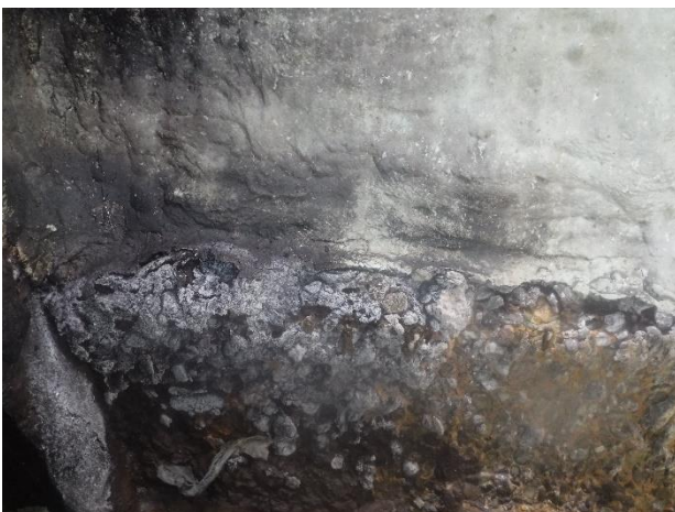
Photo A47 - 5. Exposed aggregate on interceptor-manhole joint.
