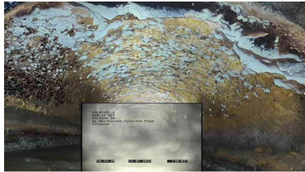
10, 00:03:58, 130.00ft Surface Damage Aggregate Projecting from 9 o'clock to 10 o'clock, within 8 inch
