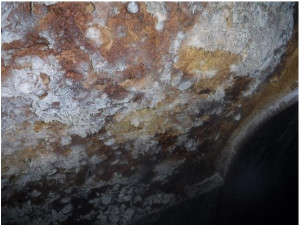
Photo 3-36. MH A37, moderate surface damage on manhole channel.
