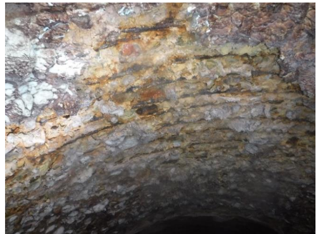
Photo A47 - 4. Crown of downstream pipe, exposed circumferential rebar is corroded.
