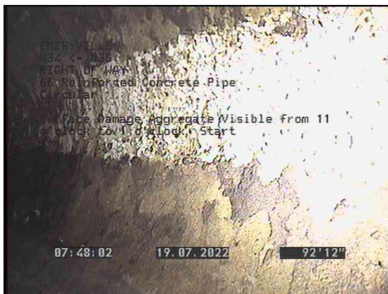
5, 00:03:57, 92.98ft Surface Damage Aggregate Visible from 11 o'clock to 1 o'clock, Start
