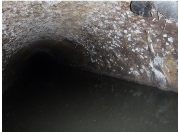
Photo A48 - 2. Upstream pipe, exposed aggregate, damaged coating, and exposed rebar.
