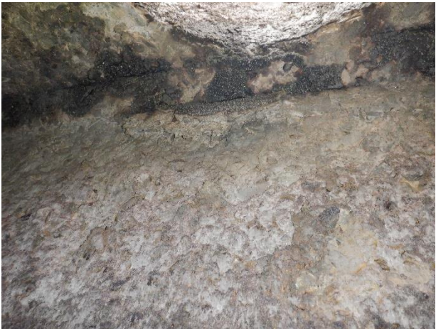
Photo 4-33. MH S15. Severe surface damage on upper section of manhole, soft concrete surface.
