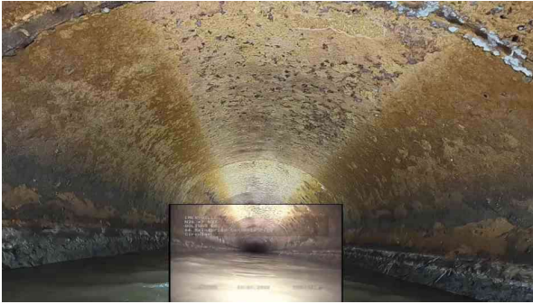
7, 00:08:22, 76.00ft Surface Damage Aggregate Projecting from 11 o'clock to 2 o'clock, within 8 inch, Finish / PROJECTING
