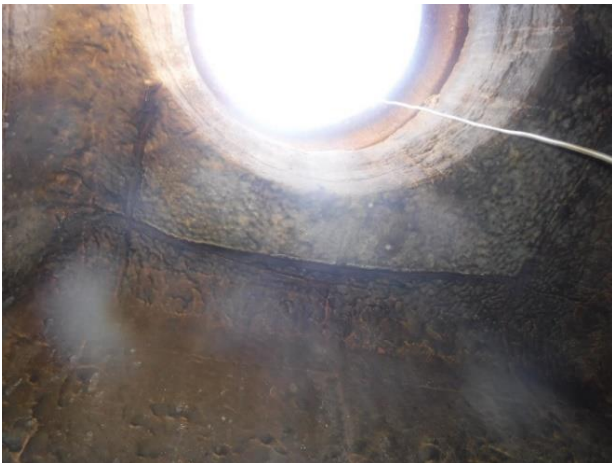
Photo 3-32. MH A35. Failed lining, exposed aggregate, and exposed reinforcing steel on ceiling.
