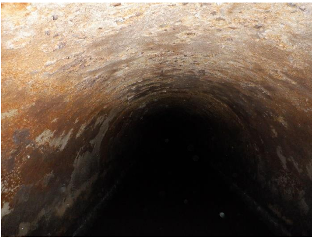
Photo N26 - 1. Upstream pipe, surface damage on crown of pipe.
