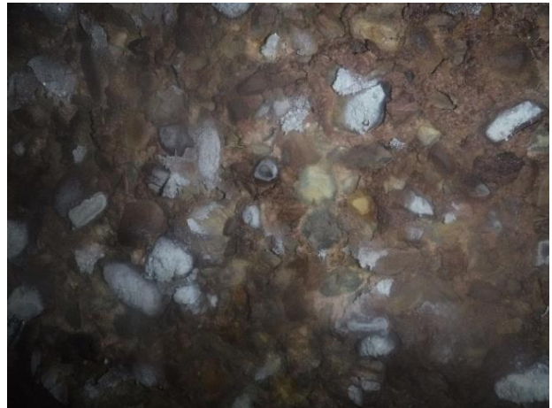
Photo A48 - 4. Exposed aggregate in upstream pipe.
