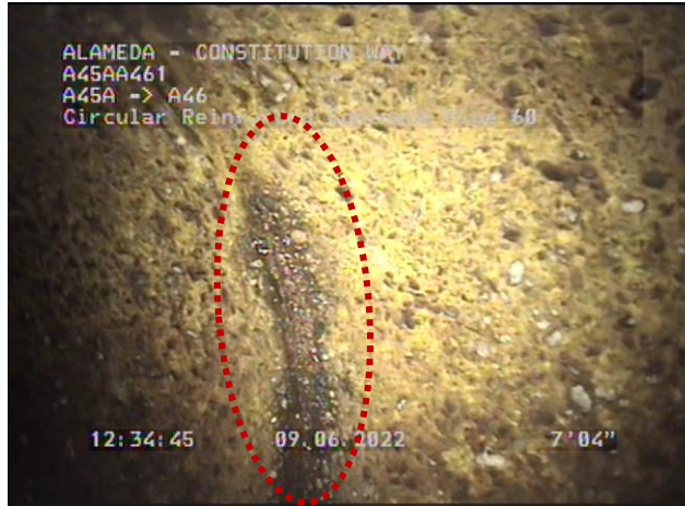
Photo 3-18. Infiltration at joint at 7 feet downstream from A45A
