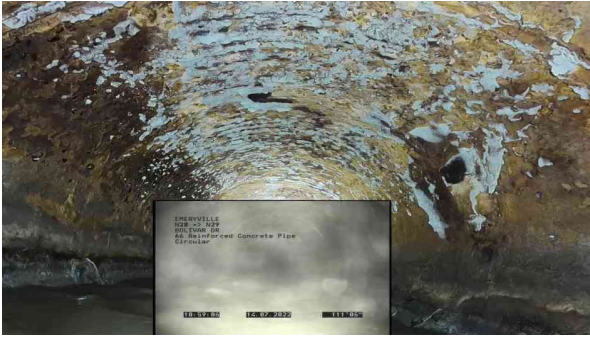
7, 00:03:43, 111.70ft Surface Damage Reinforcement Visible from 11 o'clock to 1 o'clock, within 8 inch, Start
