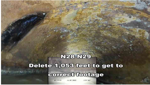
7, 00:08:19, 139.90ft Infiltration Stain Joint from 9 o'clock to 11 o'clock, within 8 inch
