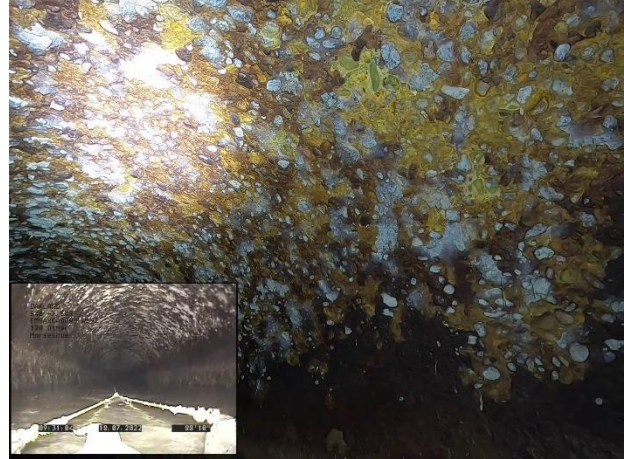
Photo 4-14. Typical severely deteriorated yellowish-white surface of 105-inch pipe with exposed aggregate; S48S491 shown
