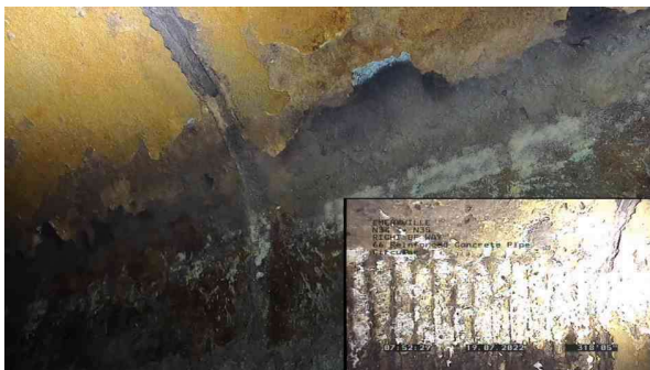
11, 00:08:29, 374.40ft Surface Damage Reinforcement Visible from 11 o'clock to 1 o'clock, within 8 inch, Finish
