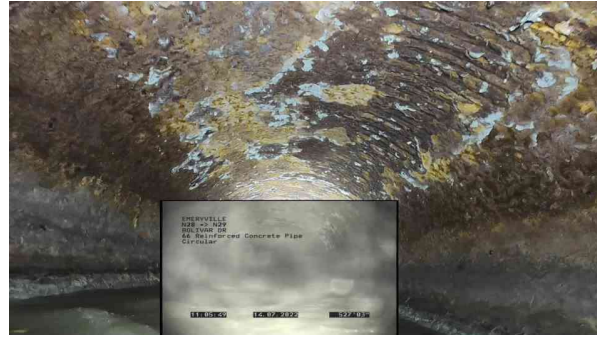
20, 00:10:27, 527.80ft Surface Damage Reinforcement Visible from 12 o'clock to 3 o'clock, within 8 inch, Start
