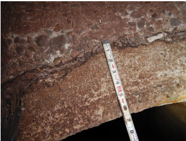
Photo S39 - 5. Exposed aggregate on manhole structure wall above upstream pipe opening
