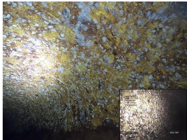
Photo 4-16. Typical severely deteriorated yellowish-white surface of 105-inch pipe with exposed aggregate; S50S511 shown
