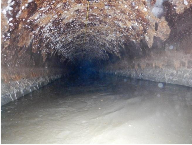
Photo S53 - 1. Downstream pipe, exposed aggregate and discoloration on top portion of pipe.
