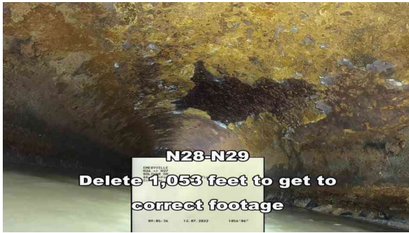
3, 00:00:04, 0.00ft Surface Damage Aggregate Visible from 8 o'clock to 4 o'clock, within 8 inch, Start
