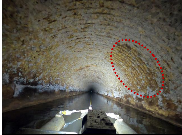
Photo 3-6. Wetness from 1:00 to 3:00 at 317 feet from A39; shelf of soft deteriorated concrete on sides
