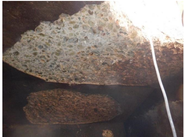
Photo S47 - 4. Delamination exposing aggregate on roof of manhole headspace.
