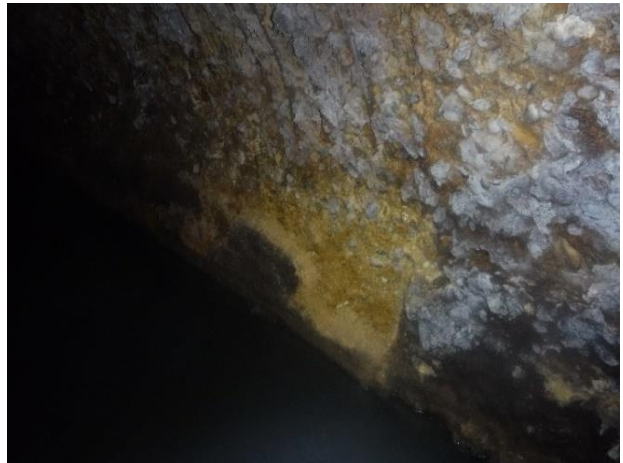
Photo A39 - 4. Delamination in upstream pipe.
