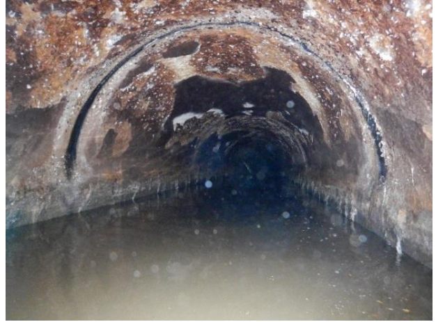
Photo S53 - 2. Upstream pipe, exposed aggregate and discoloration at joint.
