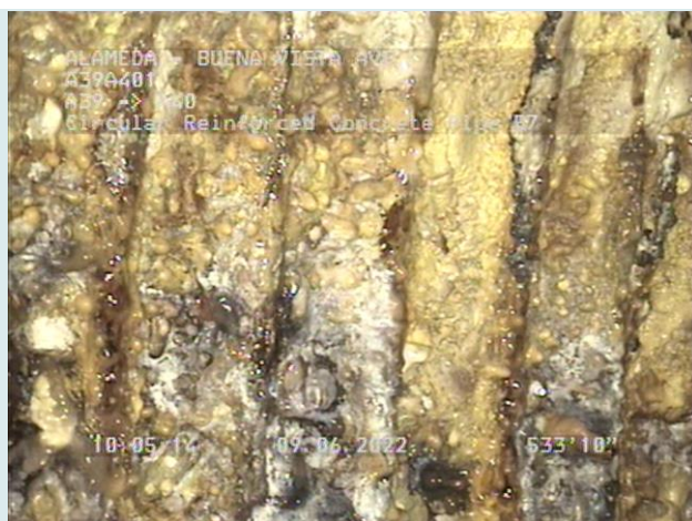
Photo 3-8. Close-up of wetness at 12:00 along possible crack at 533 feet from A39
