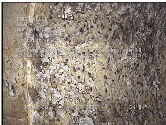
3, 00:07:00, 0.00ft Surface Damage Aggregate Visible from 10 o'clock to 2 o'clock, within 8 inch, Start
