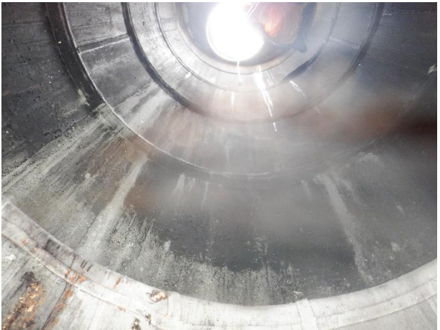
Photo 5-21. MH N35, Liner on upper section of the manhole. Signs of liner failure near top of manhole.
