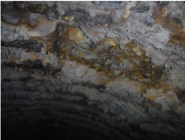
Photo A39 - 3. 12-inch x 9-inch hole at crown of downstream pipe, 2-inches deep.
