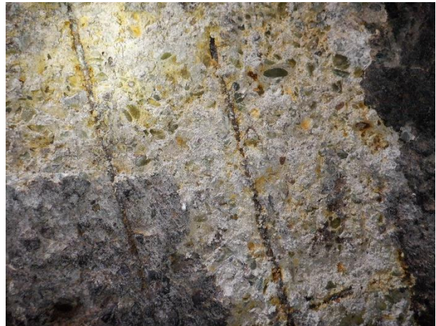
Photo 4-34. MH S15. Loss of concrete mortar and damage to reinforcement on manhole walls.
