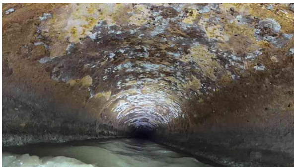
23, 00:15:33, 680.00ft Surface Damage Aggregate Visible from 8 o'clock to 4 o'clock, within 8 inch, Finish
