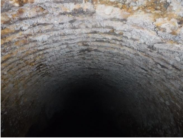
Photo A39 - 1. Downstream pipe, exposed circumferential and longitudinal rebar, exposed rebar and walls are corroded.
