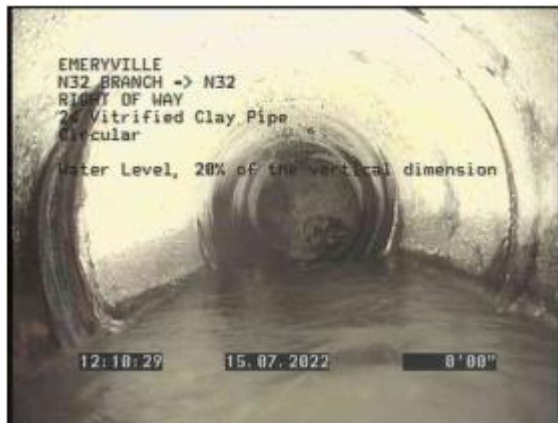
Photo 5-15. 24-inch VCP branch line from unknown EBMUD manhole to N32; pipe stained but in good condition
