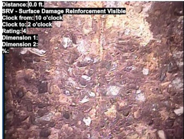
Photo 4-17. Exposed and corroded reinforcing steel from 0 - 10 feet downstream of S47
