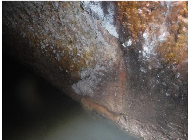
Photo A35 - 4. Broken circumferential rebar in upstream pipe.
