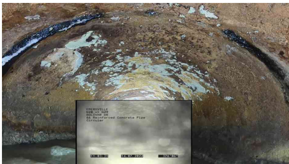
17, 00:08:09, 377.40ft Infiltration Dripper Joint from 1 o'clock to 3 o'clock, within 8 inch
