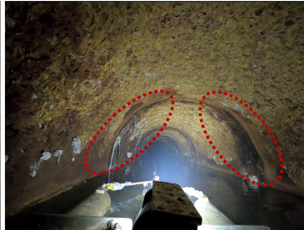
Photo 3-19. Infiltration and encrustation at joint at 454 feet downstream from A45A
