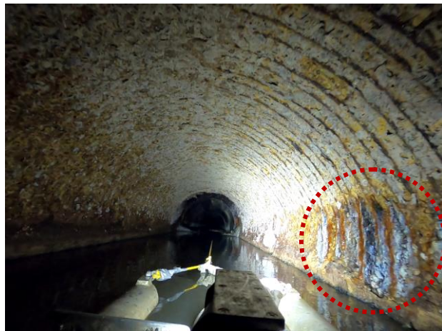
Photo 3-4. Wetness/infiltration at 3:00 at 685 feet from A35
