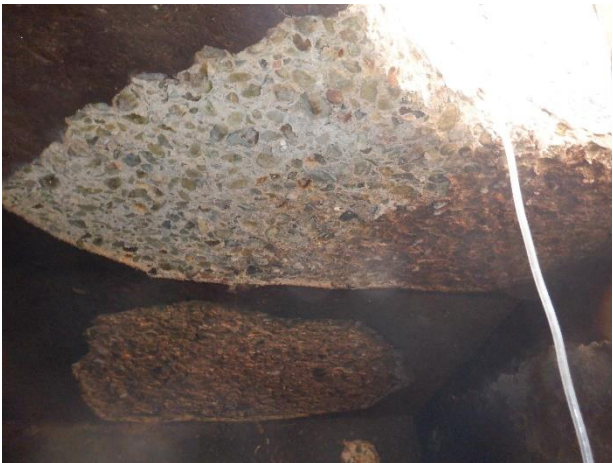
Photo 4-35. MH S47. Spalled concrete and exposed aggregate on manhole ceiling.
