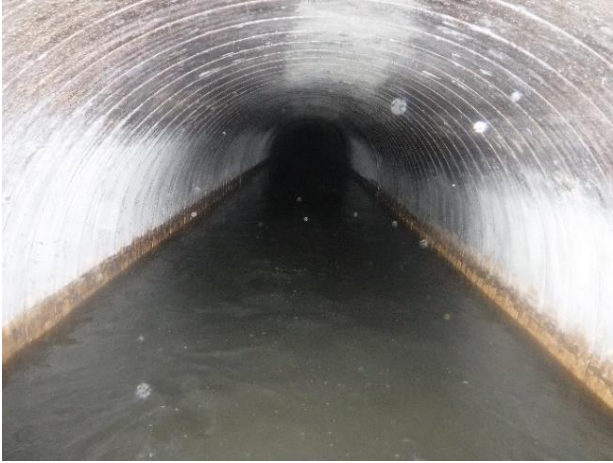
Photo A46A - 1. Downstream pipe, no visible rebar or aggregate.
