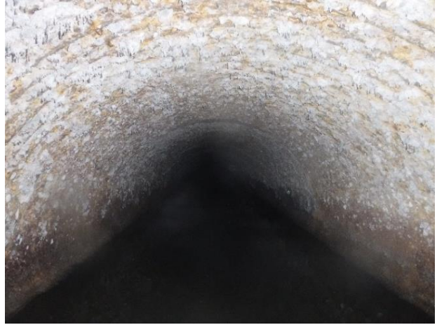
Photo A35 - 2. Upstream pipe, exposed circumferential rebar, exposed rebar is corroded, surface mortar scrapes away easily revealing rebar.
