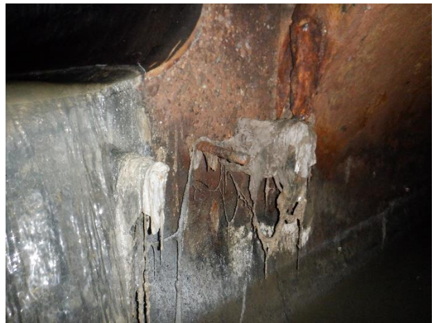
Photo S38 - 4. Exposed rebar protruding from manhole structure wall.
