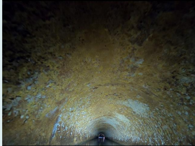
Photo 3-12. Typical area with soft yellow concrete with no exposed reinforcing steel; A34A351 shown
