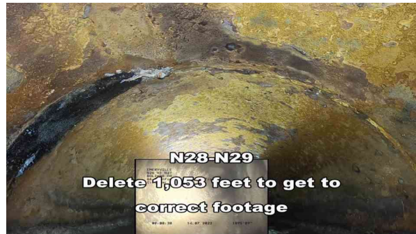
6, 00:03:06, 42.90ft Infiltration Dripper from 9 o'clock to 11 o'clock, within 8 inch
