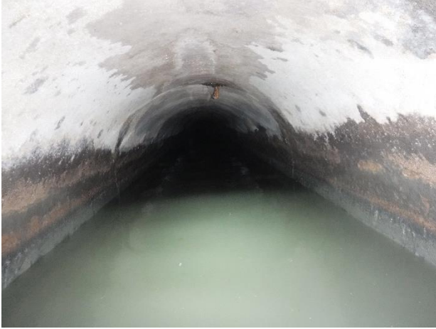
Photo N19-1. Upstream pipe in good condition, minor surface damage on crown of pipe.
