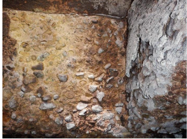
Photo 4-32. MH S48. Moderate surface damage and loss of mortar lining of manhole bench.
