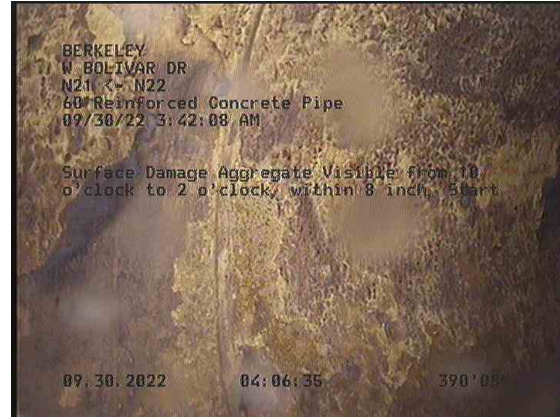
8, 00:16:11, 390.63ft Surface Damage Aggregate Visible from 10 o'clock to 2 o'clock, within 8 inch, Start
