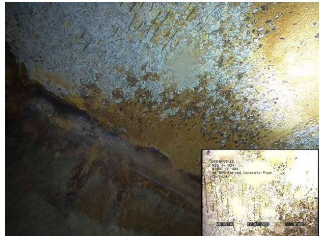
Photo 5-8. VANDA Level 4 condition with exposed reinforcing steel; up to 10 feet upstream from N34
