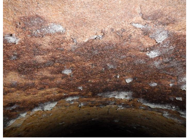
Photo N31 - 4. Downstream pipe, moderate surface damage and delamination of surface mortar lining.
