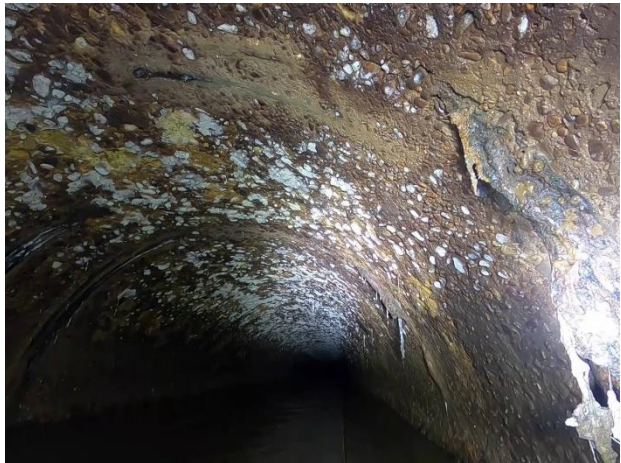
Photo 4-19. Isolated exposed reinforcing steel at 364 feet downstream of S47; near a joint
