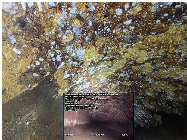
Photo 4-21. Typical severely deteriorated yellowish-white surface of 105-inch pipe with exposed aggregate; S53S541 shown
