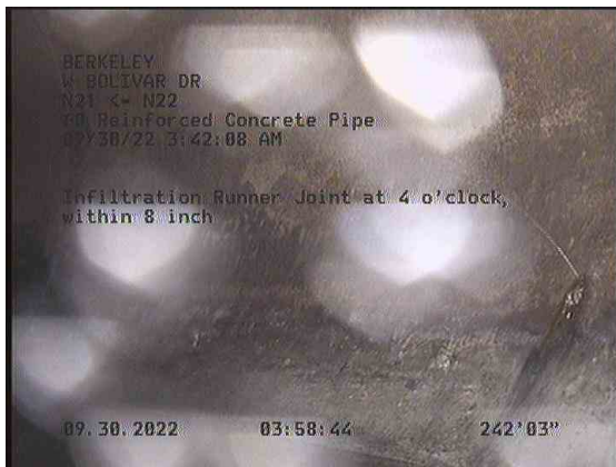
5, 00:08:33, 242.28ft Infiltration Runner Joint at 4 o'clock, within 8 inch
