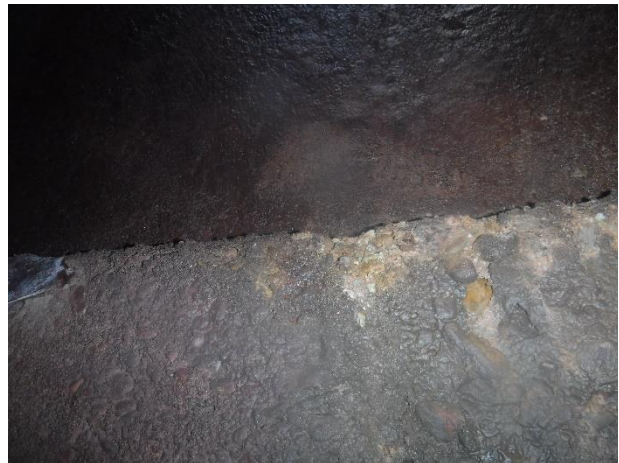
Photo 3-31. MH A37. Unlined concrete with moderate surface damage.
