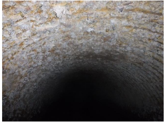
Photo A34 - 2. Upstream pipe, circumferential rebar and aggregate exposed.
