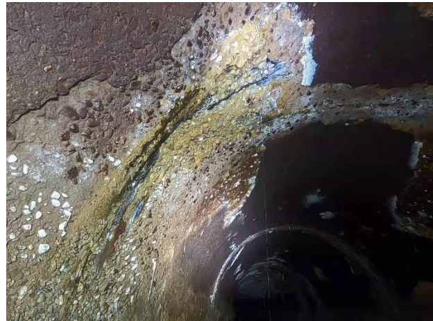
Photo 4-28. Voids with dripping infiltration at 942 feet downstream of S53
