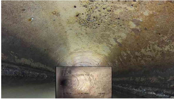
13, 00:23:25, 442.06ft Surface Damage Aggregate Projecting at 12 o'clock
