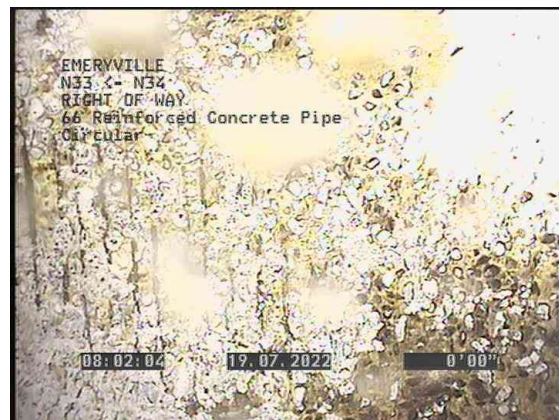
6, 00:01:50, 0.00ft Surface Damage Reinforcement Visible from 10 o'clock to 2 o'clock
