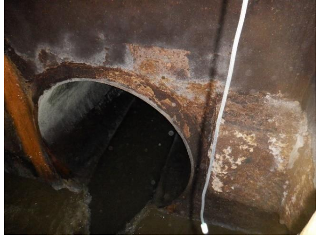
Photo S47 - 2. Side lateral line, surface coating corrosion on pipe bench.
