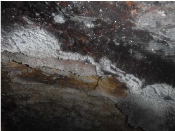
Photo A48 - 3. Damaged coating in upstream pipe, coating missing in areas.
