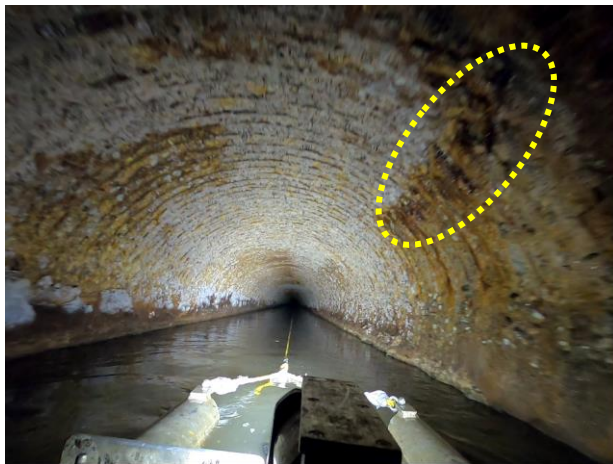
Photo 3-3. Wetness along possible longitudinal crack at 12 feet from A35
