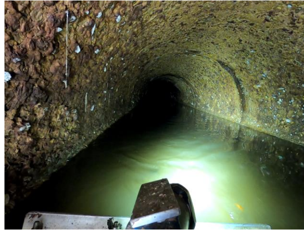
Photo 3-15. Severe surface mortar damage; no reinforcing steel exposed
