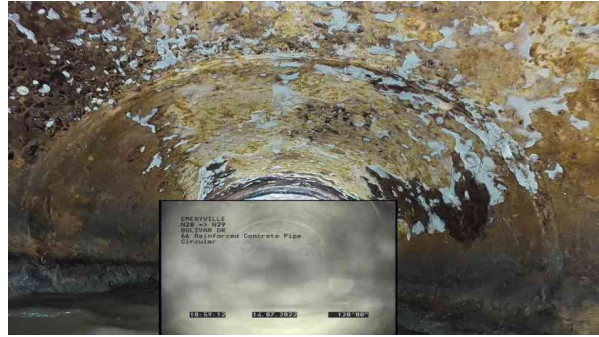
8, 00:03:49, 119.00ft Surface Damage Reinforcement Visible from 11 o'clock to 1 o'clock, within 8 inch, Finish
