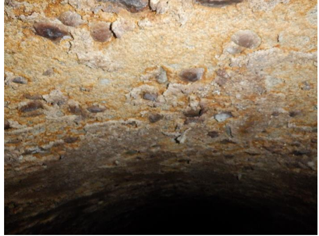
Photo N26 - 4. Downstream pipe, moderate surface damage and delamination of surface mortar lining on crown.
