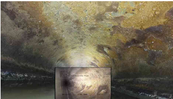
11, 00:21:32, 335.00ft Surface Damage Roughness Increased from 10 o'clock to 2 o'clock, within 8 inch, Finish
