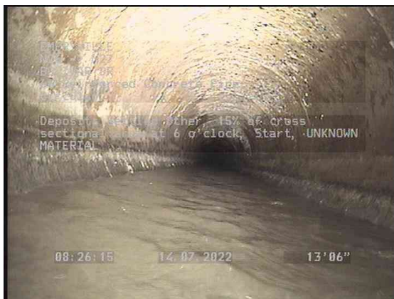
5, 00:04:44, 13.53ft Deposits Settled Other, 15% of cross sectional area at 6 o'clock, Start / UNKNOWN MATERIAL
