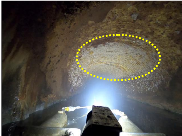
Photo 3-16. Severe surface mortar damage; reinforcing steel exposed just downstream of A46
