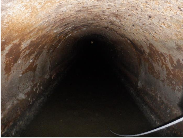
Photo N26 - 3. Downstream pipe, exposed aggregate on crown of pipe.
