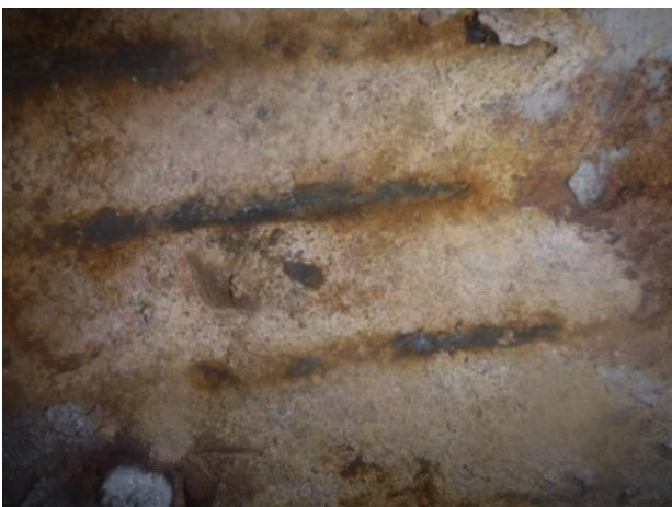
Photo A48 - 5. Exposed rebar in upstream pipe, reinforcement is corroded.
