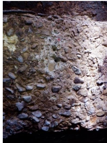
Photo S48 - 4. Exposed aggregate on top of upstream pipe.
