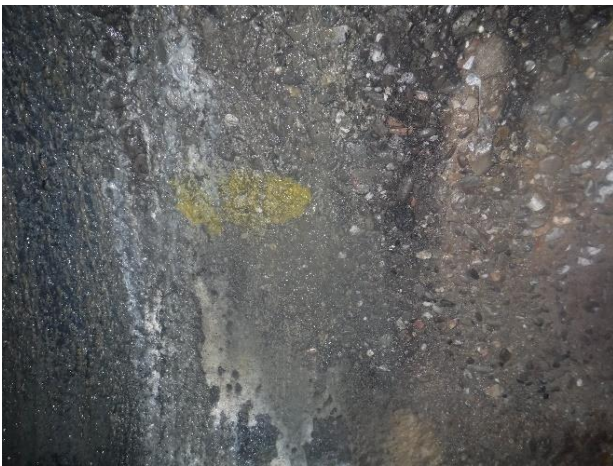
Photo S49 - 3. Wall near manhole dropdown, discoloration, and exposed aggregate.
