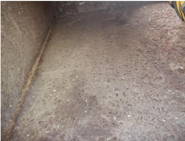
Photo 5-17. MH N26. Minor surface damage on manhole wall.
