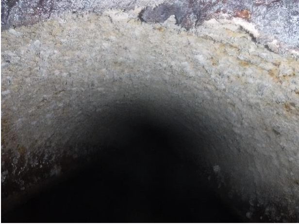
Photo A32 - 1. Downstream pipe, efflorescence and exposed aggregate on walls.
