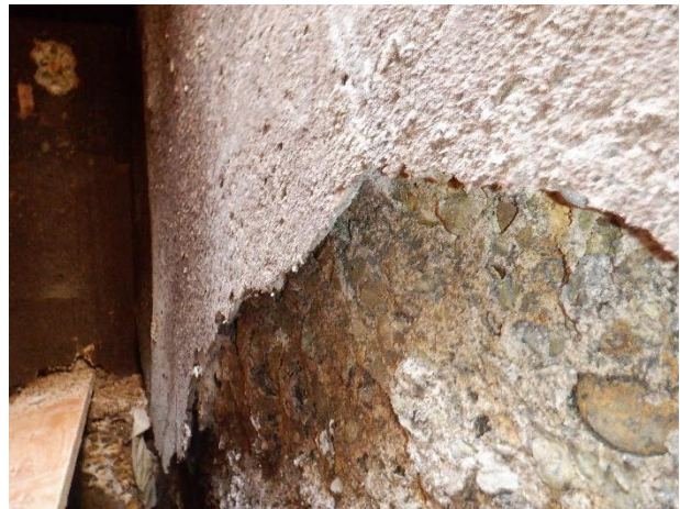
Photo 4-36. MH S47. Spalled concrete and exposed aggregate on manhole wall.
