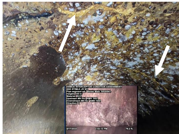
Photo 4-22. Circumferential cracks at 76 feet and 79 feet downstream from S53
