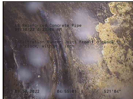
10, 00:26:51, 521.37ft Infiltration Runner Joint from 1 o'clock to 2 o'clock, within 8 inch
