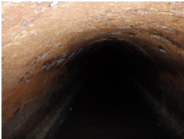
Photo N31 - 1. Upstream pipe, sections of exposed aggregate along crown of pipe.
