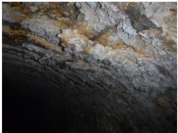
Photo A39 - 6. Exposed circumferential and longitudinal rebar in upstream pipe. Walls and rebar are corroded.
