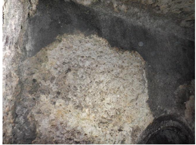
Photo S15 - 2. Bench wall, large spall with exposed aggregate beneath.
