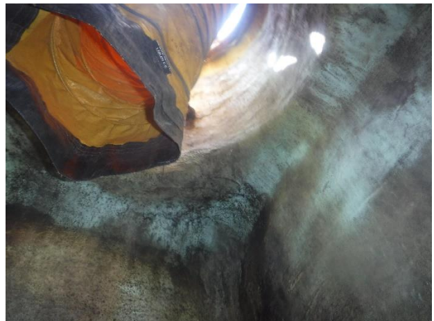
Photo A46A - 6. Green lining on upper section of manhole structure.
