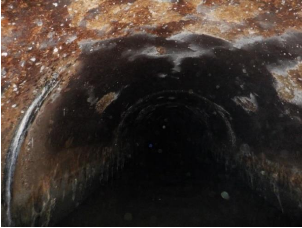
Photo S54 - 1. Downstream pipe, some exposed aggregate and discoloration at joints.
