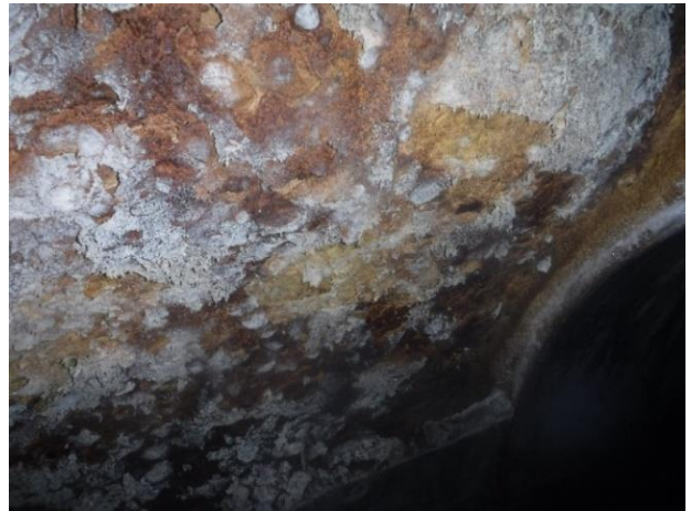
Photo A37 - 4. Exposed aggregate on manhole structure above upstream pipe.
