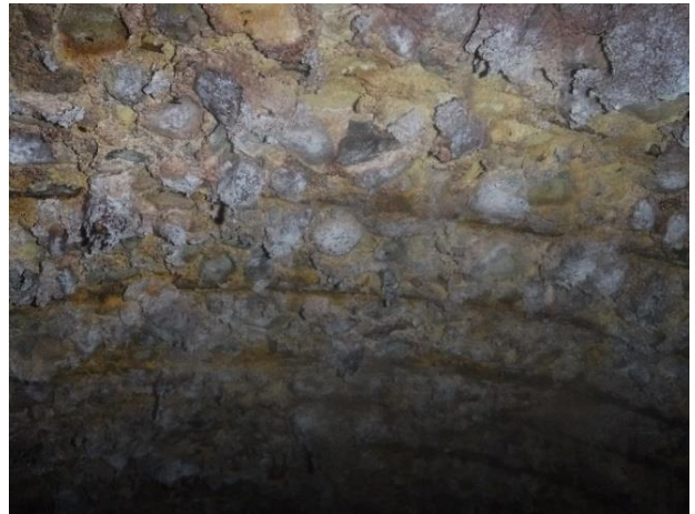
Photo A34 - 4. Exposed circumferential rebar and large aggregate in upstream pipe.
