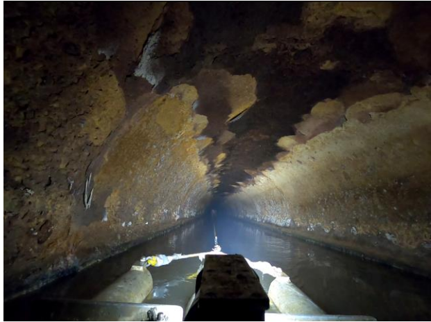
Photo 3-14. Moderate surface damage with outer mortar layer hanging from pipe surface
