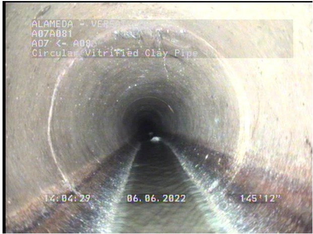
Photo 3-22. Circumferential crack at 145 feet upstream of A08; 1 of 4 within 17-foot span
