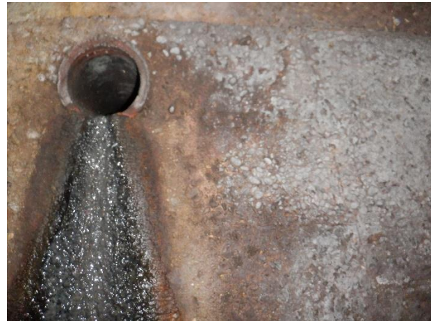
Photo 5-18. MH N26. Minor surface damage on manhole bench near drop inlet.
