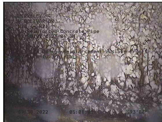
12, 00:32:37, 593.29ft Surface Damage Reinforcement Visible from 1 o'clock to 3 o'clock
