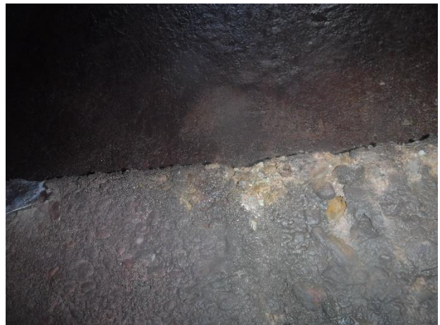
Photo A37 - 6. Soft mushy yellow concrete in manhole structure.
