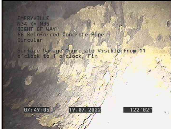
7, 00:05:01, 122.14ft Surface Damage Aggregate Visible from 11 o'clock to 1 o'clock, Finish
