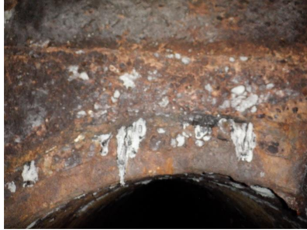
Photo 5-20. MH N31, Minor surface damage on manhole bench above inlet.
