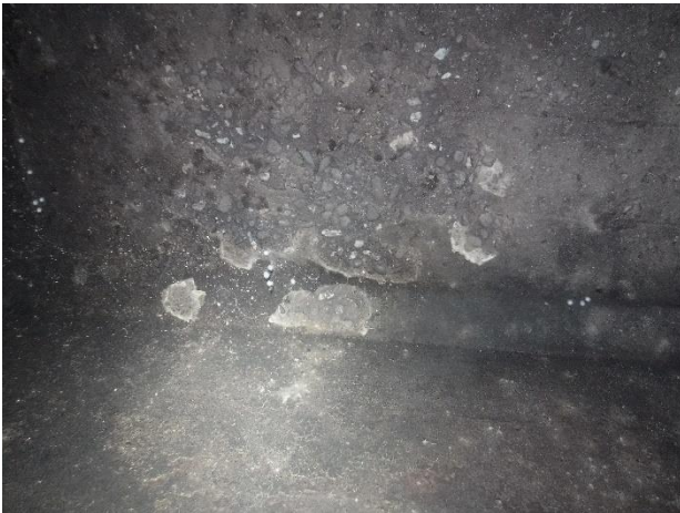
Photo N22-3. Exposed large aggregate on manhole ceiling.
