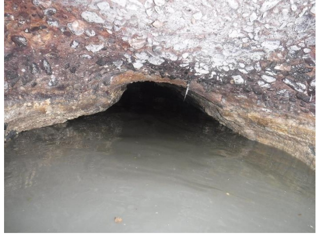
Photo N19-2. Downstream siphon, exposed aggregate on crown and near siphon entrance.
