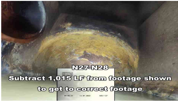
9, 00:00:36, 37.00ft Surface Damage Aggregate Visible from 8 o'clock to 4 o'clock, within 8 inch, Finish
