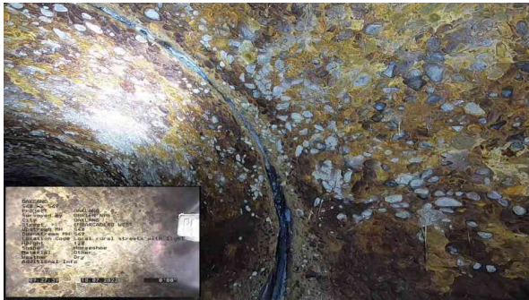
3, 00:00:09, 0.00ft Surface Damage Aggregate Visible from 7 o'clock to 5 o'clock, within 8 inch, Start
