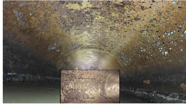
8, 00:14:53, 199.01ft Surface Damage Aggregate Projecting at 2 o'clock
