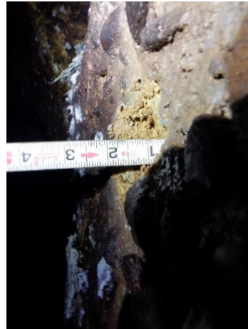
Photo S54 - 4. 2-inch-deep hole in soft mortar.
