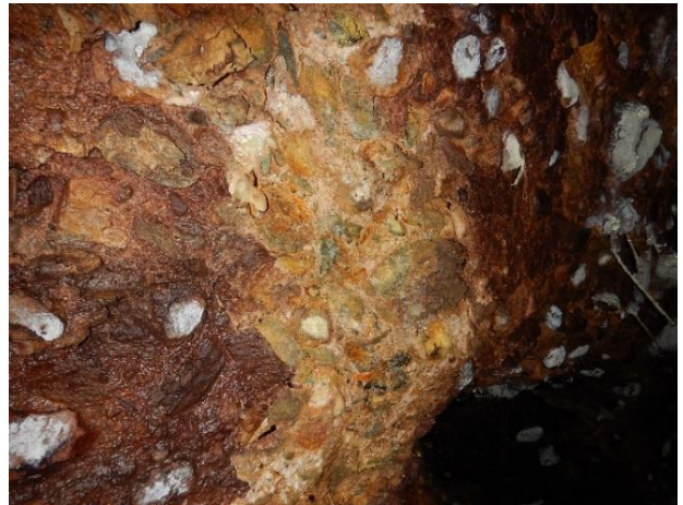
Photo S53 - 4. Exposed aggregate on top of upstream pipe.
