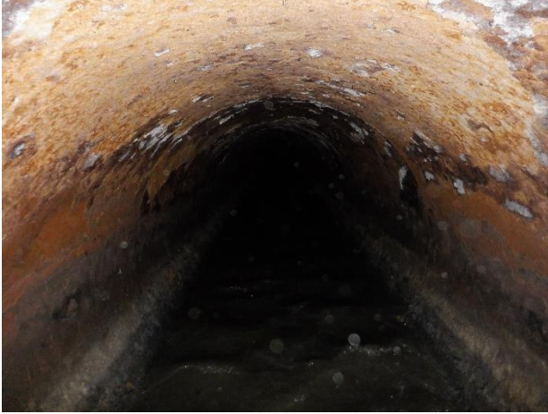
Photo N31 - 3. Downstream pipe, surface damage on crown of pipe.
