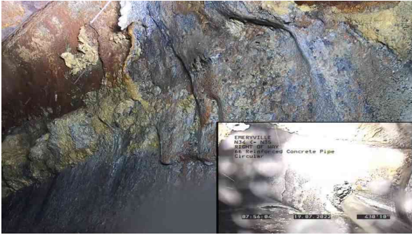
13, 00:12:03, 430.85ft Surface Damage Aggregate Visible from 11 o'clock to 1 o'clock, Finish
