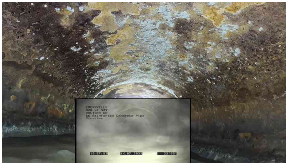
5, 00:02:31, 23.30ft Surface Damage Roughness Increased from 8 o'clock to 4 o'clock, within 8 inch, Finish
