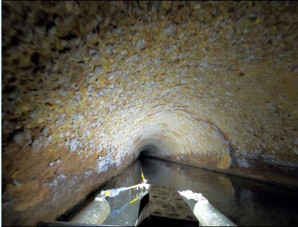
Photo 3-11. Typical area with soft yellow concrete with no exposed reinforcing steel; A32A331 shown
