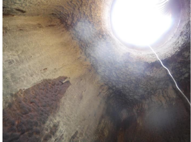
Photo 3-29. MH A32. Upper section of manhole, coating crumbly and in poor condition.
