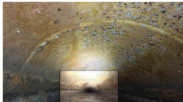
6, 00:05:17, 27.00ft Surface Damage Aggregate Projecting from 11 o'clock to 2 o'clock, within 8 inch, Start / PROJECTING
