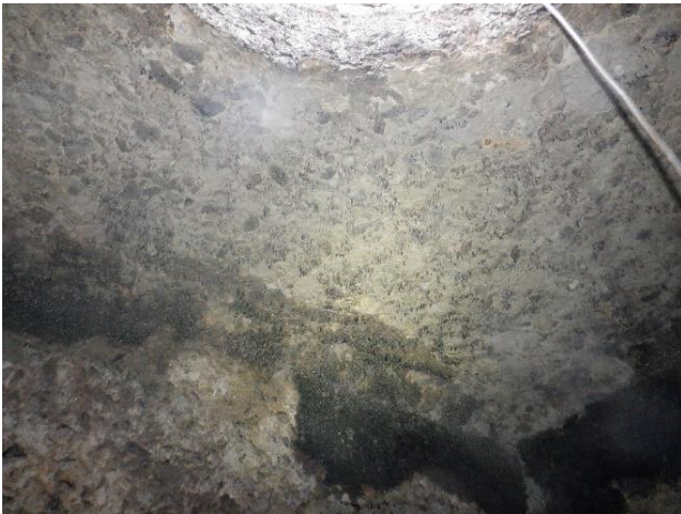
Photo S15 - 3. Roof of the manhole access, large aggregate exposed.
