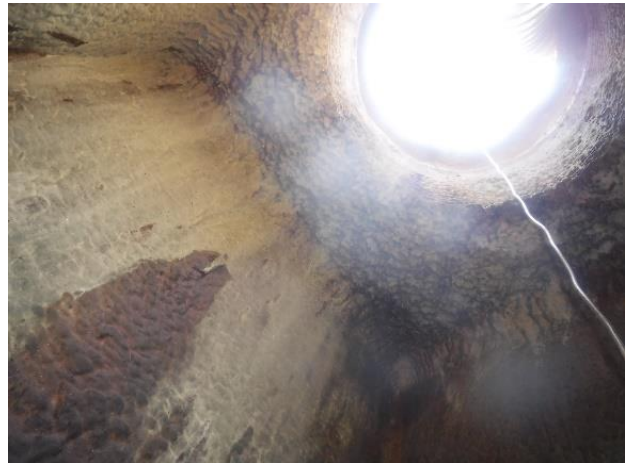
Photo A32 - 4. Efflorescence and discoloration on bench walls.
