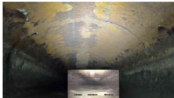
12, 00:26:12, 1066.09ft Deposits Settled Gravel, 30% of cross sectional area at 6 o'clock
