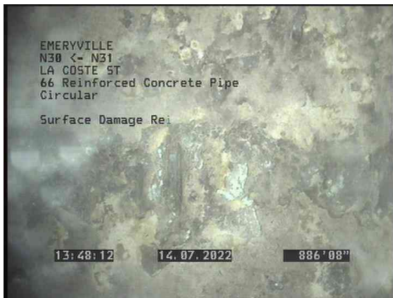
3, 00:24:58, 886.64ft Surface Damage Reinforcement Visible at 12 o'clock
