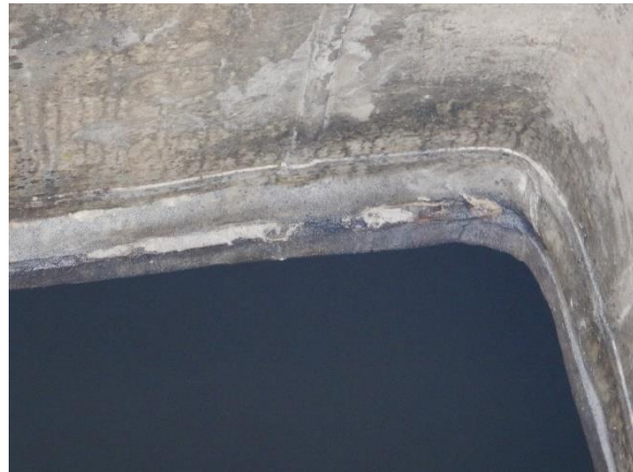
Photo S55 - 2. Lining degradation above inlet pipe.
