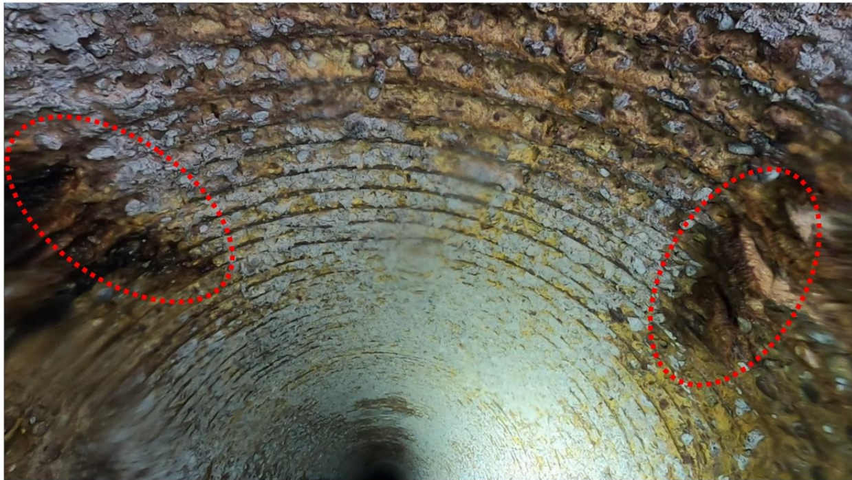
Photo 3-13. Wetness/infiltration/encrustation at 10:00 and 2:00 clock positions at 5 feet downstream from A33; peaks and valleys between circumferential bars
