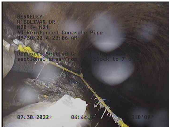
9, 00:17:02, 510.77ft Deposits Settled Gravel, 10% of cross sectional area from 6 o'clock to 7 o'clock
