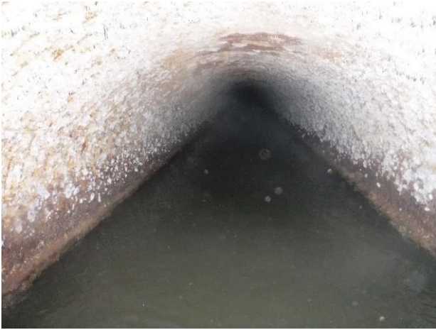
Photo A34 - 1. Downstream pipe, circumferential rebar and aggregate exposed.
