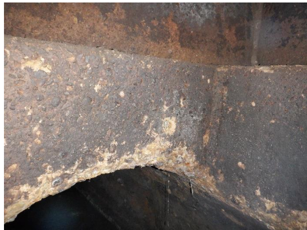
Photo 4-30. MH S16. Minor surface damage on the manhole bench.
