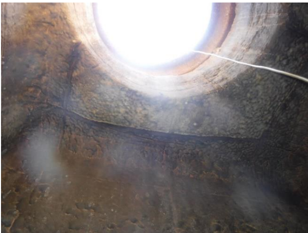
Photo A35 - 5. Bottom of manhole access, exposed rebar is corroded.
