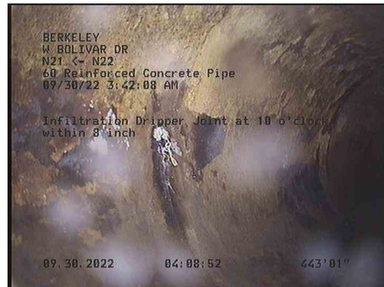
10, 00:18:17, 443.04ft Infiltration Dripper Joint at 10 o'clock, within 8 inch
