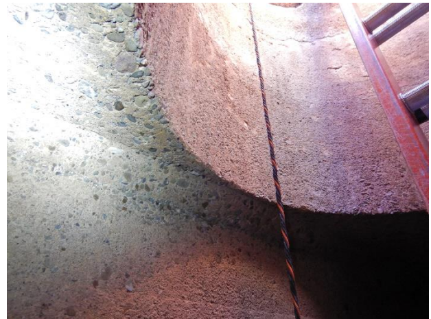
Photo S39 - 6. Exposed aggregate on roof of manhole structure.
