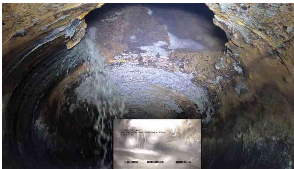
5, 00:01:39, 0.00ft Surface Damage Aggregate Visible from 8 o'clock to 10 o'clock, within 8 inch, Start
