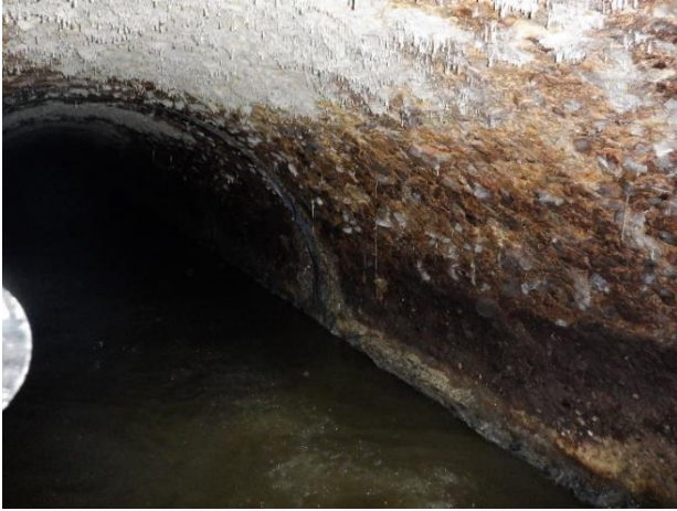
Photo S48 - 1. Downstream pipe, exposed aggregate and soft mushy mortar, mineral deposit on crown of pipe.
