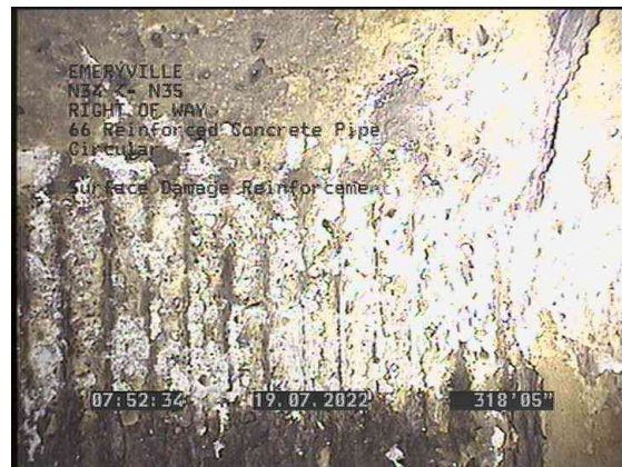
10, 00:08:29, 318.42ft Surface Damage Reinforcement Visible from 11 o'clock to 1 o'clock, within 8 inch, Start
