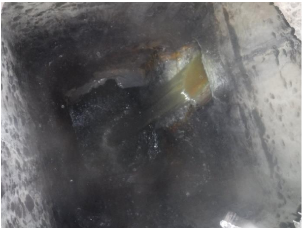
Photo 3-30. MH A40. Upper section of manhole, coating appeared crumbly and in poor condition.
