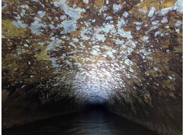
Photo 4-13. Typical severely deteriorated yellowish-white surface of 105-inch pipe with exposed aggregate; S47S481 shown
