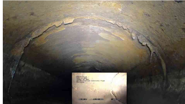
8, 00:15:35, 555.90ft Deposits Attached Other, 5% of cross sectional area from 9 o'clock to 3 o'clock, within 8 inch / UNKNOWN
