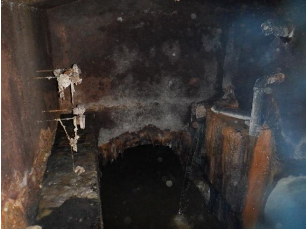
Photo S47 - 1. Downstream pipe and manhole headspace as seen from the top bench
