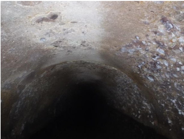
Photo A46A - 3. Crown of upstream pipe, top portion of pipe does not have exposed aggregate.
