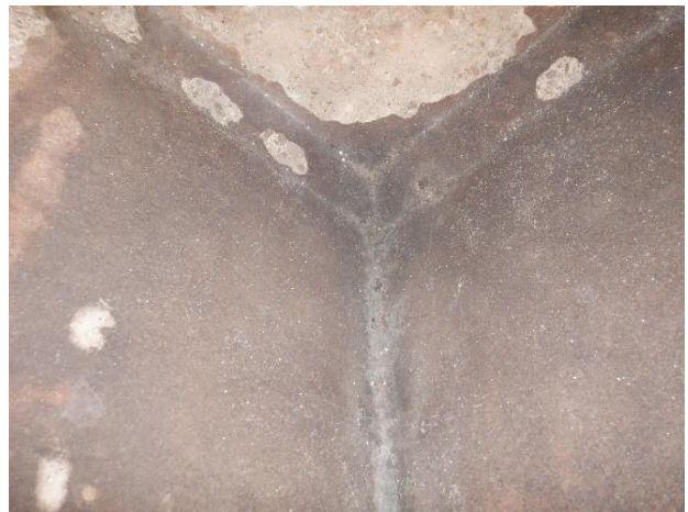
Photo S16 – 4. Bench walls, small spalls exposing aggregate.
