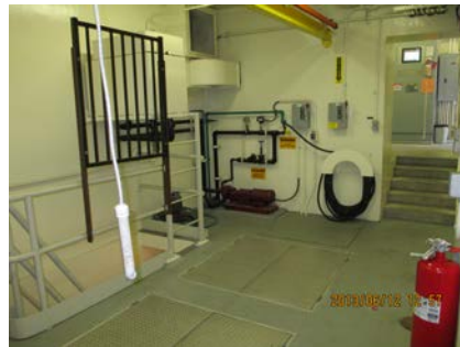
Pump Station B Bldg Photo
