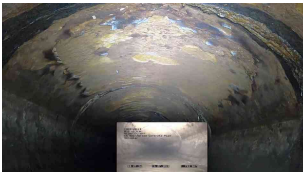
11, 00:19:32, 782.20ft Infiltration Stain Joint from 8 o'clock to 4 o'clock, within 8 inch
