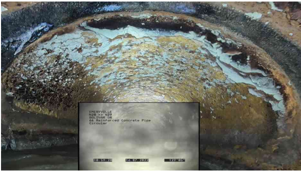
9, 00:03:57, 129.50ft Infiltration Stain from 9 o'clock to 3 o'clock, within 8 inch
