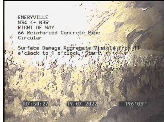
8, 00:06:22, 196.29ft Surface Damage Aggregate Visible from 11 o'clock to 1 o'clock, Start
