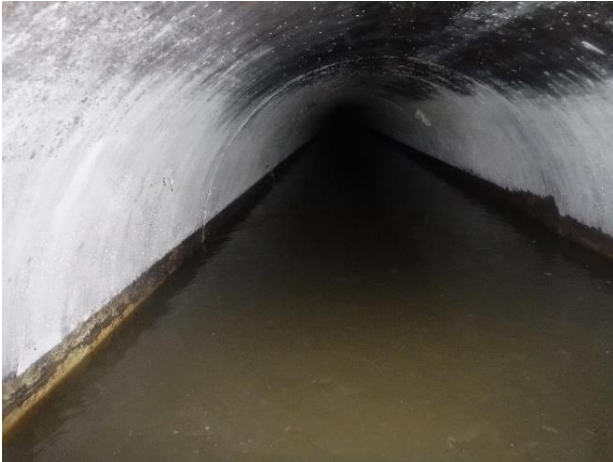
Photo A48 - 1. Downstream pipe, no visible aggregate or reinforcement.
