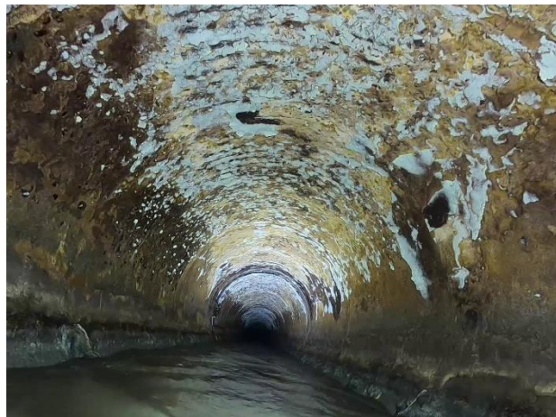
Photo 5-3. VANDA Level 4 condition with exposed reinforcing steel at the crown; 112 to 119 feet downstream from N29
