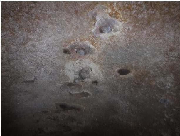
Photo A46A - 5. Pitting on walls of manhole structure.
