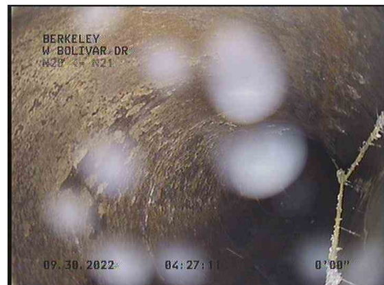
4, 00:01:00, 0.00ft Surface Damage Aggregate Visible from 10 o'clock to 2 o'clock, Start
