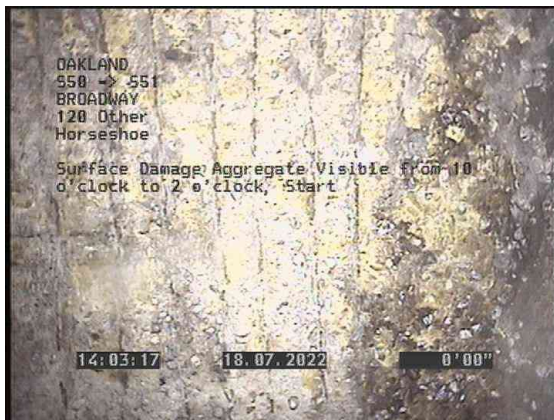
3, 00:00:00, 0.00ft Surface Damage Aggregate Visible from 10 o'clock to 2 o'clock, Start
