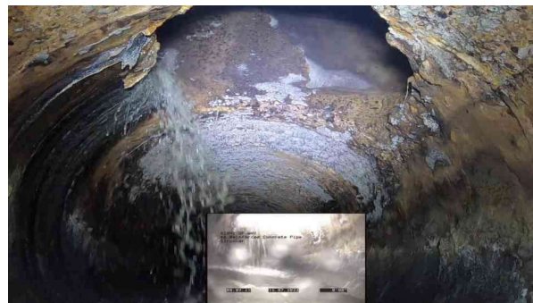
6, 00:01:39, 0.00ft Surface Damage Aggregate Visible from 3 o'clock to 5 o'clock, within 8 inch, Start
