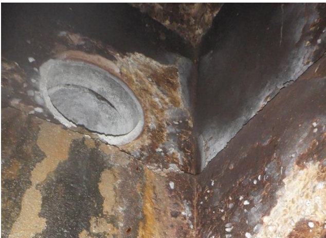
Photo S54 - 5. Exposed aggregate on manhole wall and spalled concrete near drop inlet.
