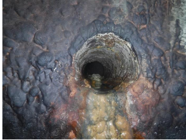
Photo 3-35. MH A32, rough and crumbly lining around manhole inlet.
