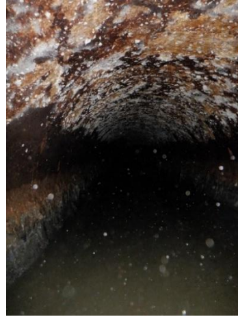
Photo S54 - 2. Upstream pipe, exposed aggregate on crown of pipe.
