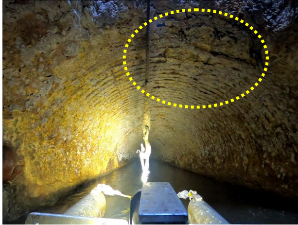
Photo 3-5. Missing circumferential bars at A39; longitudinal bars also exposed
