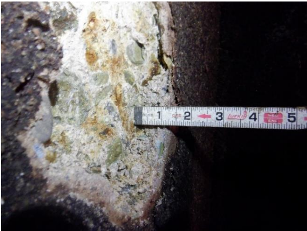
Photo S47 - 3. Spall on west wall, aggregate exposed beneath delamination.
