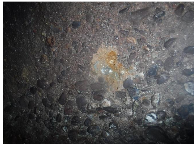
Photo S49 - 4. Wall penetration with discolored soft mortar exposed.
