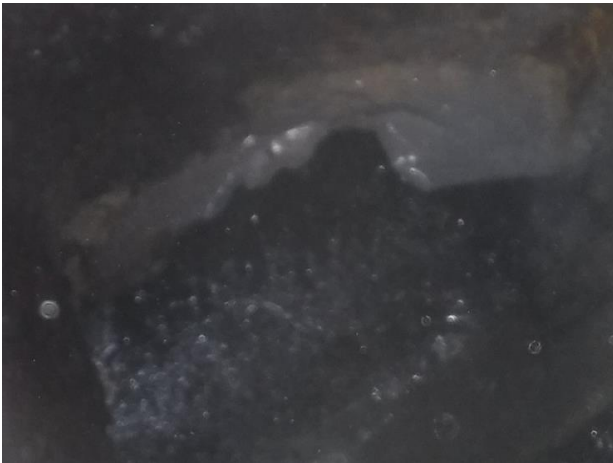
Photo A40 -3. Upstream pipe, loss of concrete on crown of pipe.
