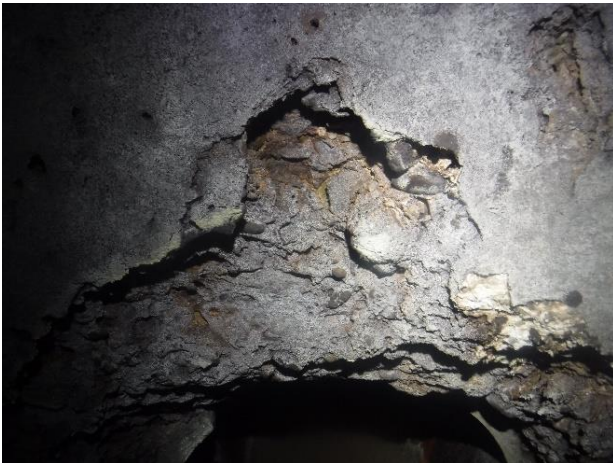
Photo S51 - 3. Wall deterioration on upper bench.
