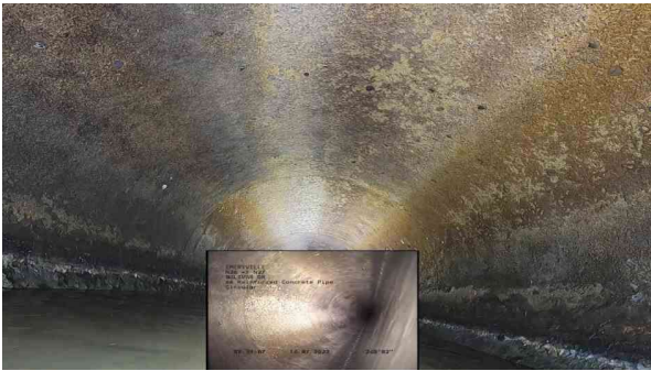
9, 00:17:42, 248.19ft Surface Damage Aggregate Visible from 10 o'clock to 2 o'clock, within 8 inch, Finish
