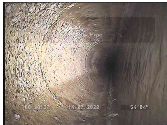
4, 00:07:00, 0.00ft Surface Damage Aggregate Visible from 10 o'clock to 2 o'clock, within 8 inch, Start
