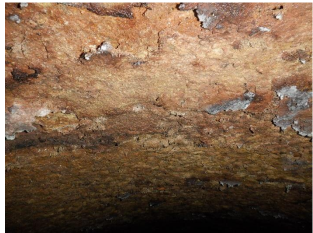
Photo N31 - 2. Upstream pipe, moderate surface damage and delamination of surface mortar lining.
