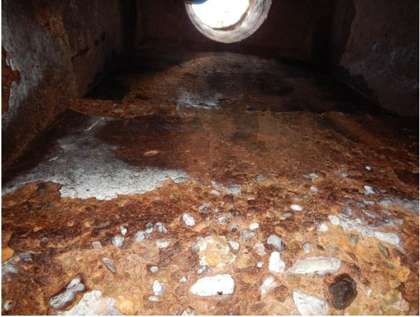
Photo 4-31. MH S53. Moderate surface damage and loss of mortar lining of bench.
