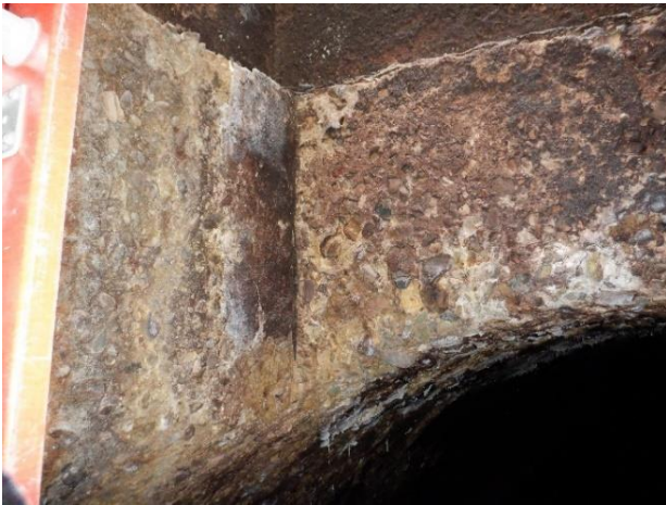
Photo S48 - 3. Top bench of downstream pipe, corroded and some exposed aggregate.
