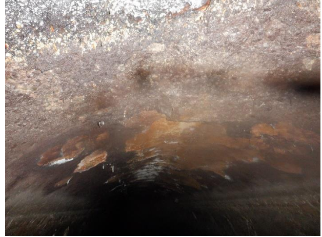
Photo N35 - 2. Upstream pipe, moderate surface damage and delamination of surface mortar lining.
