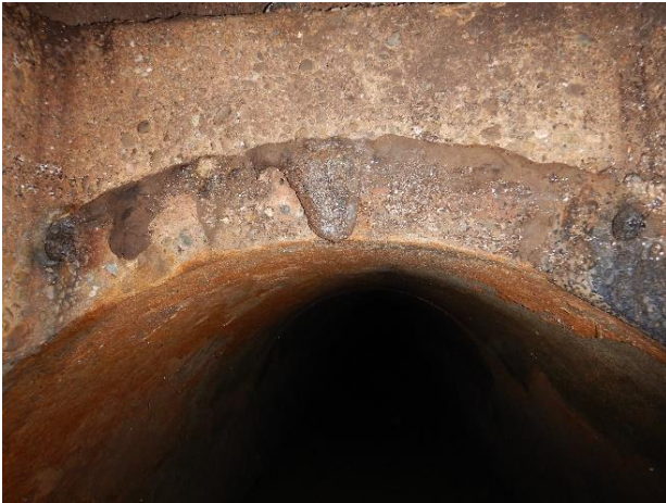
Photo S14 - 3. Downstream pipe and manhole headspace as seen from the top bench.
