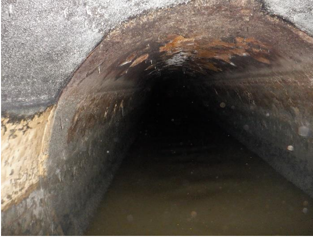
Photo N35 - 1. Upstream pipe, surface damage along crown of pipe.
