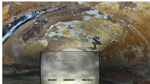
18, 00:08:21, 390.60ft Infiltration Stain from 9 o'clock to 12 o'clock, within 8 inch
