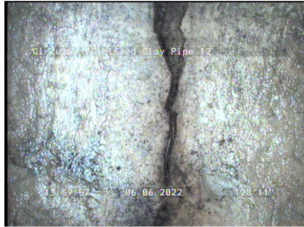
Photo 3-23. Crack with void and soil visible at 128 feet upstream of A08
