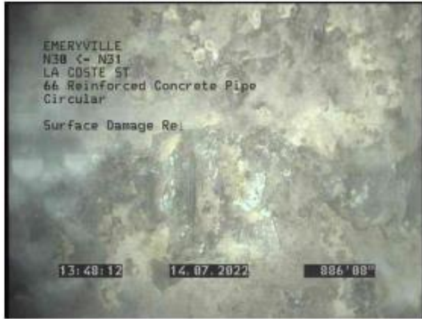
Photo 5-5. VANDA Level 4 condition with exposed reinforcing steel; 887 feet upstream from N31
