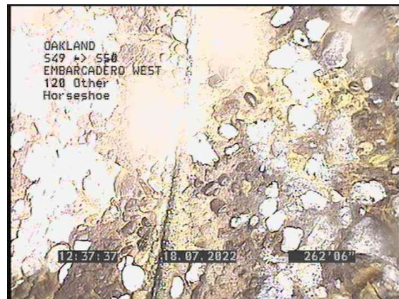
4, 00:07:13, 262.52ft Infiltration Dripper at 12 o'clock, within 8 inch
