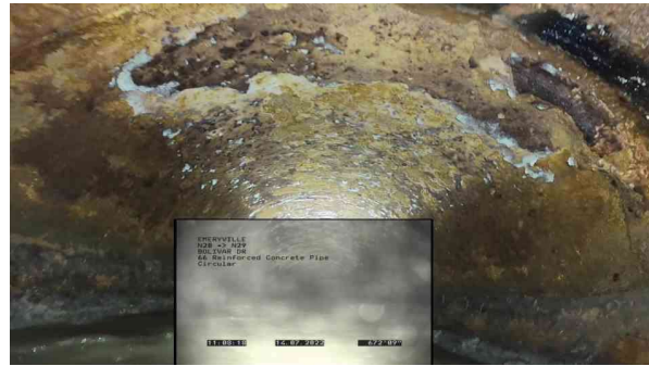
22, 00:12:55, 672.90ft Infiltration Stain from 1 o'clock to 2 o'clock, within 8 inch
