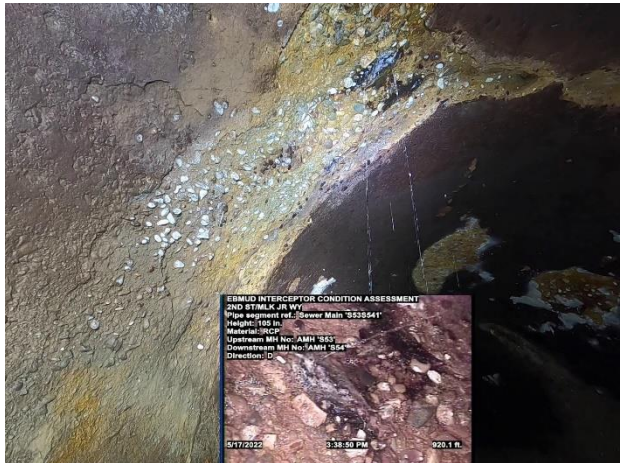
Photo 4-27. Voids with dripping infiltration at 920 feet downstream of S53
