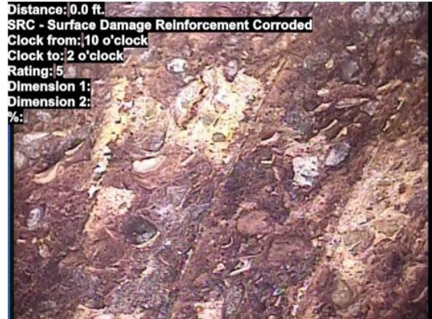
Photo 4-18. Exposed and corroded reinforcing steel from 0 - 10 feet downstream of S47
