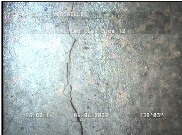
Photo 3-24. Crack at 138 feet upstream of A08
