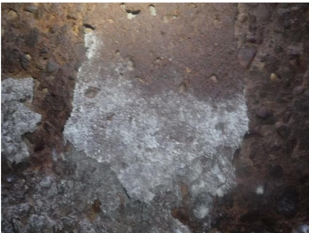
Photo A37 - 5. Concrete spalling on manhole structure wall.
