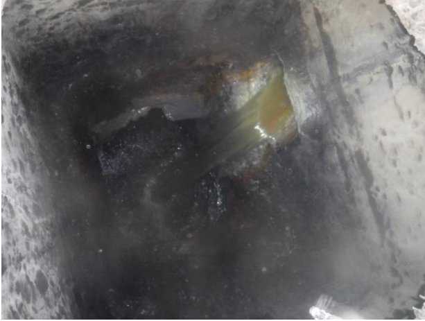
Photo A40 -1. Manhole, discoloration, and degradation observed on walls.
