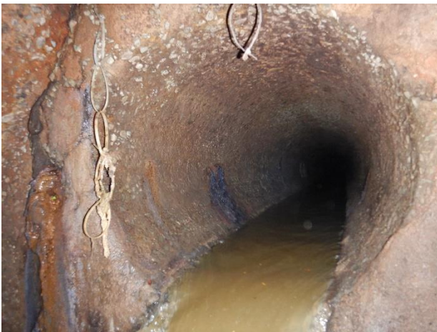
Photo S39 - 3. Large side lateral line.
