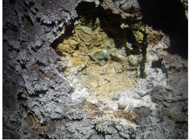
Photo S51 - 2. Large crater in wall exposing yellow surface mortar and aggregate.
