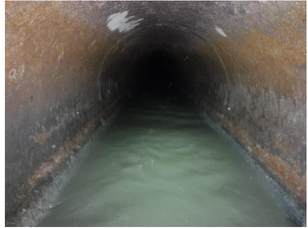
Photo N22-2. Downstream pipe, surface damage and delamination of surface mortar lining.
