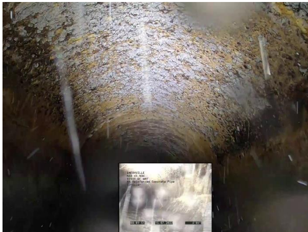
Photo 5-7. VANDA Level 4 condition with exposed reinforcing steel; up to 10 feet downstream from N33
