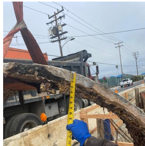
Photo 4-4. Piece of RCP removed from just downstream of S15; approx. 2 inches of wall remained
