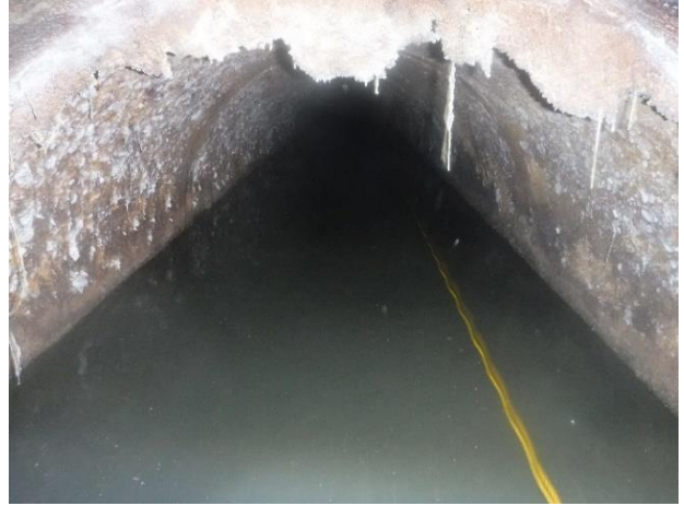
Photo A46A - 2. Upstream pipe, lining is sagging into pipe and aggregate is exposed.
