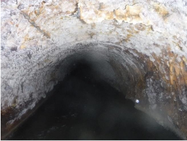
Photo A35 - 1. Downstream pipe, exposed circumferential and longitudinal rebar, rebar is corroded, remaining mortar is soft and mushy.
