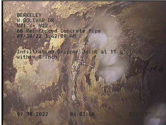
7, 00:13:41, 322.81ft Infiltration Dripper Joint at 11 o'clock, within 8 inch
