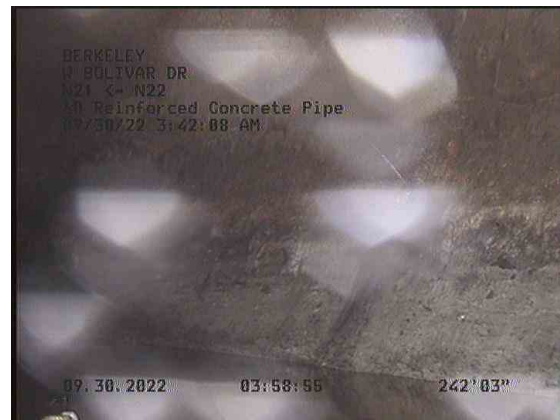
6, 00:08:33, 242.28ft Infiltration Runner Joint at 4 o'clock, within 8 inch
