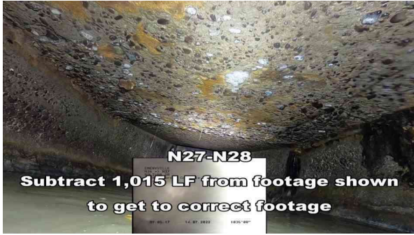
7, 00:00:23, 19.00ft Infiltration Stain from 1 o'clock to 3 o'clock
