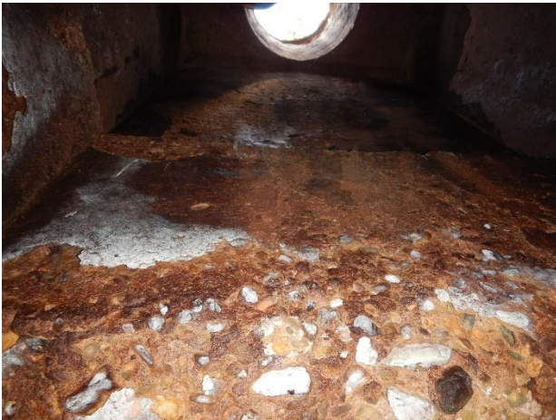
Photo S53 - 3. Exposed aggregate on manhole walls and ceiling.
