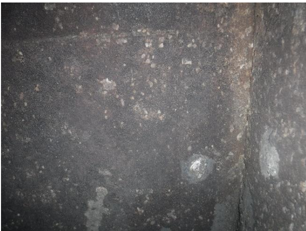
Photo S50 - 3. Walls near manhole opening, multiple small pits and craters.
