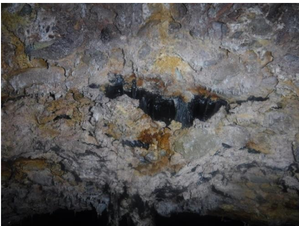
Photo A39 - 5. Crack above downstream pipe, black tar inside crack.
