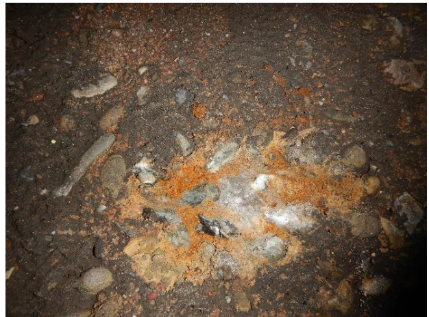
Photo S14 - 6. Exposed aggregate on manhole structure wall, \frac{3}{4} " deep.
