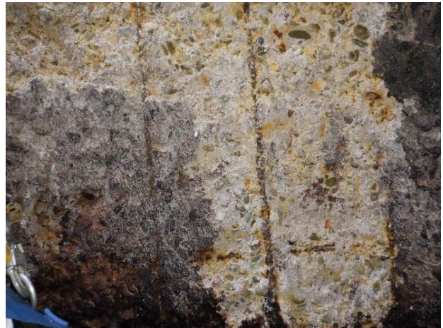
Photo S15 - 4. Bench wall, corroded reinforcement partially exposed.
