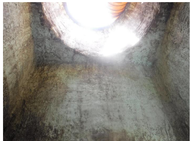
Photo A47 - 6. Green discoloration on upper manhole structure.
