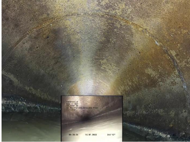
Photo 5-11. Typical VANDA Level 2 condition with minor surface damage; N26N271 shown
