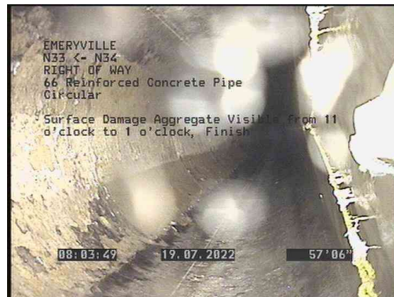
10, 00:03:45, 57.51ft Surface Damage Aggregate Visible from 11 o'clock to 1 o'clock, Finish
