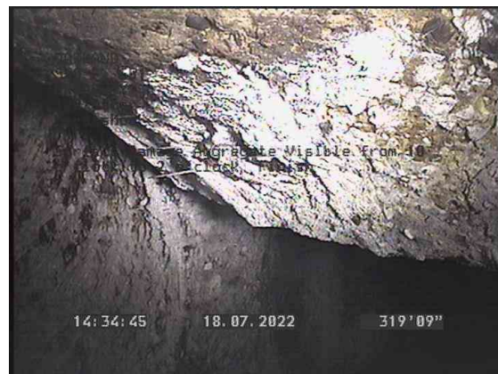
6, 00:33:13, 319.73ft Surface Damage Aggregate Visible from 10 o'clock to 2 o'clock, Finish
