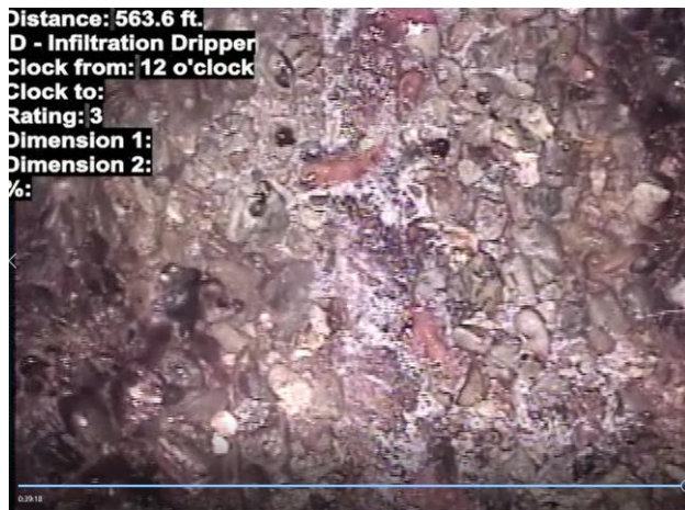
Photo 4-3. Wetness/dripping infiltration through pipe at crown just downstream of S15
