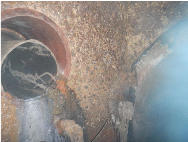
Photo S38 - 5. Exposed aggregate on manhole structure wall above upstream pipe opening.
