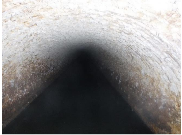
Photo A39 - 2. Upstream pipe exposed circumferential rebar and aggregate. Concrete is soft and scrapes away easily revealing rebar.
