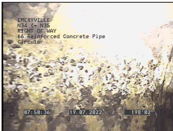
9, 00:06:22, 196.29ft Surface Damage Aggregate Visible from 11 o'clock to 1 o'clock, Start
