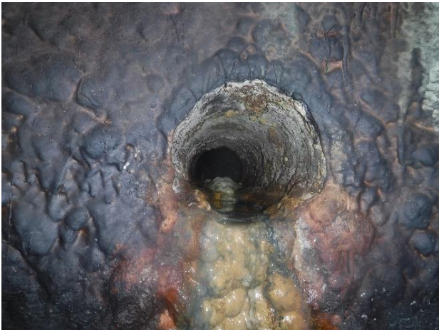
Photo A32 - 3. Side lateral pipe, showing signs of coating damage.
