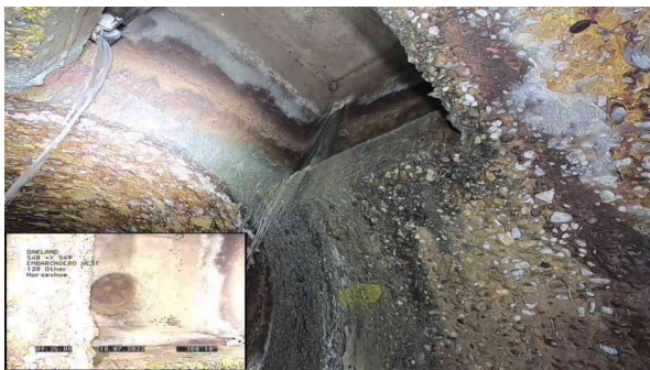
5, 00:07:37, 380.00ft Surface Damage Aggregate Visible from 7 o'clock to 5 o'clock, within 8 inch, Finish
