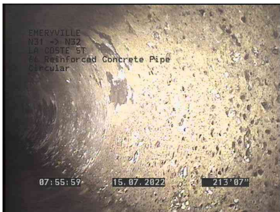
5, 00:07:06, 213.62ft Surface Damage Aggregate Visible from 11 o'clock to 1 o'clock, within 8 inch, Start
