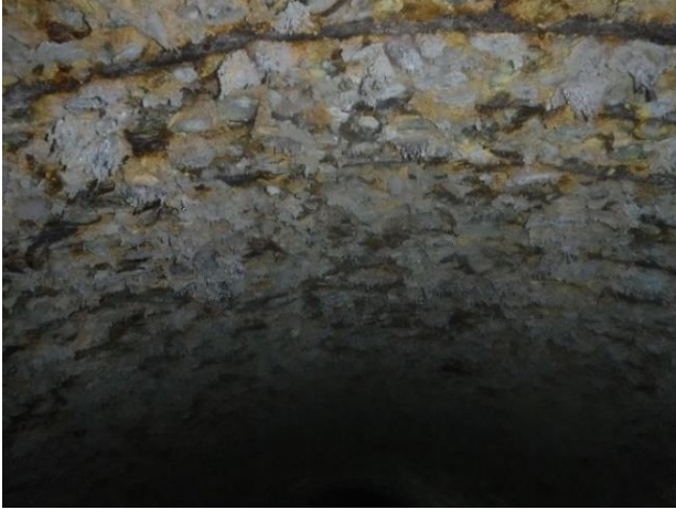
Photo A37 - 1. Downstream pipe, exposed circumferential rebar and aggregate.
