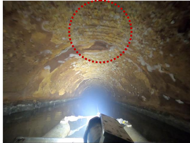
Photo 3-17. Severe surface mortar damage; reinforcing steel exposed downstream of A47
