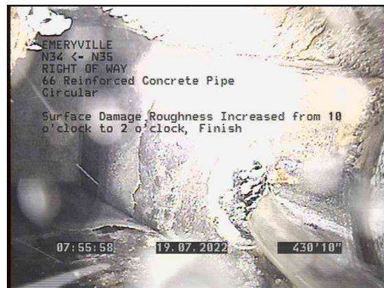
12, 00:11:53, 430.75ft Surface Damage Roughness Increased from 10 o'clock to 2 o'clock, Finish
