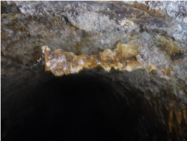
Photo A35 - 3. Rebar sagging into pipe headspace at crown of downstream pipe.
