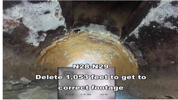
8, 00:09:36, 181.00ft Surface Damage Aggregate Visible from 8 o'clock to 4 o'clock, within 8 inch, Finish
