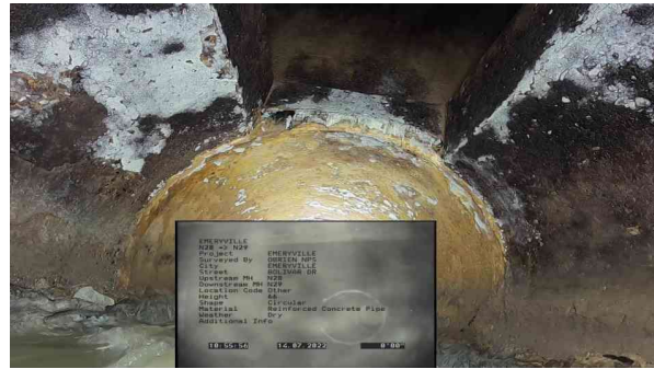
4, 00:00:34, 0.00ft Surface Damage Roughness Increased from 8 o'clock to 4 o'clock, within 8 inch, Start
