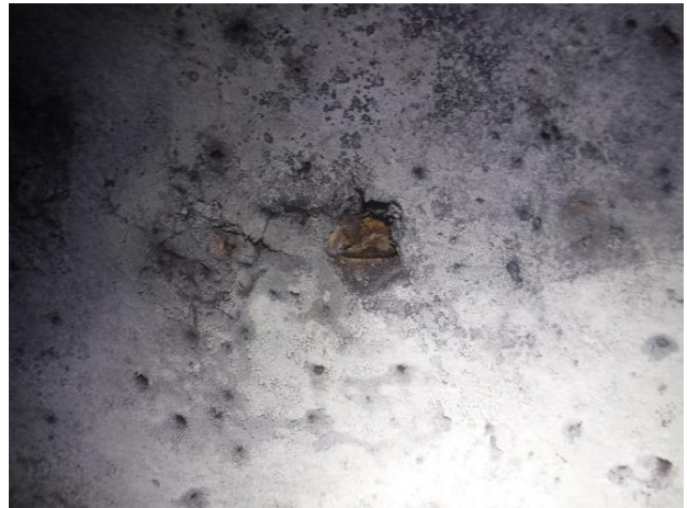
Photo S51 - 4. Exposed corroded rebar in crater in upper bench.
