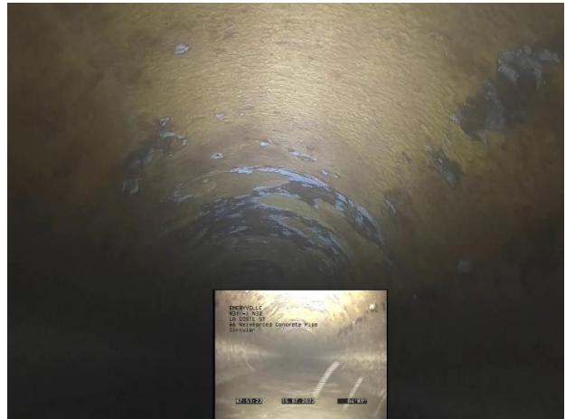
Photo 5-14. Typical VANDA Level 2 condition with minor surface damage; N34N351 shown
