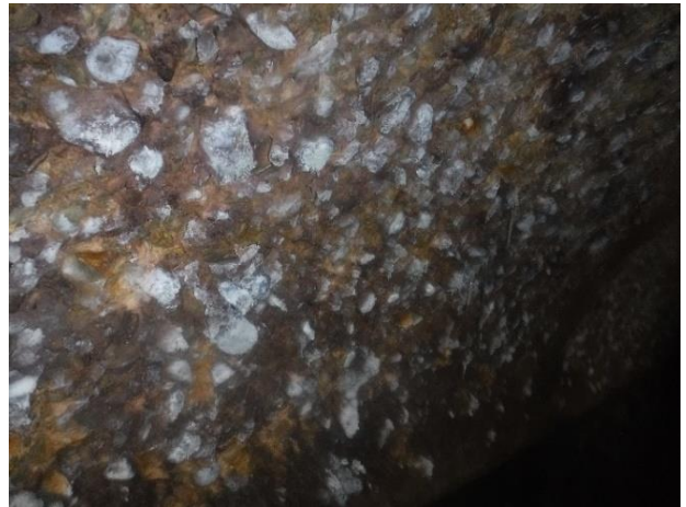
Photo A46A - 4. Detail of exposed aggregate in upstream pipe.
