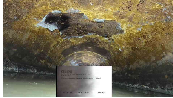
14, 00:39:37, 894.80ft Infiltration Stain Barrel at 11 o'clock
