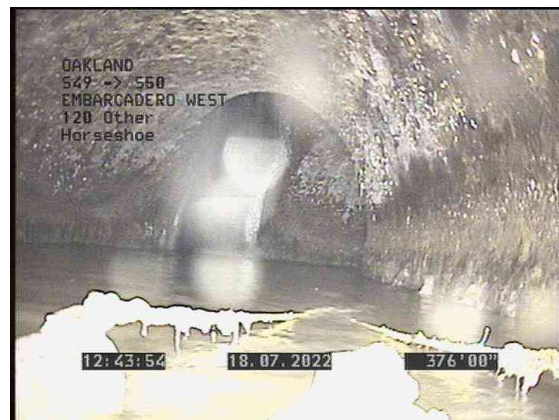
6, 00:13:24, 376.04ft Miscellaneous Survey Abandoned / PARACHUTE GOT STUCK AT BEND. CAMERA WILL NOT TRAVEL ANY
