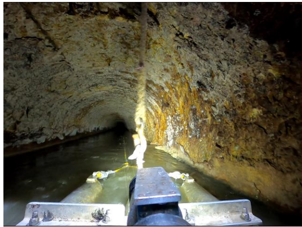
Photo 3-2. Missing circumferential reinforcing steel bars downstream of manhole A35
