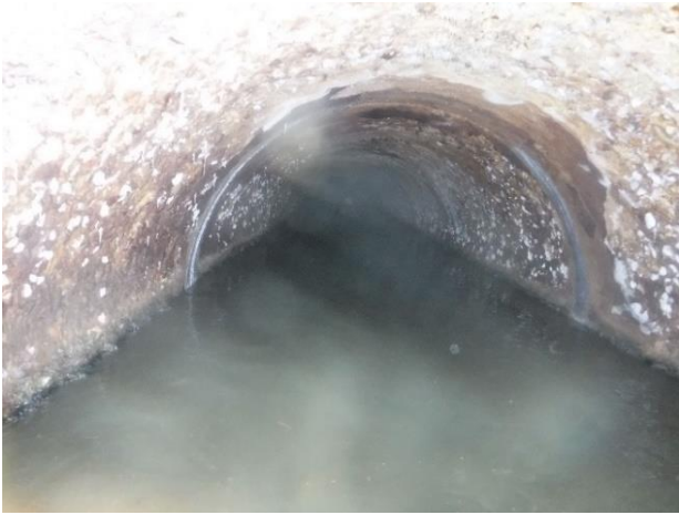
Photo A47 - 1. Downstream pipe, exposed aggregate and discoloration at joints.
