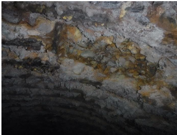
Photo 3-1. Missing/broken circumferential reinforcing steel bars just downstream of A39
