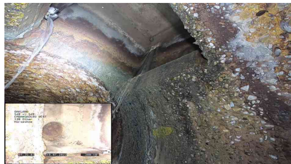
6, 00:07:33, 380.10ft Surface Damage Aggregate Projecting from 11 o'clock to 1 o'clock, within 8 inch, Finish
