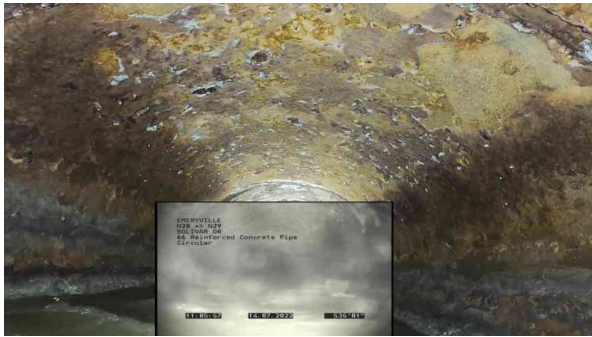
21, 00:10:34, 534.90ft Surface Damage Reinforcement Visible from 12 o'clock to 3 o'clock, within 8 inch, Finish
