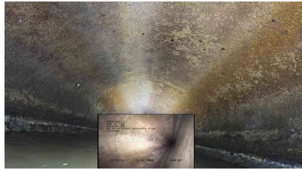
10, 00:18:17, 248.19ft Surface Damage Roughness Increased from 10 o'clock to 2 o'clock, within 8 inch, Start
