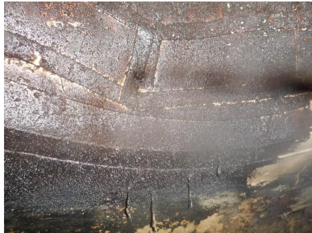
Photo 5-22. MH N35, Liner on lower section of manhole in good condition, black discoloration.
