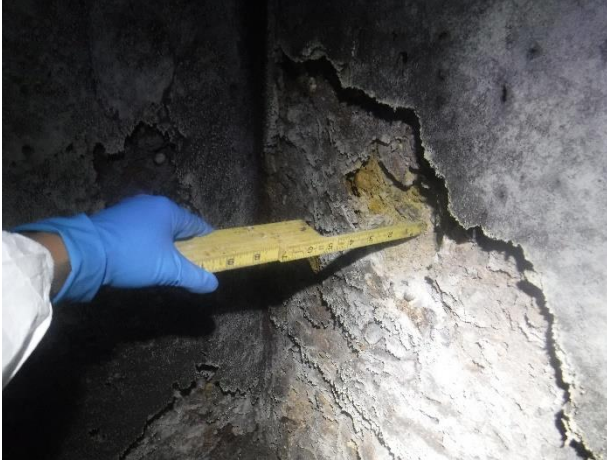
Photo 4-37. MH S51. Spalled concrete and exposed on manhole ceiling.
