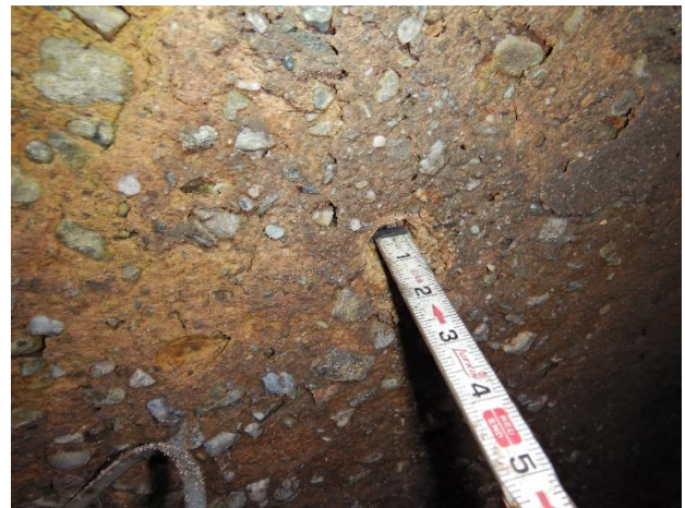
Photo S39 - 4. Exposed aggregate and pit on manhole structure wall.
