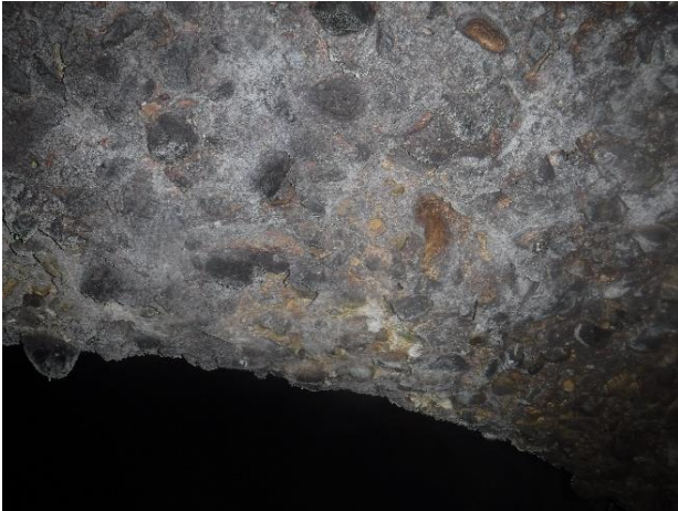
Photo S50 - 1. Large aggregate exposed on crown of downstream pipe.
