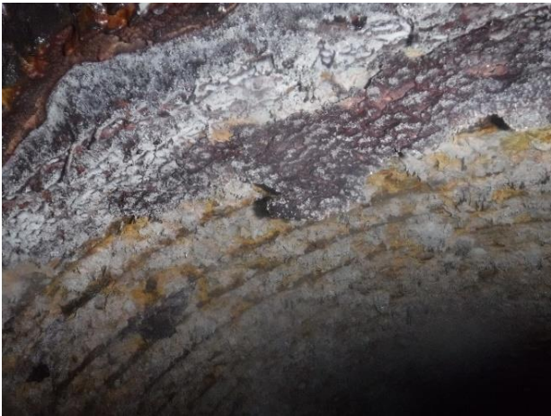
Photo A34 - 3. Coating damage and exposed circumferential rebar in downstream pipe.
