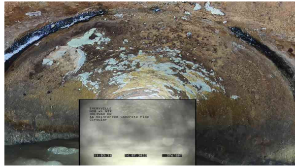
16, 00:08:09, 377.40ft Infiltration Dripper Joint from 9 o'clock to 12 o'clock, within 8 inch
