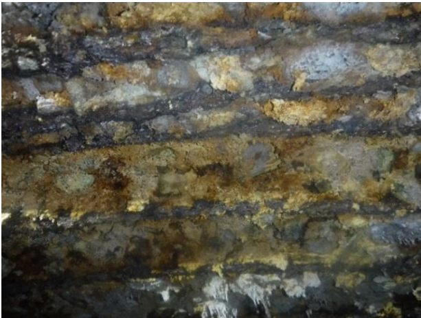
Photo A37 - 3. Exposed and corroded circumferential rebar in downstream pipe.
