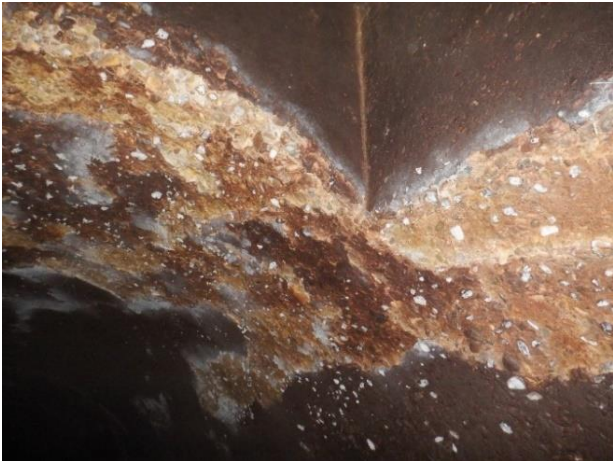
Photo S54 - 3. Exposed aggregate and wall corrosion on bench at downstream pipe opening.
