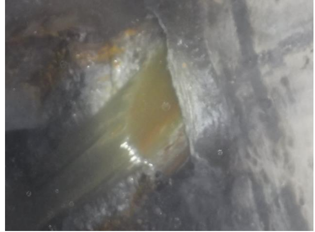
Photo A40 -2. Drop inlet, surface damage on crown and 6:00 of pipe.
