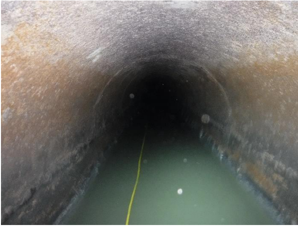
Photo N22-1. Upstream pipe, surface damage along crown of pipe.
