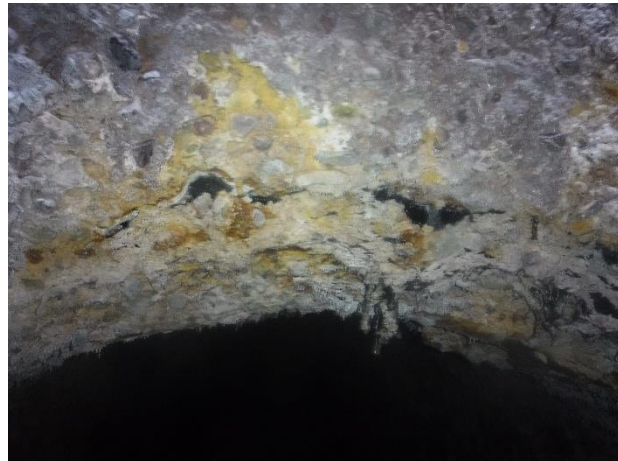
Photo 3-37. MH A39, Sever surface damage above inlet pipe. Concrete failure along inlet joint.
