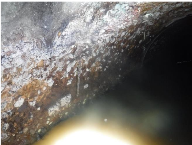
Photo A47 - 3. Left wall of downstream pipe, exposed aggregate protruding from wall.
