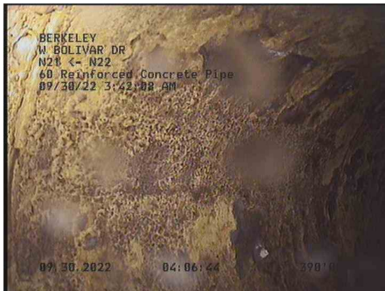
9, 00:16:11, 390.63ft Surface Damage Aggregate Visible from 10 o'clock to 2 o'clock, within 8 inch, Start
