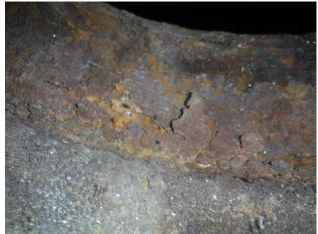
Photo N22-4. Moderate corrosion observed on manhole rim.
