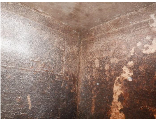
Photo S48 - 5. Upper walls of pipe in fair condition.
