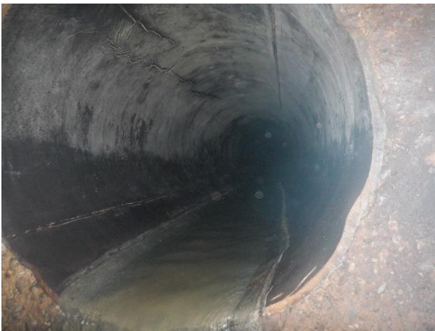
Photo S38 - 3. Large side lateral line.
