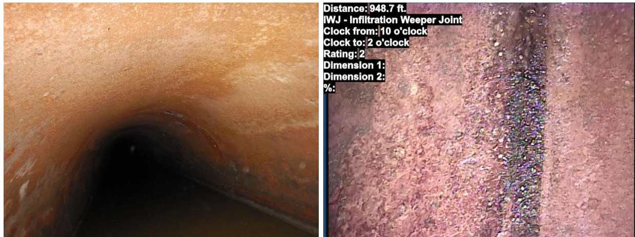
Photo 4-11. Minor surface damage in segment S38S391 at manhole S39
