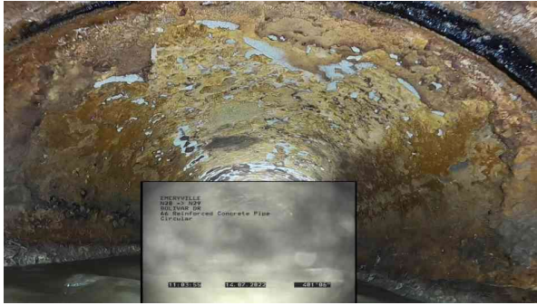
19, 00:08:33, 401.70ft Infiltration Stain from 9 o'clock to 3 o'clock, within 8 inch
