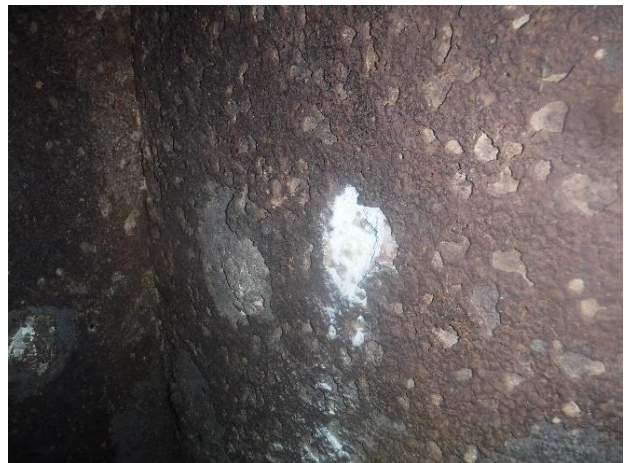
Photo S50 - 4. Chalky, white surface mortar exposed.
