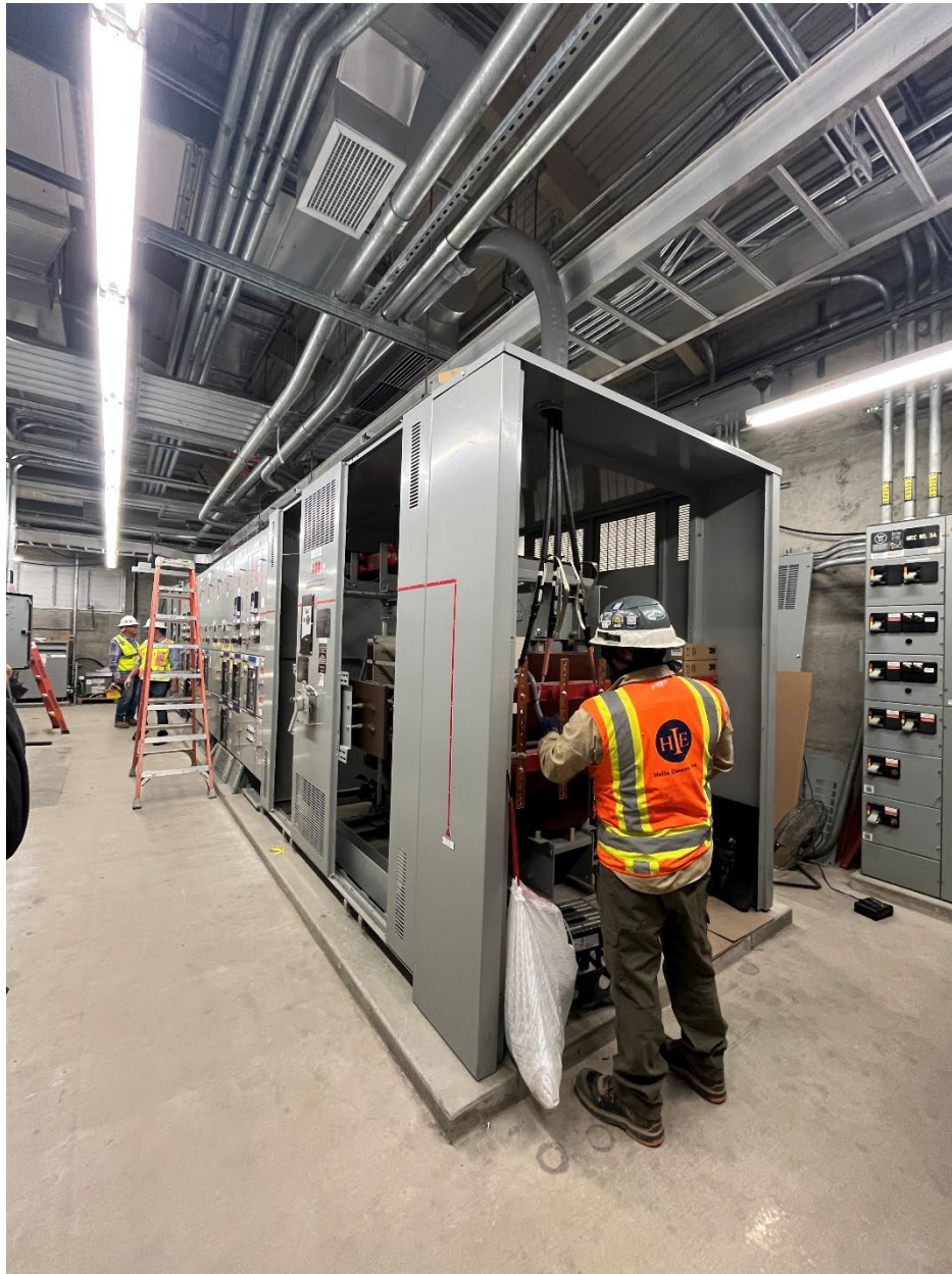
Figure 1 – USL WTP – Installation of new USS-01 Gear in Electrical Room. This electrical equipment provides primary power to the WTP from PG&E.
