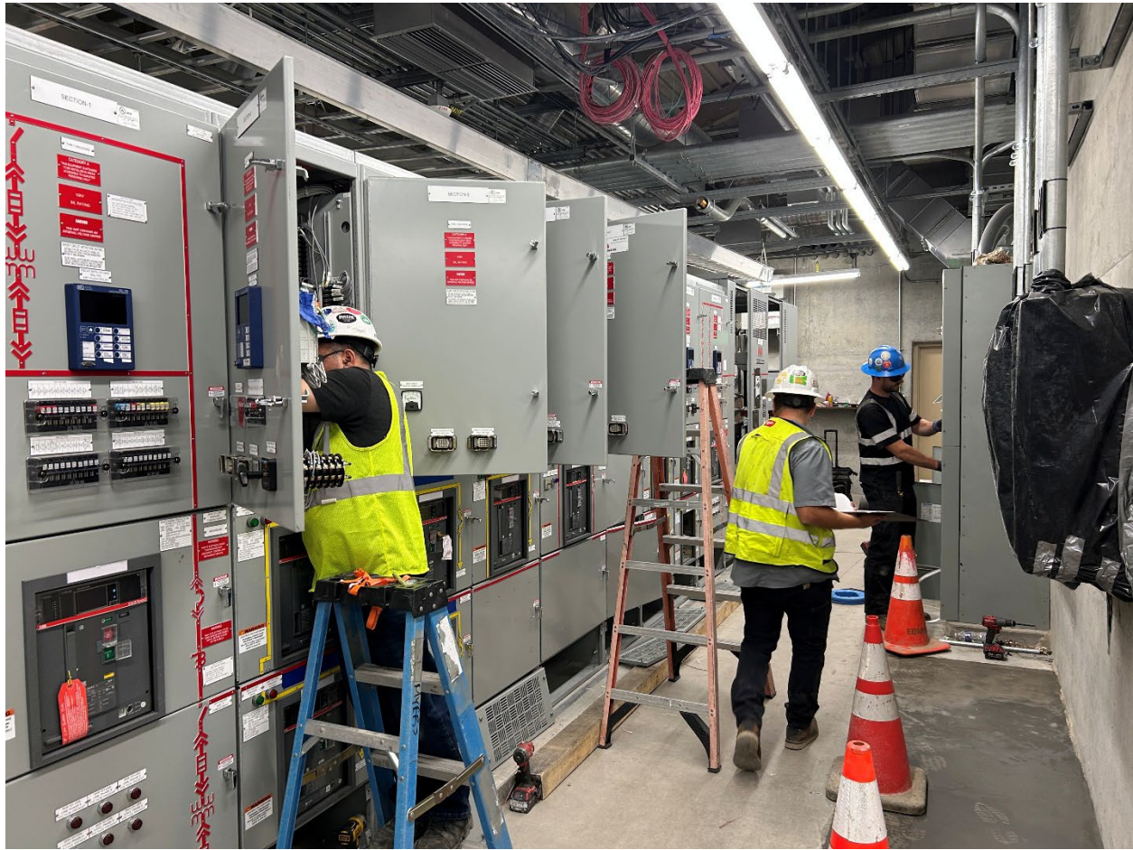
Figure 2 – USL WTP – Ongoing work on USS-01 equipment. This electrical equipment provides primary power to the WTP from PG&E.
