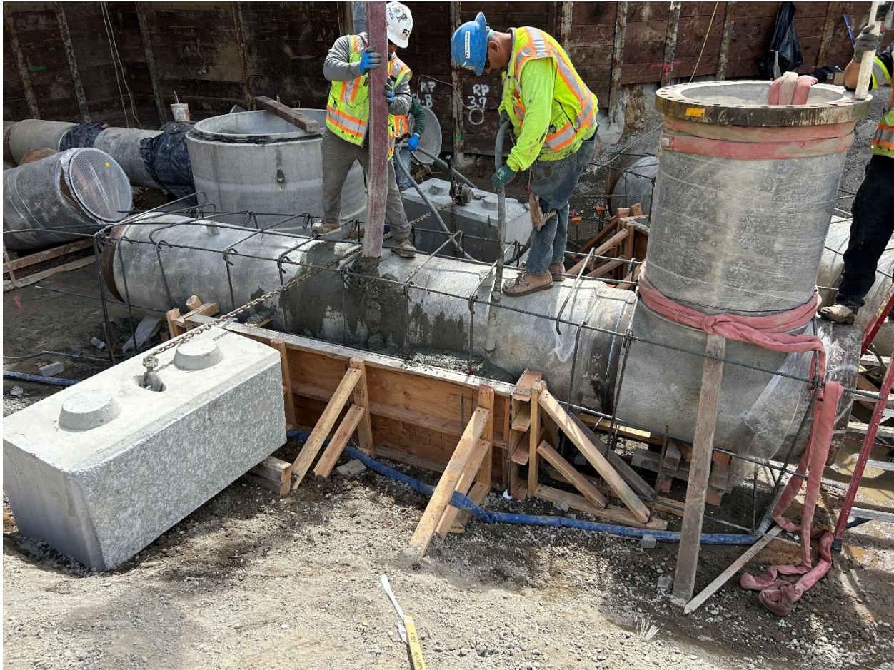
Figure 3 – Placement of North and South 30 Piping in the future CCB. This piping supplies water to the distribution system when the CCB operates as a clearwell for planned maintenance.
