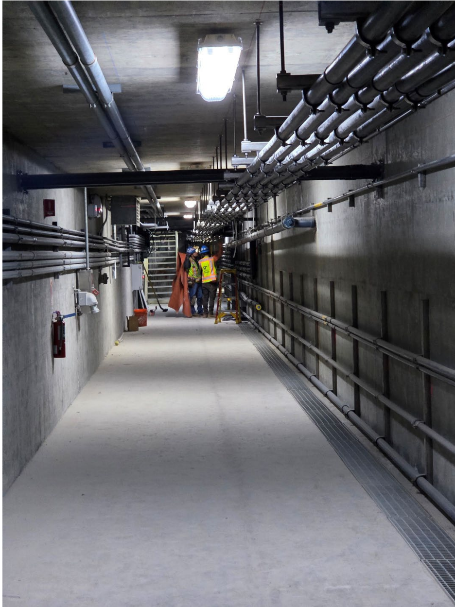
Figure 16 – Sobrante WTP newly installed chemical pipe runs in pipe gallery.
