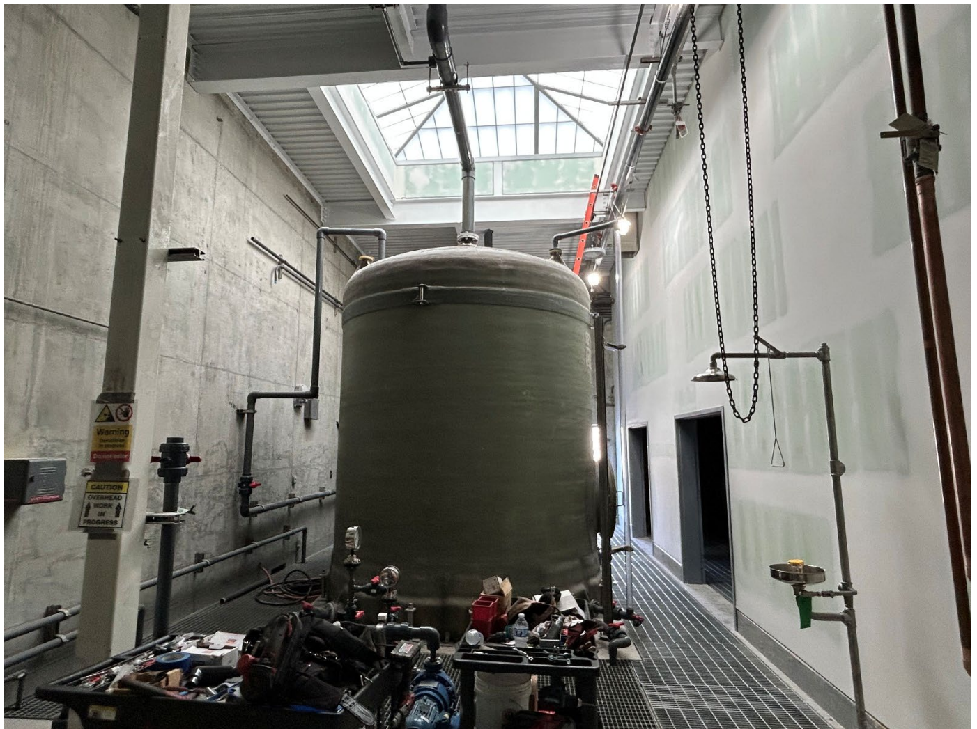
Figure 15 – Sobrante WTP: newly installed caustic soda chemical tank and skylight
