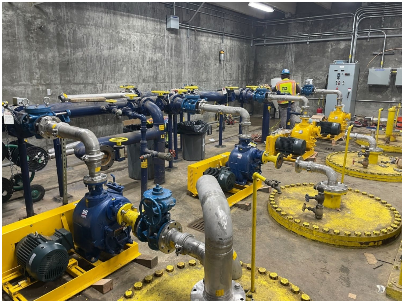
Figure 7 - Solids Pumping Plant: began installation of thickened solids and detention basins transfer pumps and associated piping
