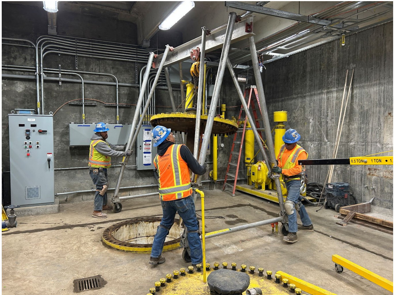
Figure 6 – Solids Pumping Plant: demolished existing pumps and piping and prepared the suction barrels for condition assessment
