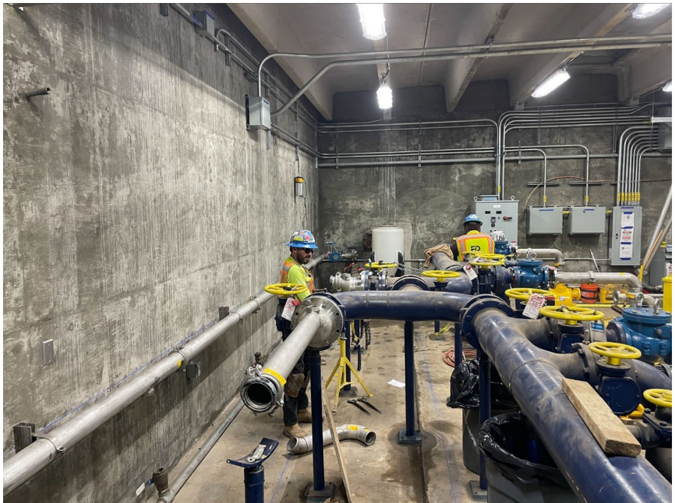
Figure 8 - Solids Pumping Plant: began installation of downstream solids removal piping and service water piping
