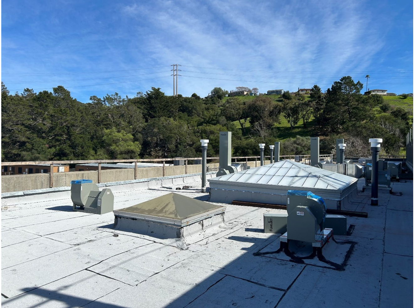
Figure 16 – Sobrante WTP Chemical Building Roof: completed skylights and roof repair in progress
