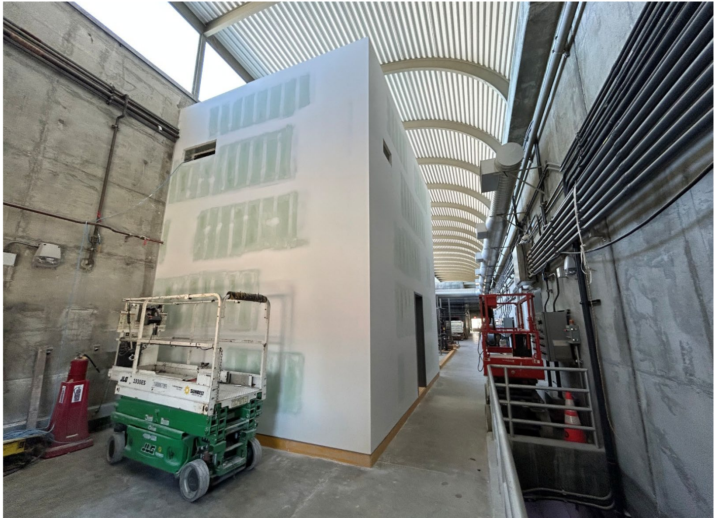
Figure 13 – Sobrante Chemical Building: new caustic soda room
