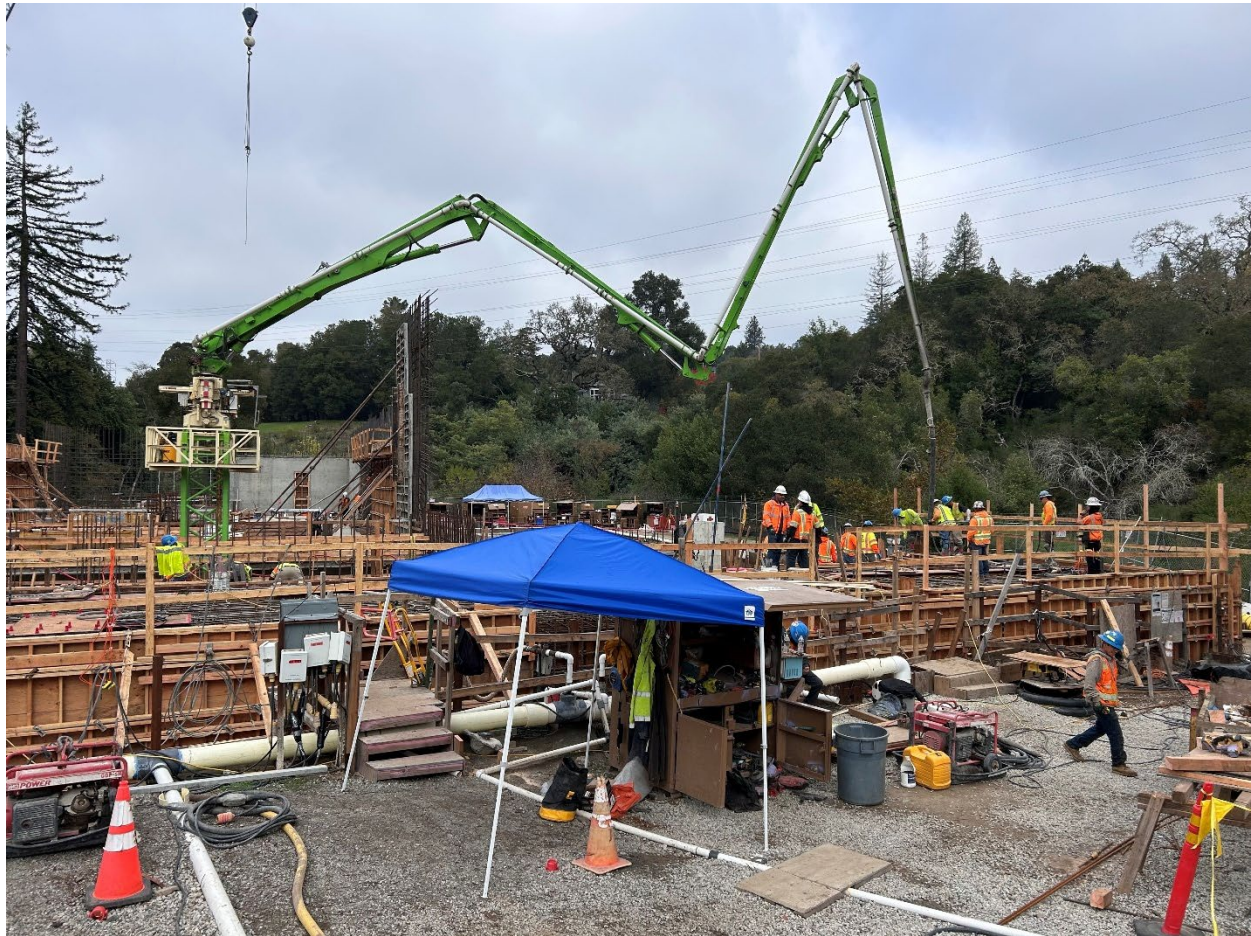
Figure 21 – Workers completing the final concrete pour for the roof of the Effluent Weir Structure with the aid of the green telescoping concrete pump.
