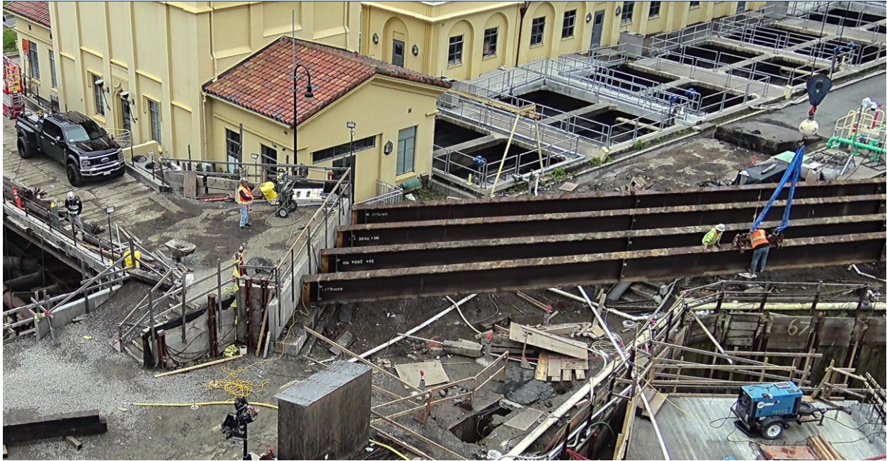
Figure 46 – Workers attaching crane sling to roadway beam of UV-CCB Facility temporary bridge in preparation for removal.
