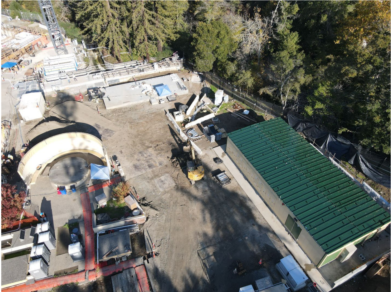
Figure 33 – Aerial view of completed SEB on the right and empty concrete pad, in the background, ready to receive the pre-fabricated LAPB.
