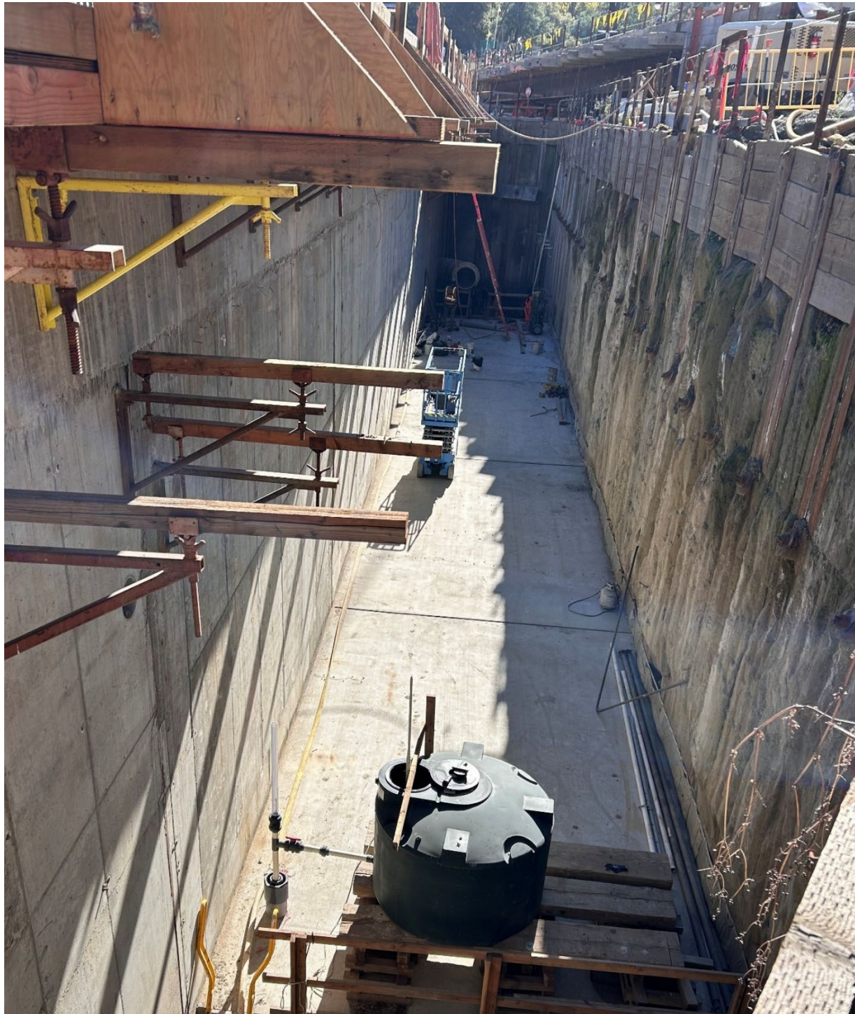
Figure 6 – Black plastic water reservoir providing static water level for hydrostatic water testing of the UV Influent Channel located underneath the concrete slab which the reservoir is resting upon.
