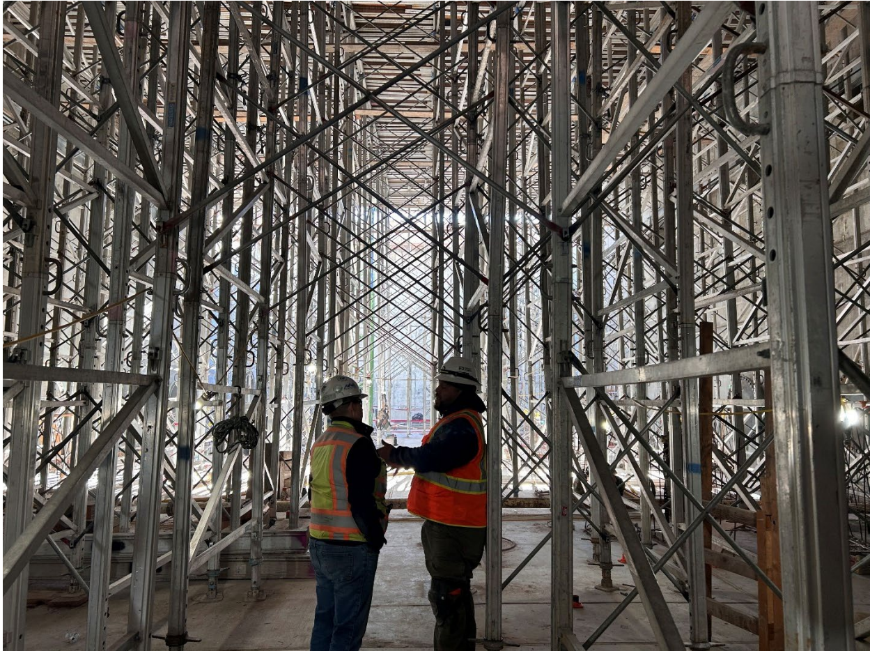
Figure 17 – View looking down the length of the UV Room with scaffolding towers providing temporary support for placement of the UV Room concrete roof slab, located 25-feet above the floor.
