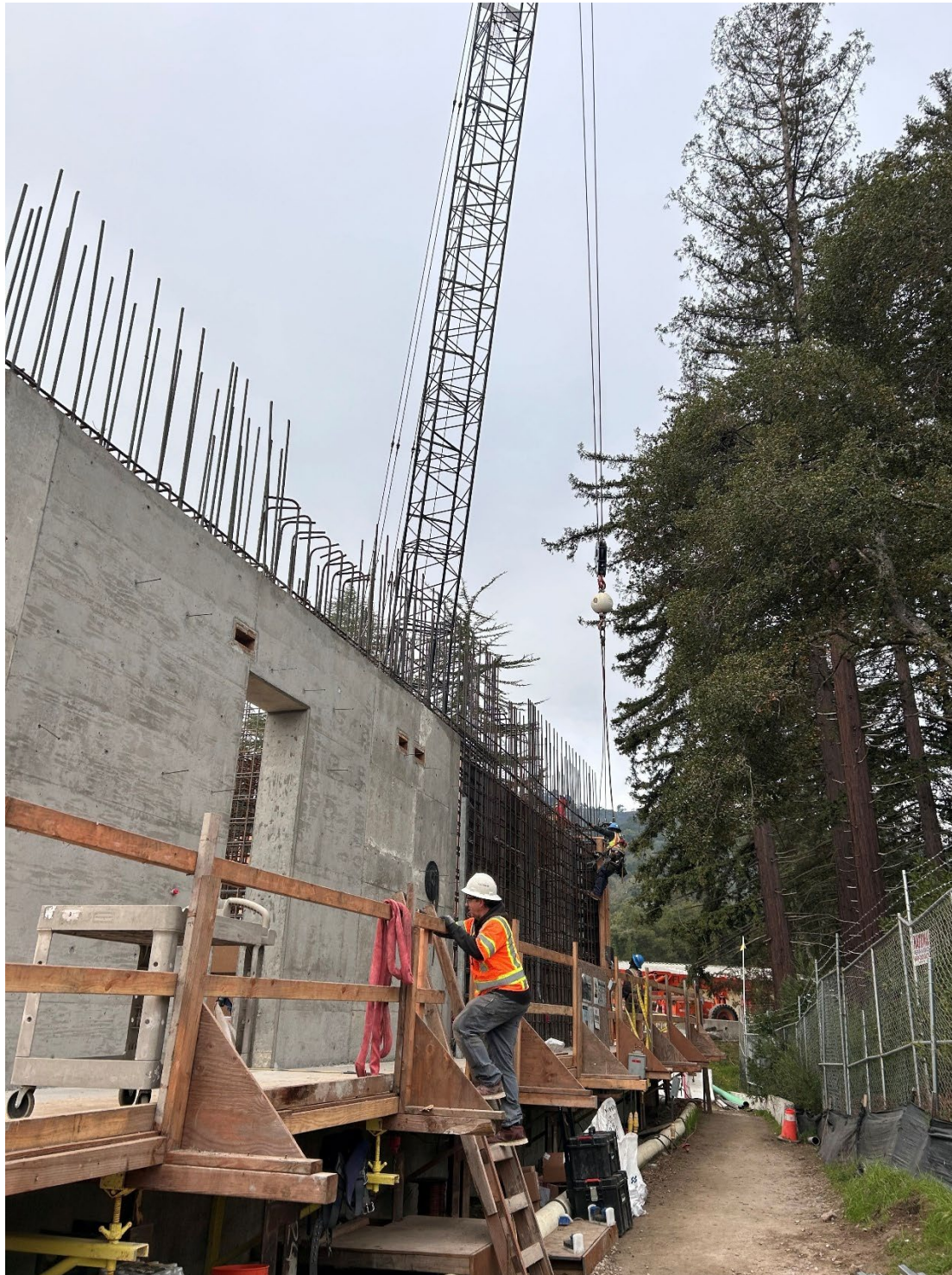
Figure 19 – Worker climbing onto the temporary catwalk which provides access for construction of the first level reinforced concrete walls for the future MAUVE Building.
