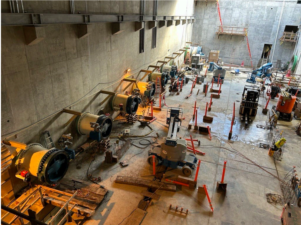
Figure 32 – 48-inch fabricated steel piping segments installed with isolation valves in the UV Room. Each of the six piping segments will be part of the six UV trains which will extend across the UV Room floor in the future.
