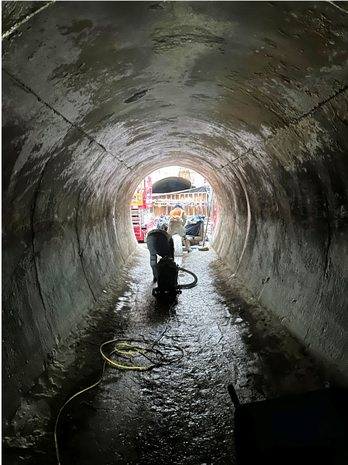
Figure 4 – Claremont Tunnel: view looking down length of the tunnel as workers clean it out in preparation for disinfection and return to service to end the outage.
