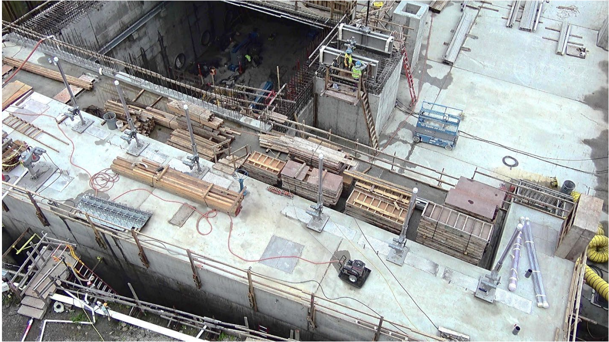
Figure 22 – Aerial view of the completed Effluent Weir Structure with the tall stems of the 6 effluent weir gates extending up out of the roof.
