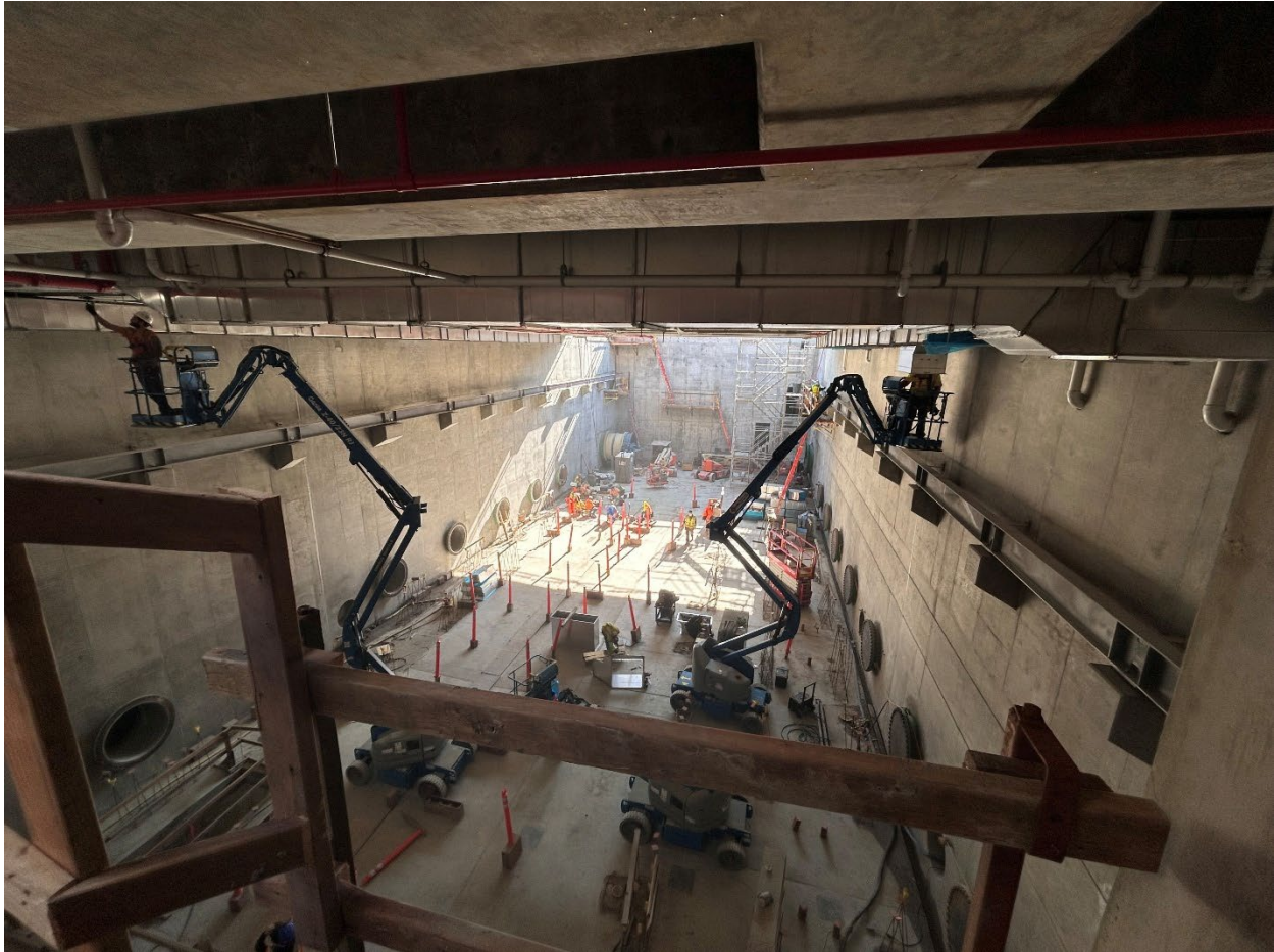
Figure 30 – View looking down the length of the UV Room (opposite direction from Figure 24) showing workers on telescoping lifts installing mechanical, electrical, and plumbing on the ceiling.
