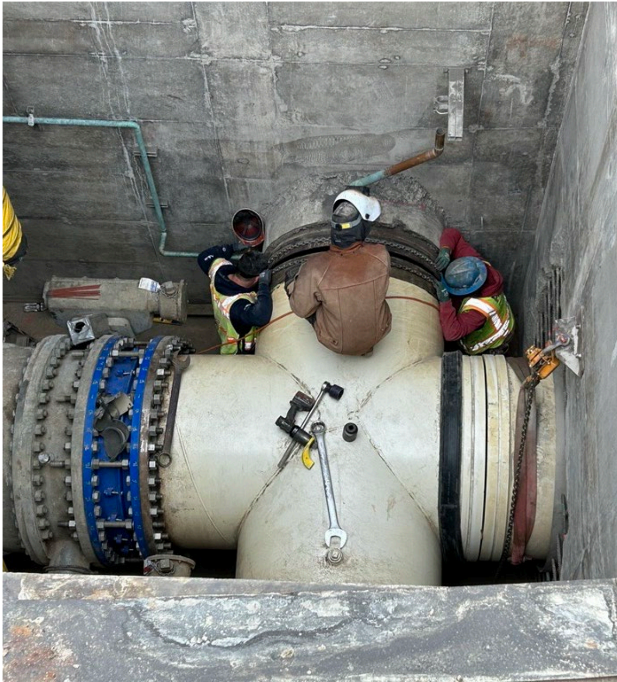
Figure 13 – Workers connecting special 48-inch steel piping piece to existing piping using a welded butt strap connection.
