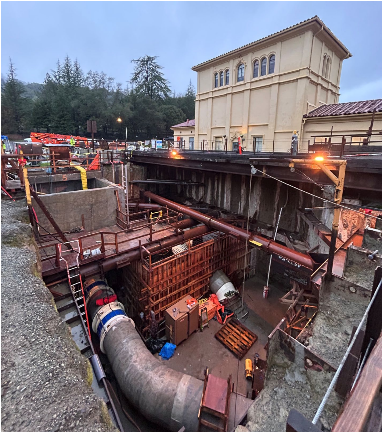
Figure 16 – View looking down into Effluent 1 excavation showing piping completed and wooden wall forms in the foreground which will provide temporary support for future underground Effluent 1 vault walls.
