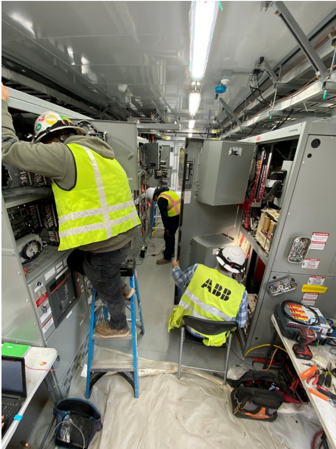
Figure 36 – Electricians completing reconnection and wiring of electrical gear inside the pre-fabricated LAPB.
