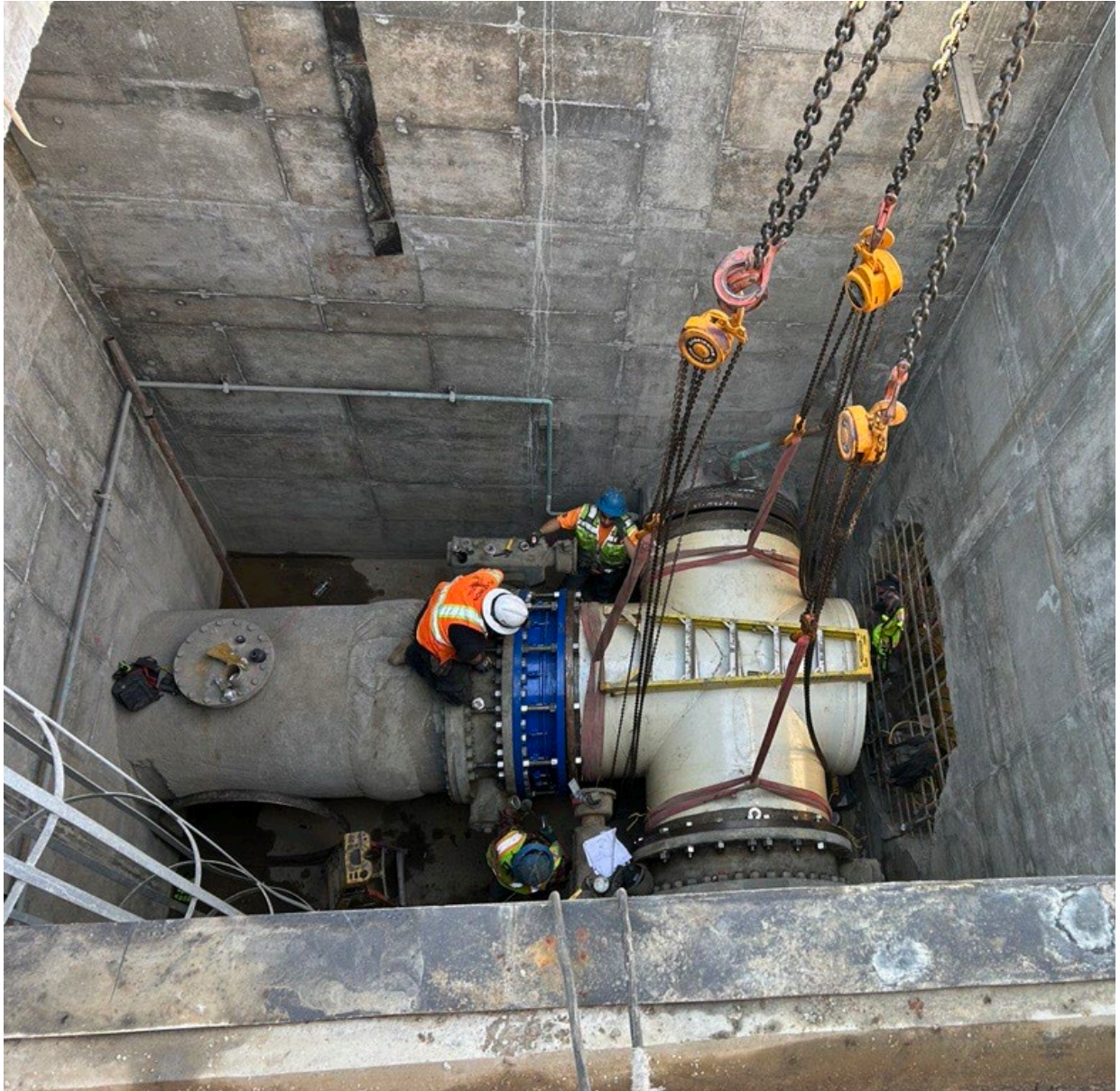
Figure 12 – View looking down into LAPP2 suction piping vault of workers positioning special 48-inch steel piping piece with the aid of a crane located above.
