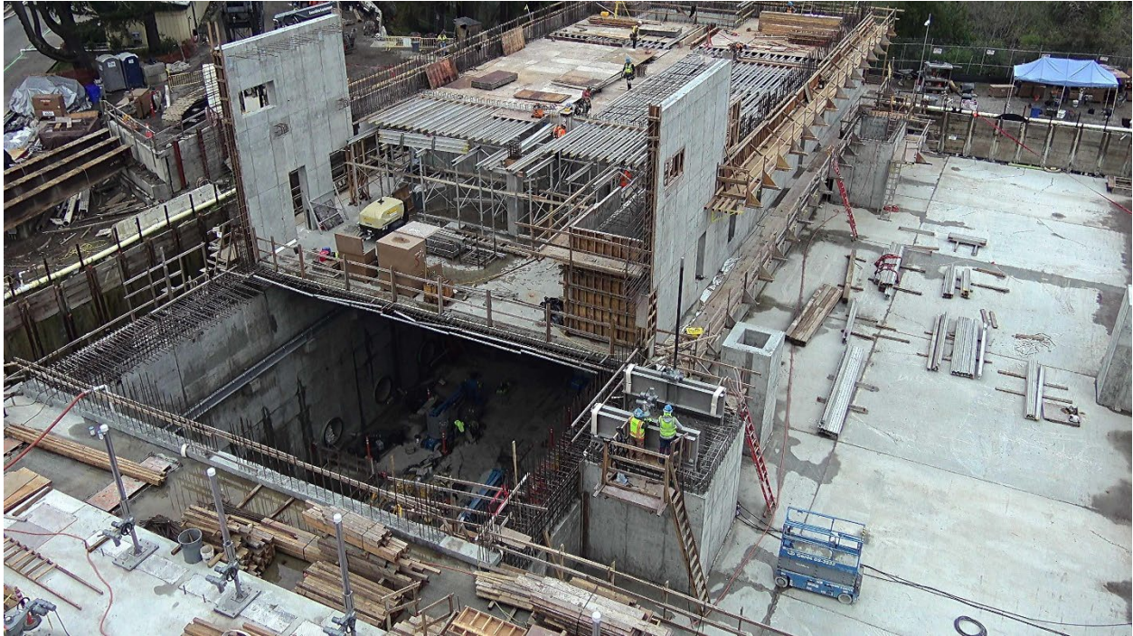
Figure 23 – Aerial view of the UV-CCB Facility. The contractor is only building the north end of the MAUVE Building at this point to maintain clear access for bringing materials into the UV Room below through the large opening shown in the lower left of the photo.
