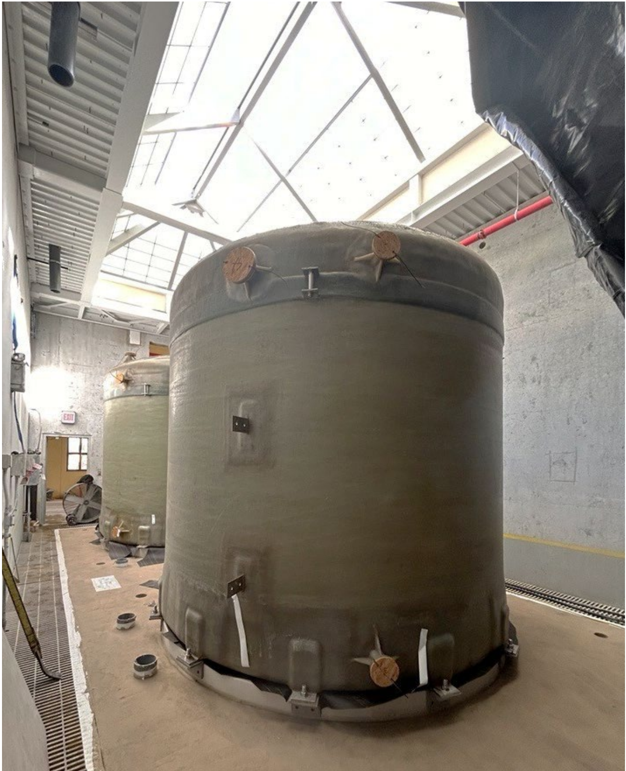
Figure 41 – New fiberglass reinforced plastic chemical tanks and skylights installed in the Chemical Building.
