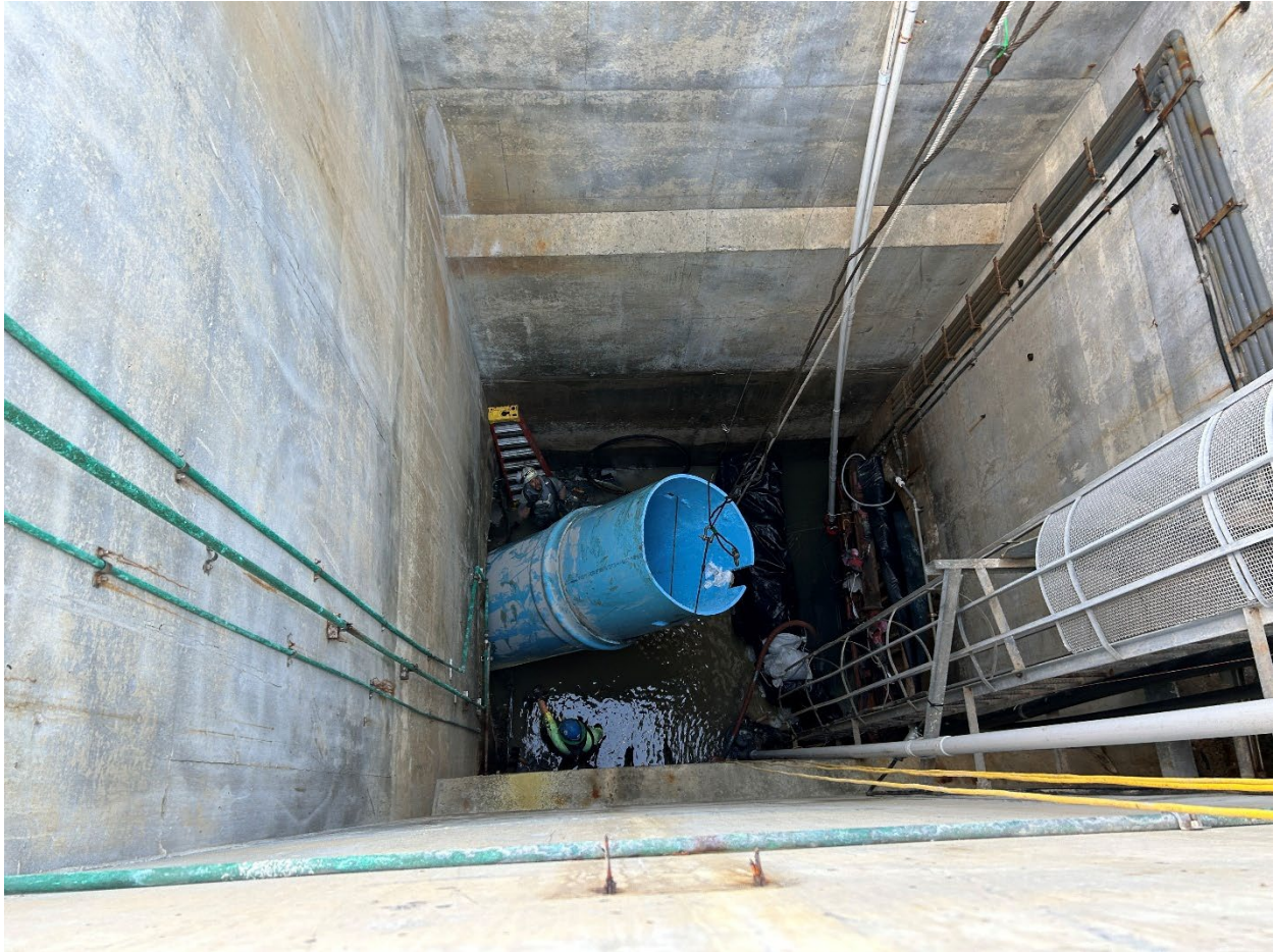
Figure 3 – Claremont Tunnel Access Shaft: view looking down as crane lifts 48-inch Effluent 1 bypass piping out of the tunnel.
