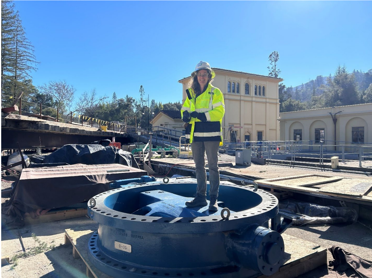
Figure 26 – Engineer standing on top of 84-inch valve to show scale. The valve will be placed in the UV Room for hydraulic isolation of the bypass piping.
