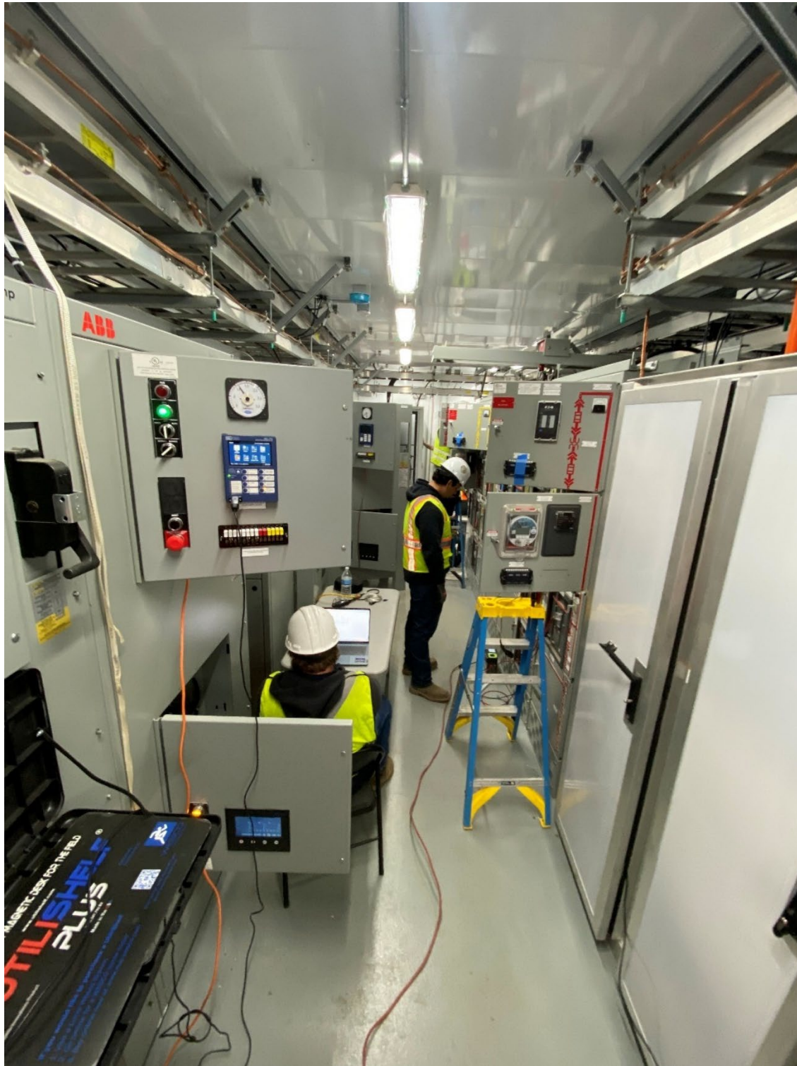
Figure 37 – Engineers performing testing of electrical gear inside the pre-fabricated LAPB.
