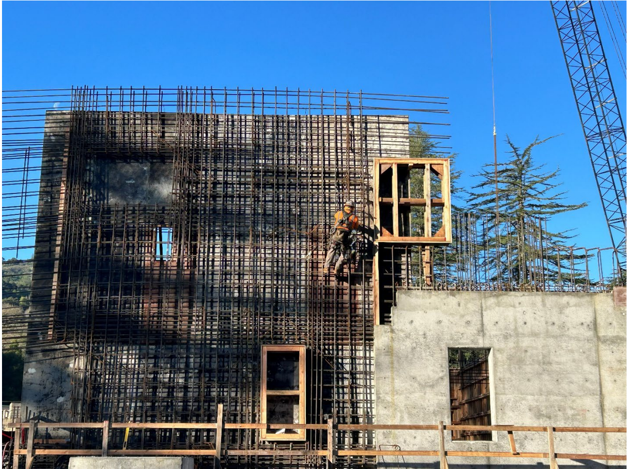
Figure 20 – Worker connecting reinforcing steel for full height concrete wall which will serve as the exterior wall for the first two floors of the future MAUVE Building.
