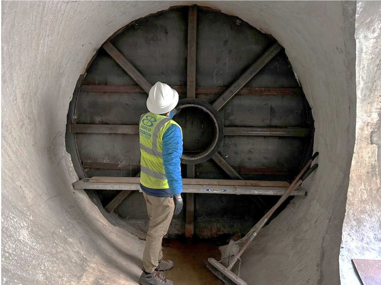
Figure 5 – Engineer inspecting 108-inch steel bulkhead installed for hydrostatic testing of the UV Influent Channel.
