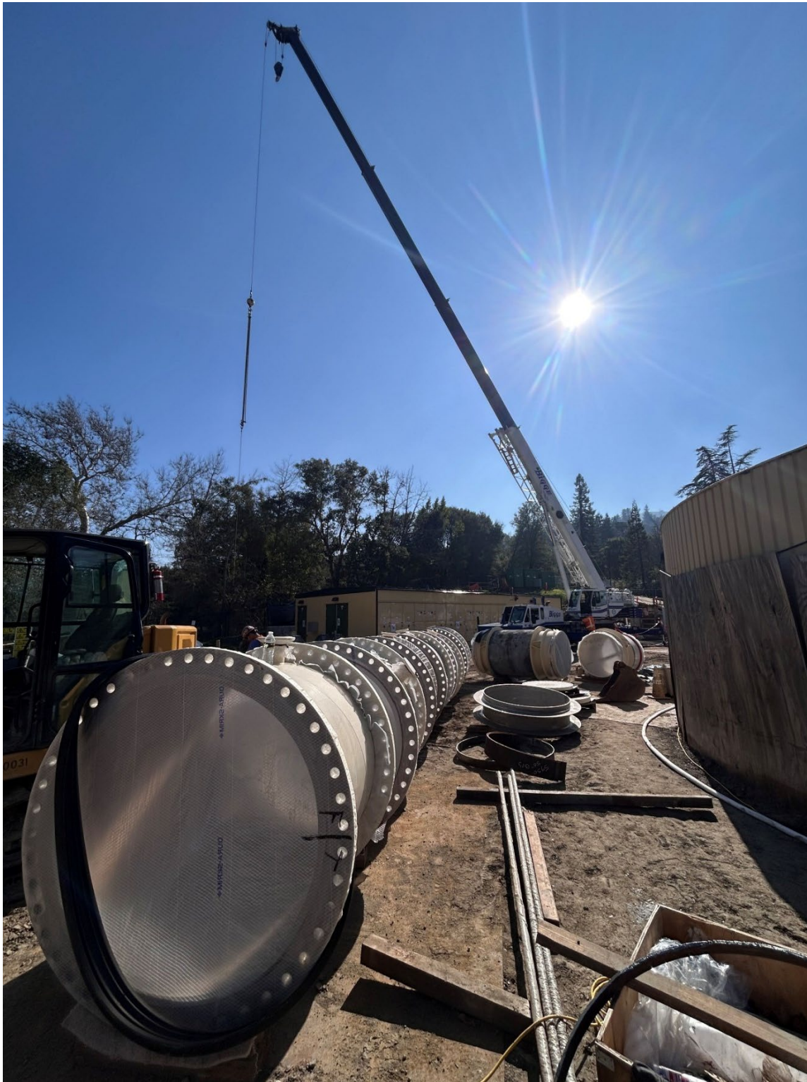
Figure 31 – Crane in the background ready to lift 48-inch fabricated steel piping segments which into the UV Room.
