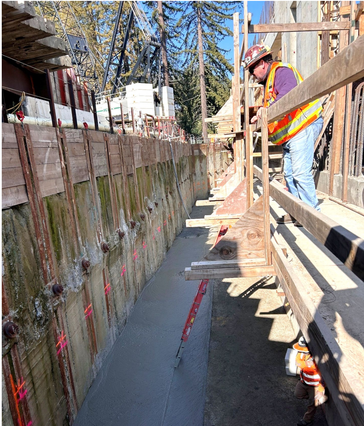
Figure 10 – Inspector watching workers below place flowable fill to bury 36-inch LAF1 Wasteway steel piping and UV Influent Channel.
