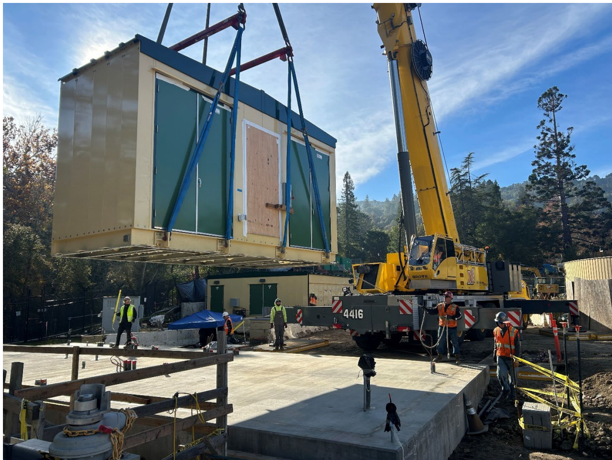
Figure 35 – Closeup view of crane lifting first segment of the pre-fabricated LAPB onto the prepared concrete foundation.
