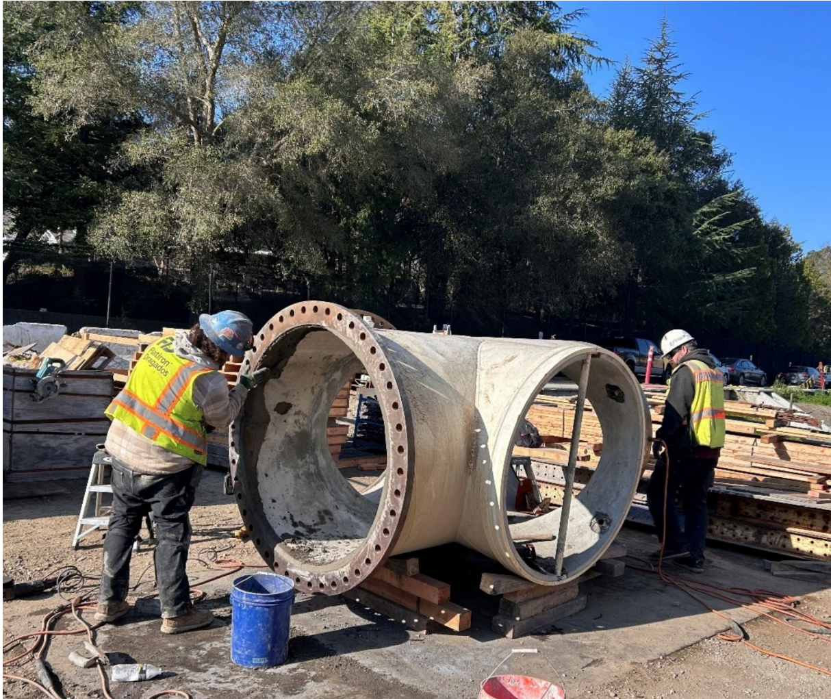
Figure 11 – Workers applying protective mortar lining inside special 48-inch steel piping piece for LAPP2 suction piping.
