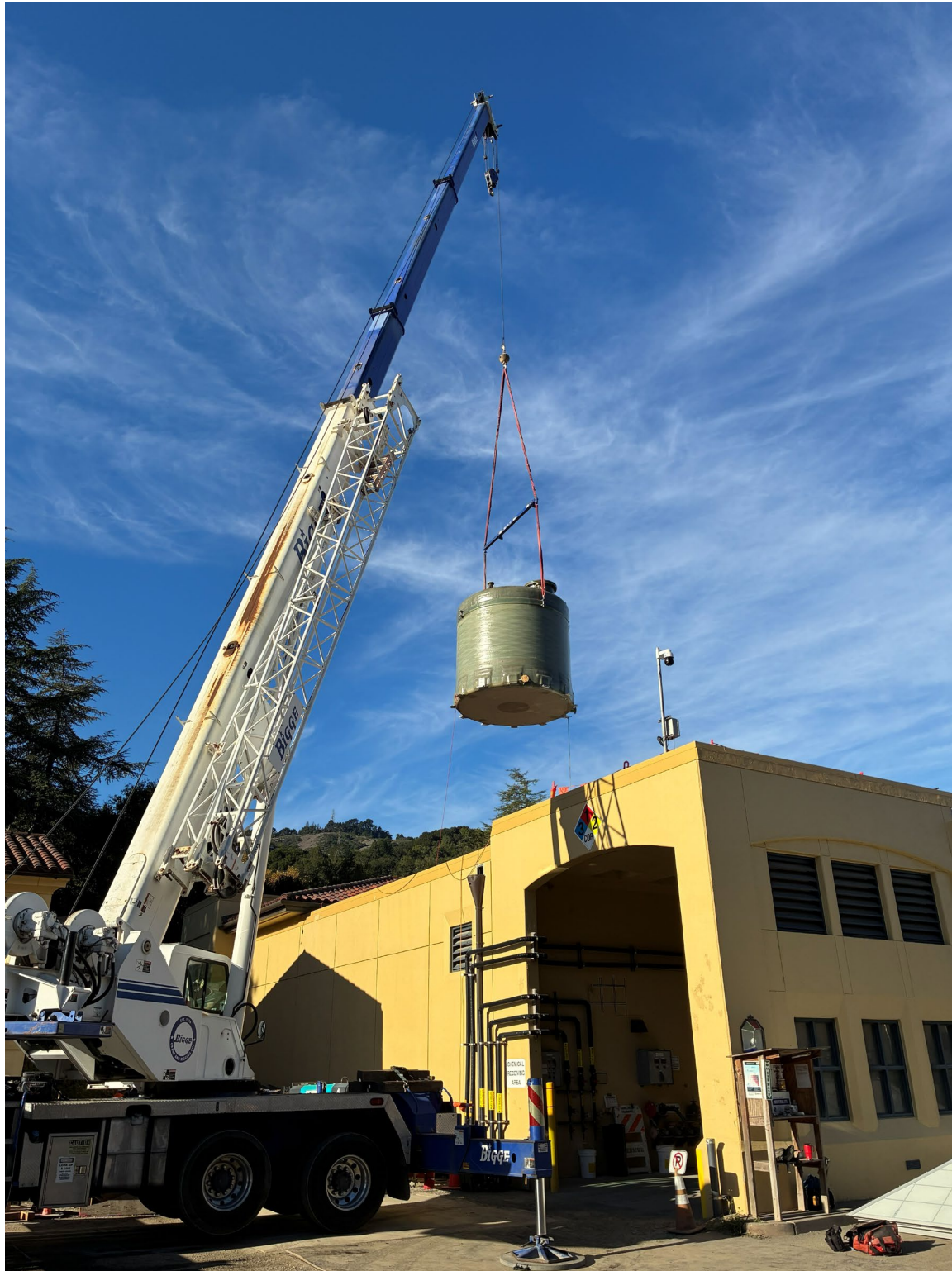
Figure 39 – Crane lowering fiberglass reinforced plastic chemical tank into Chemical Building through the roof opening.
