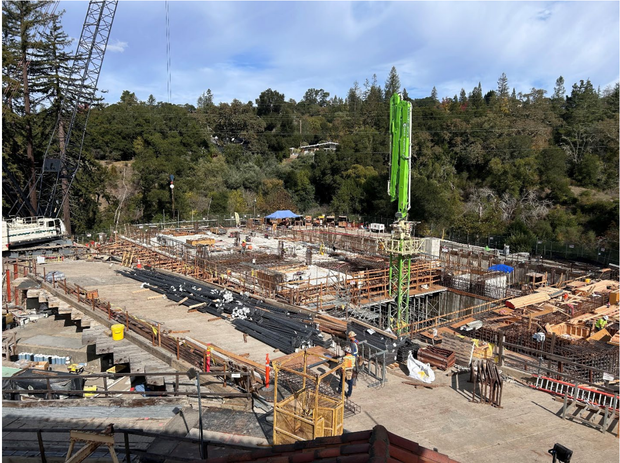
Figure 18 – View of the completed UV Room concrete roof slab which serves as the ground level floor for the future MAUVE Building.
