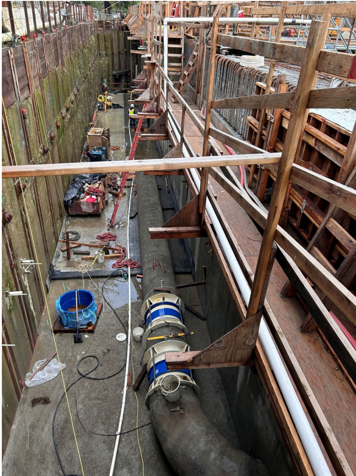
Figure 9 – 36-inch LAF1 Wasteway steel piping installed on the roof of the UV Influent Channel.
