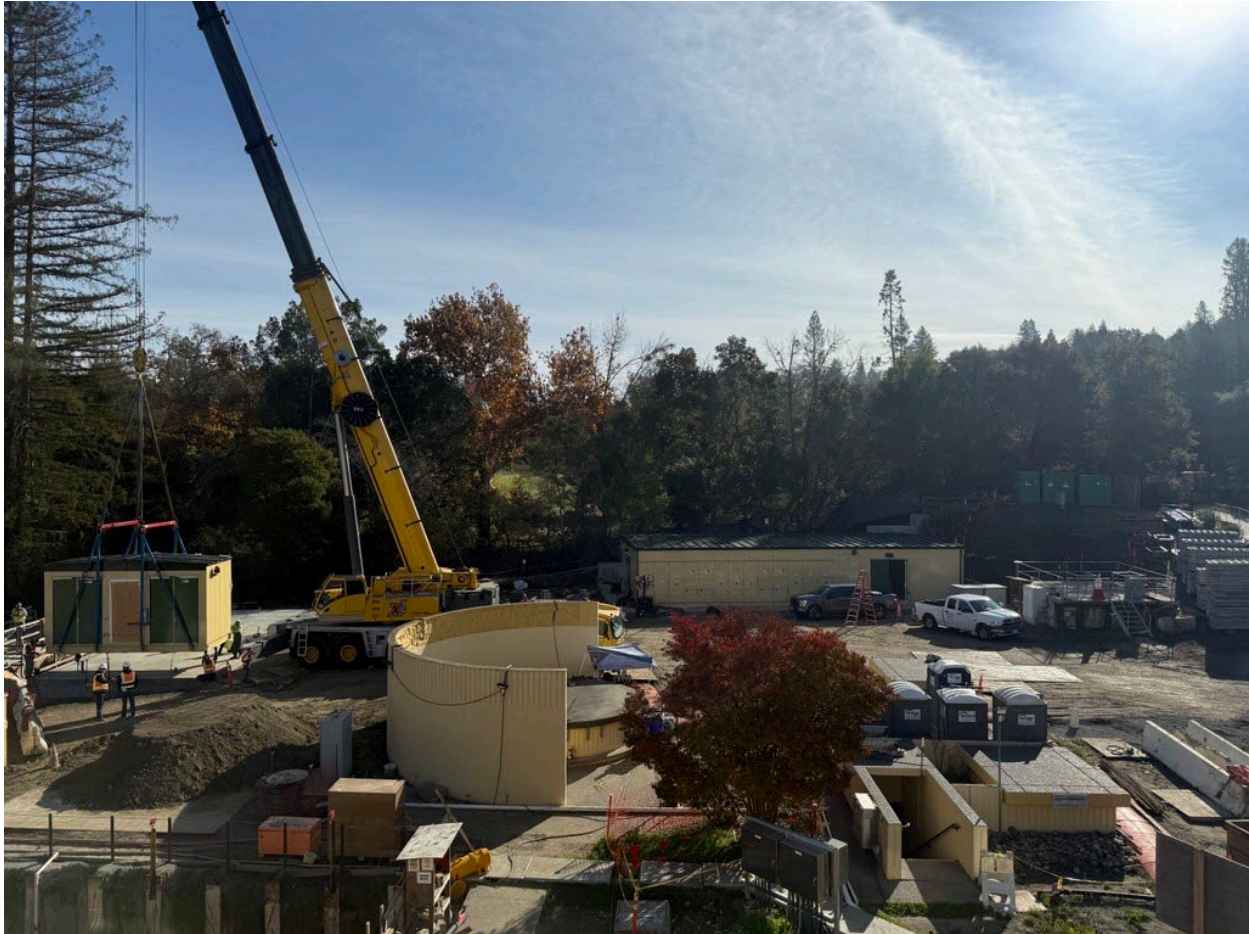
Figure 34 – View of crane lifting first segment of the pre-fabricated LAPB on the left side of the photo.
