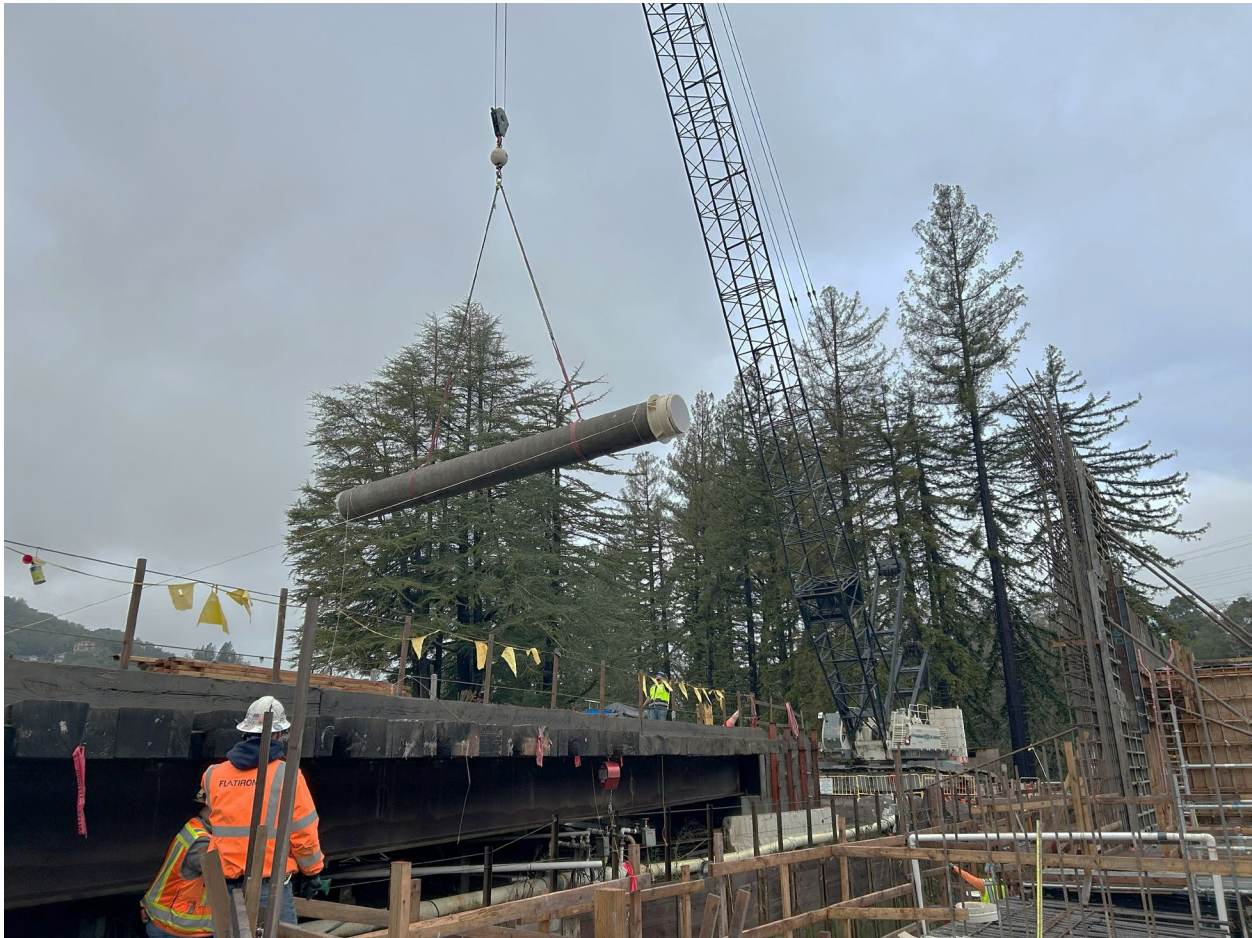
Figure 8 – Crawler crane lifting 40-foot segment of 36-inch LAF1 Wasteway steel piping from the temporary bridge into the trench located below.
