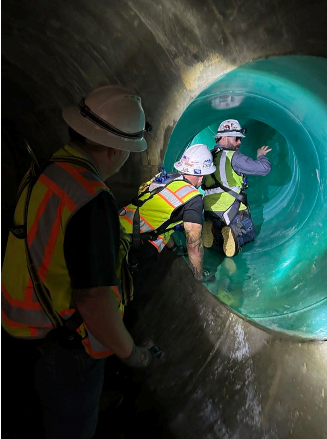
Figure 14 – Inspector kneeling in 48-inch branch line providing feedback to contractor’s staff who are standing inside 108-inch Effluent 1 steel piping.
