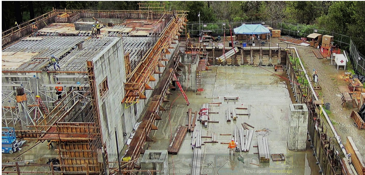
Figure 20 – Aerial view of UV-CCB Facility. On the left, workers are placing temporary scaffolding and decking support for reinforced concrete deck which will serve as the support for the second floor of the future MAUVE Building. On the right, there is a depressed concrete slab which is the roof of the underground CCB. This structure will be buried in soil soon. In the meantime, workers are staging materials for the operation happening on the left side of the photo.
