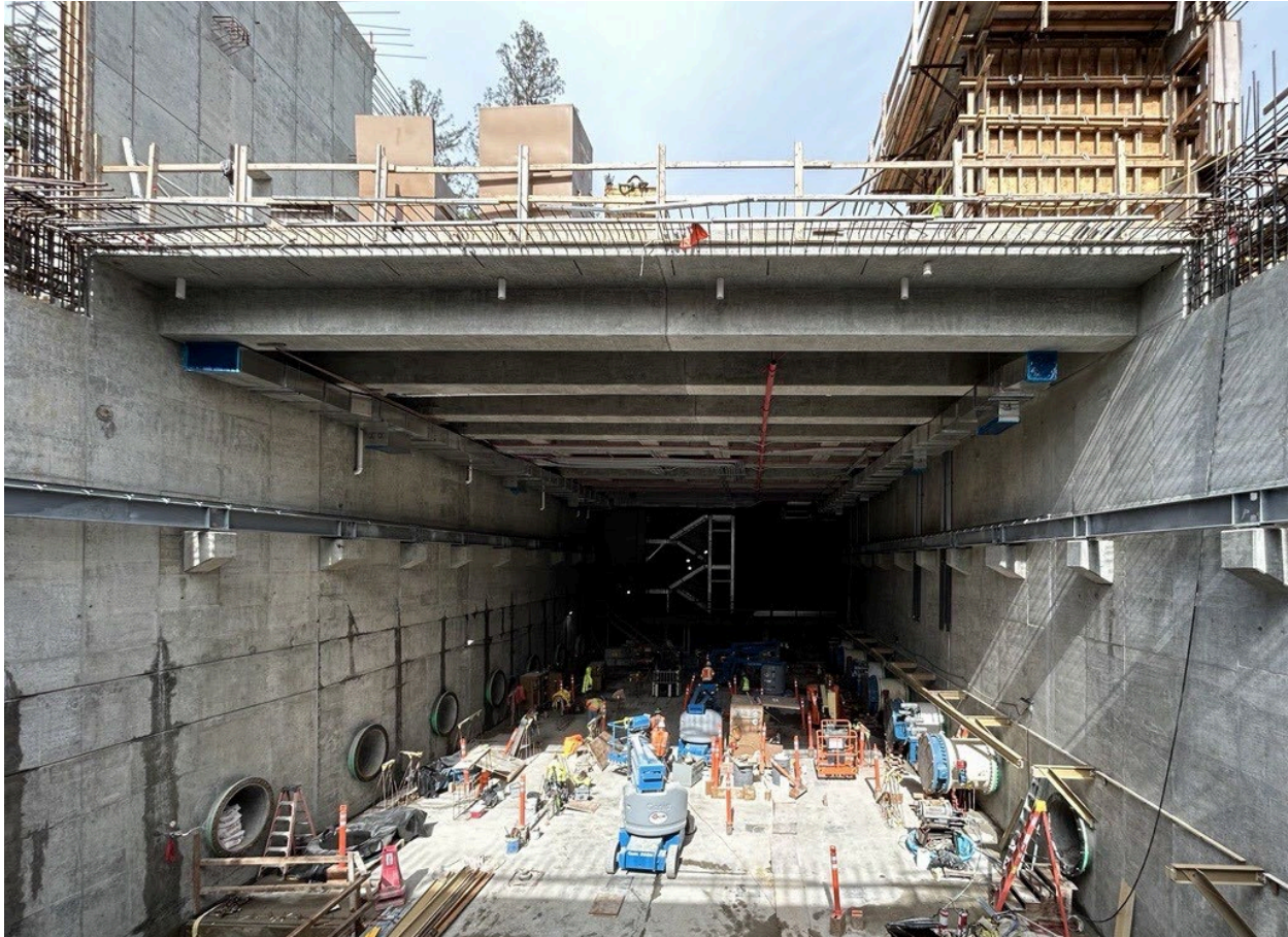
Figure 24 – View looking down the length of the UV Room showing the temporary scaffolding towers removed.
