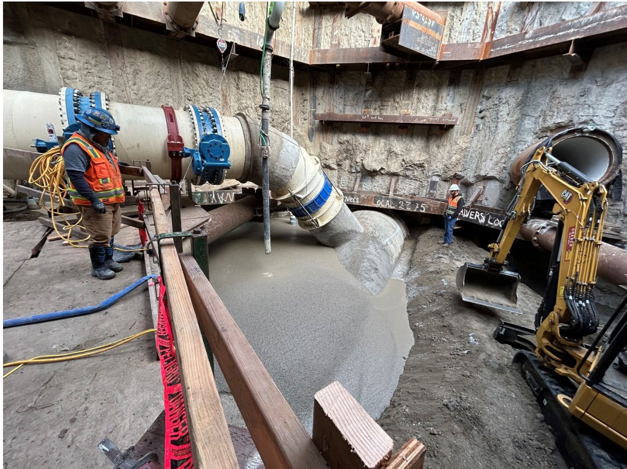
Figure 15 – Workers backfilling 108-inch Effluent 1 steel piping with flowable fill inside the Effluent 1 excavation.
