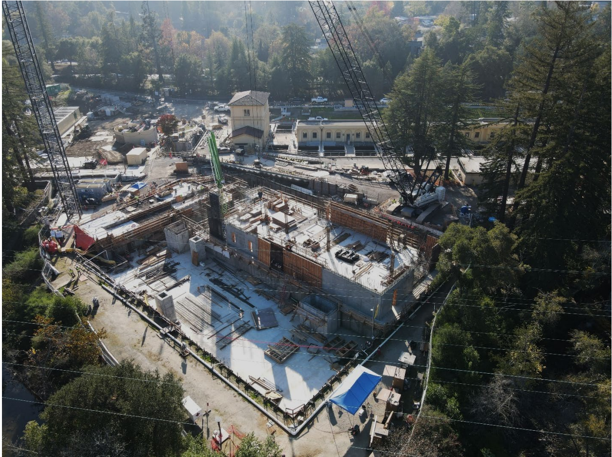
Figure 1 – Aerial View of UV-CCB Facility
