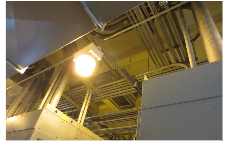
Conduit runs inside building
