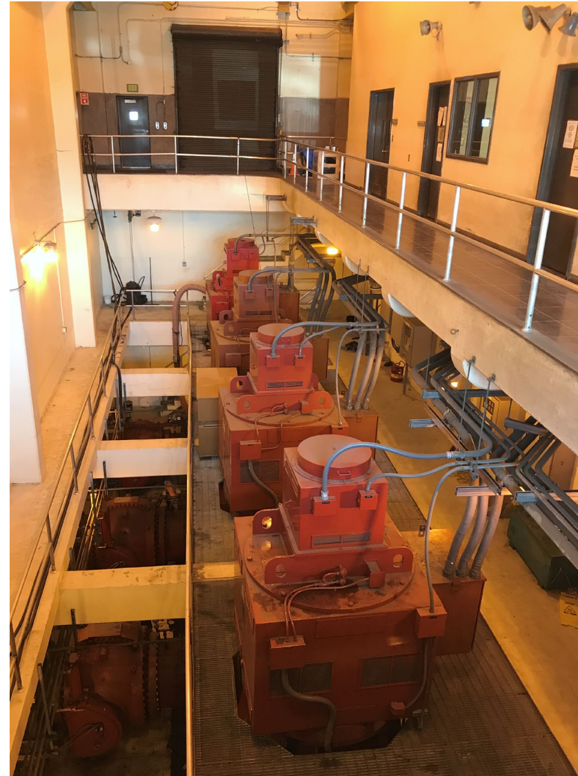
Pump Room Inside IPS
