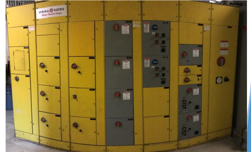
Aging and Obsolete Electrical Infrastructure
