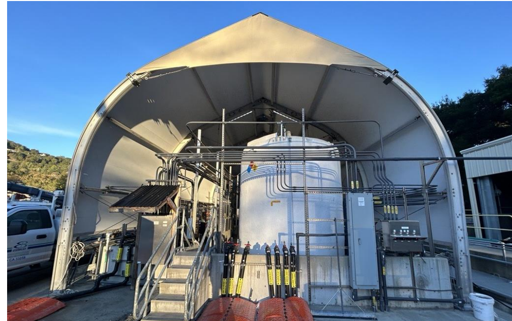
Temporary chemical system at Orinda WTP
