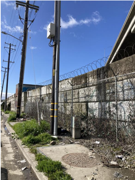
Both PG&E Grid Connections Vulnerable to Damage
