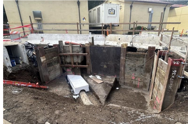
Unforeseen underground conditions at Sump 2
