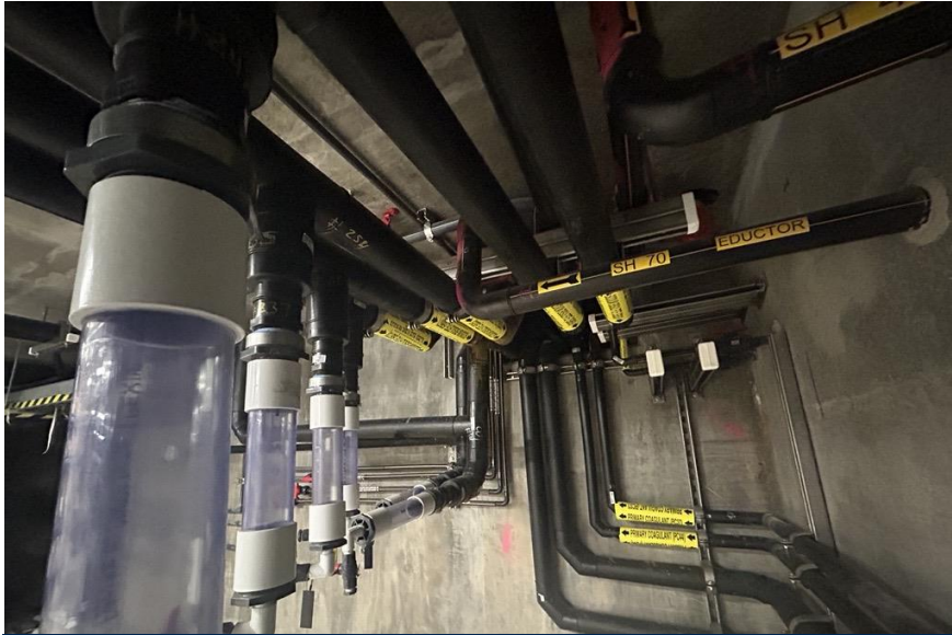
View inside chemical building at Orinda WTP, showing wall of piping entering a chemical trench
