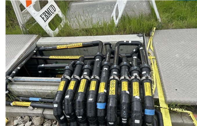
Temporary chemical lines tied into live lines
