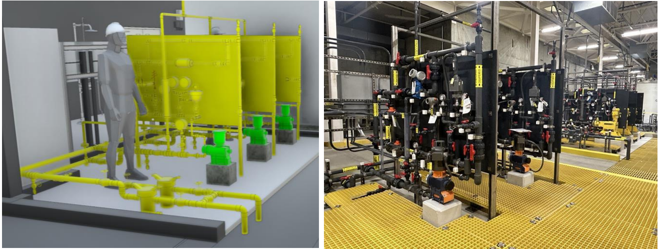
Figure 38 -- The two figures show a comparison between the designed and constructed chemical systems. On the left you can see the innovative 3D design aid used to visualize the space to O&M staff. On the photo of the right, you can see the completed installation with clear pathways between each system and the orderly and uniform installation of the large amount of equipment in a small space.
