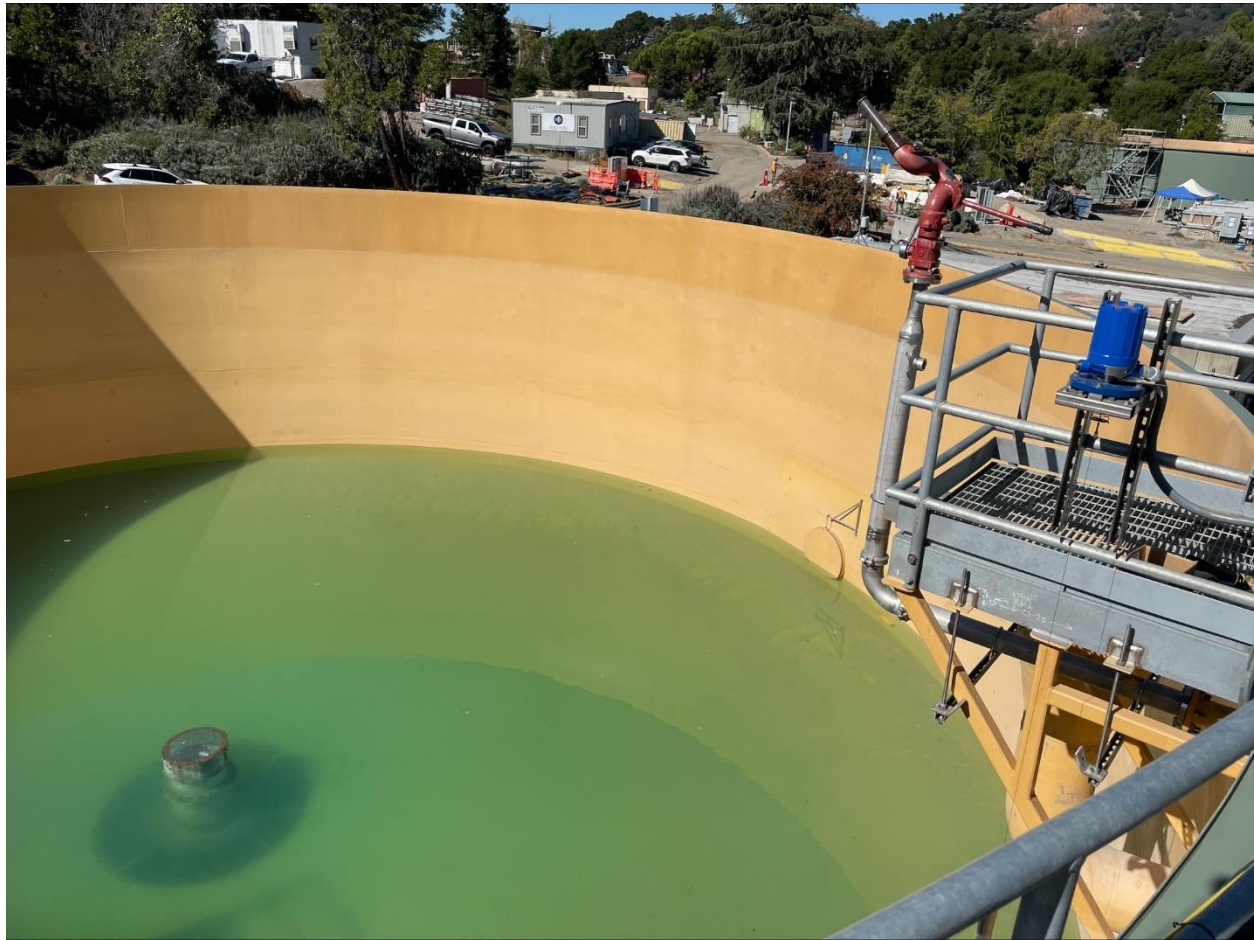
Figure 8 – Spent Washwater Basin No. 2 in service
