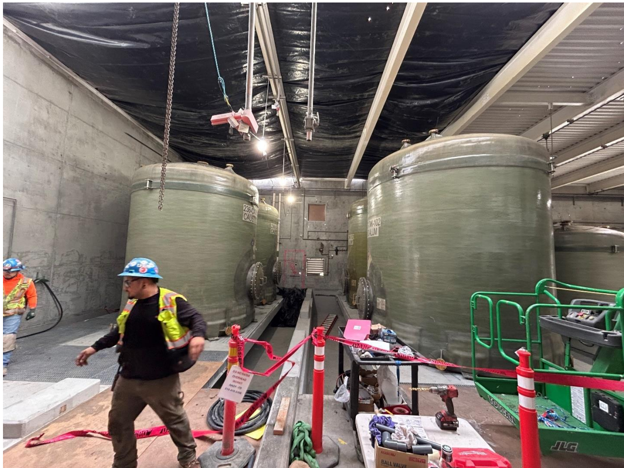
Figure 16 – Sobrante WTP new fiberglass reinforced plastic (FRP) chemical storage tanks
