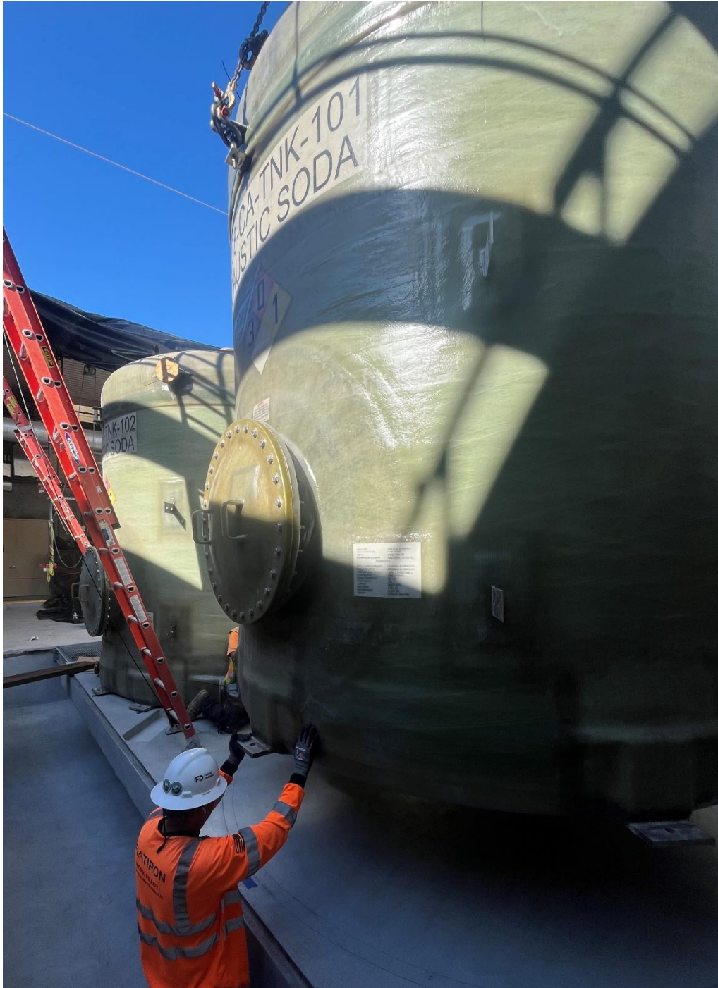
Figure 11 – USL chemical system - newly installed Caustic Soda Tanks
