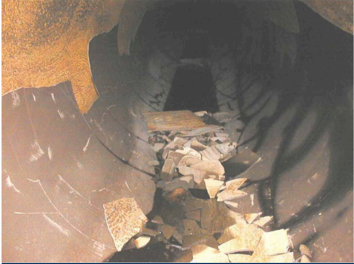
Delaminated Lining Accumulated on Pipe Invert
