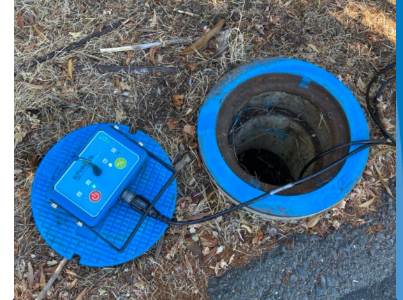
Non-Invasive Condition Assessment Sensor in Valve Pot
