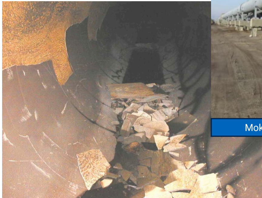
Failed Mortar Lining Accumulated in Pipe
