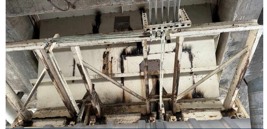
Corroded and Leaking Hoppers
