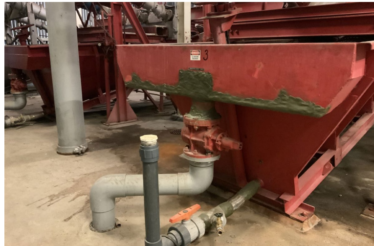
Repaired Grit Dewatering Equipment
