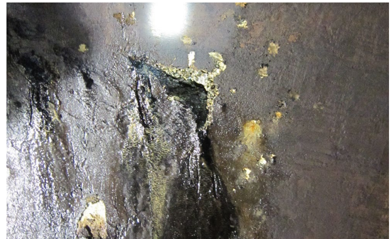
Typical Tunnel Lining Defect
