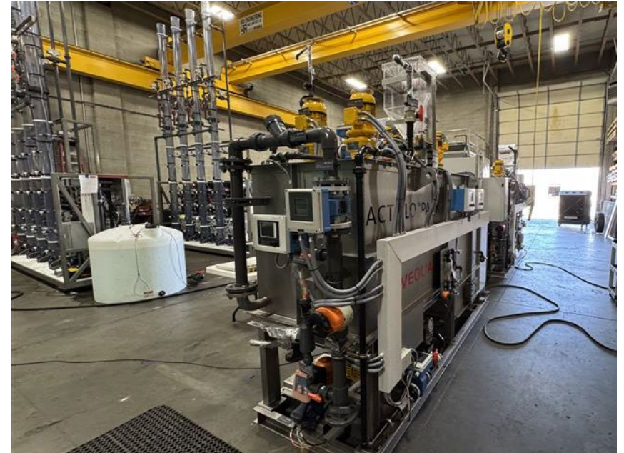
Water Quality Research Facility Pilot Testing Equipment
