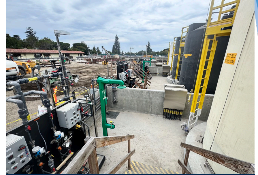
Photo of Temporary Chemical System at USL WTP
