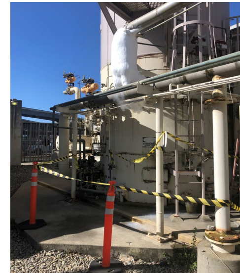
Failing and Leaking Pipes
