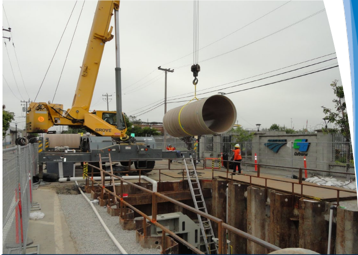
29 Miles of Large-Diameter Interceptors
