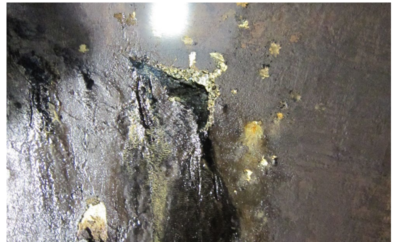
Typical Tunnel Lining Defect
