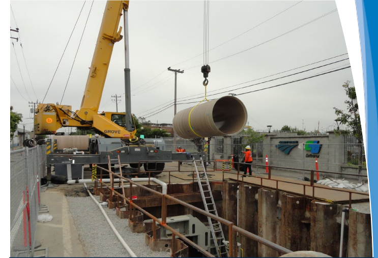
29 Miles of Large-Diameter Interceptors
