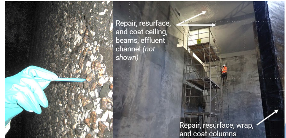
Secondary Reactor Interior
