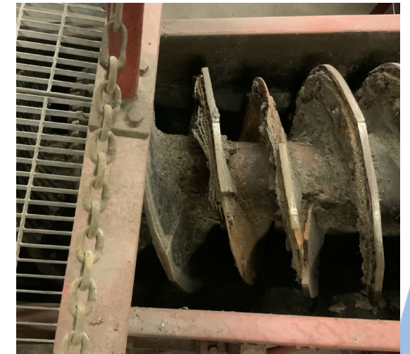
Damaged Grit Screws
