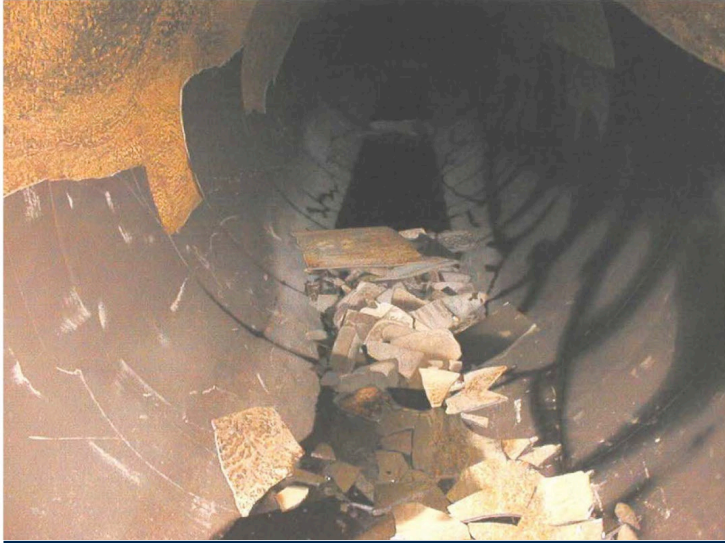
Delaminated Lining Accumulated on Pipe Invert
