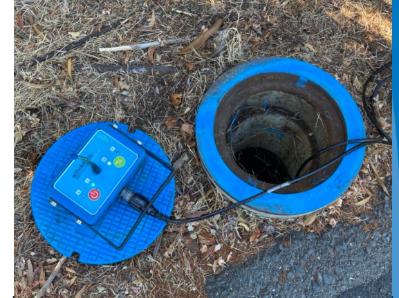
Non-Invasive Condition Assessment Sensor in Valve Pot
