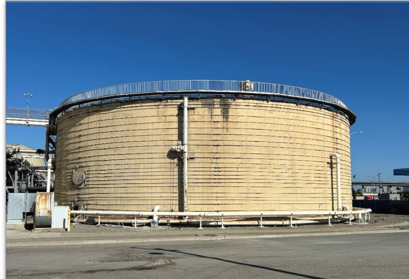
Typical Primary Digester
