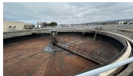
Drained Clarifier Before Rehabilitation
