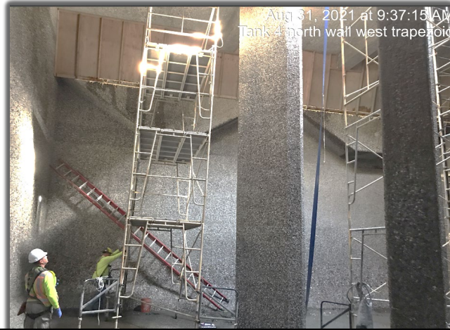
Inside Reactor. Concrete to be resurfaced & coated.
