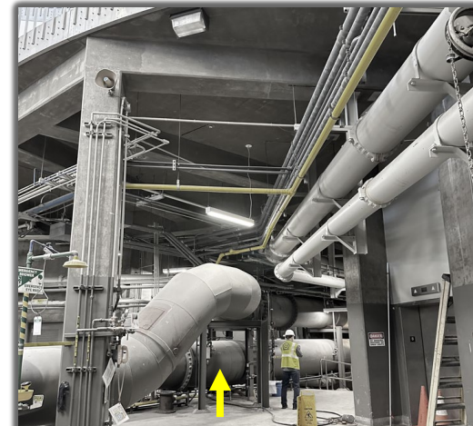
42" ø RAS pipe. Pipe will be repaired and relined.
