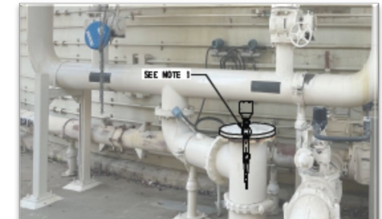
New Overflow Temperature Sensors
