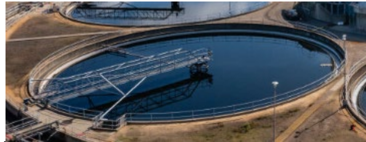
Clarifier in Operation
