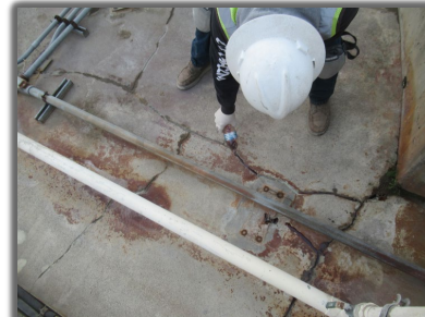
Cracks in the Reactor Deck. Cracks to be sealed with epoxy.
