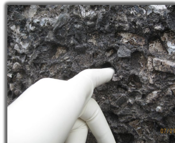
Corroded Concrete. Concrete aggregate exposed.
