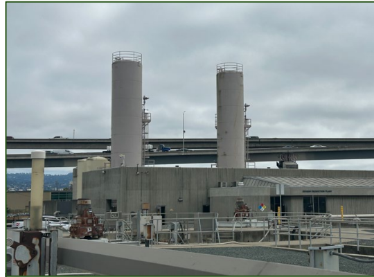
O2 Plant with Cold Boxes (Towers) in Background
