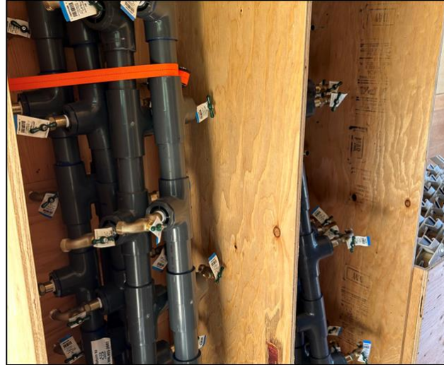
CPOD manifolds inside trailer
