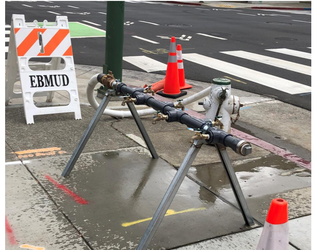
Emergency water manifold
