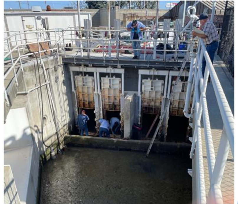
Effluent gates at Oakport Wet Weather Facility
