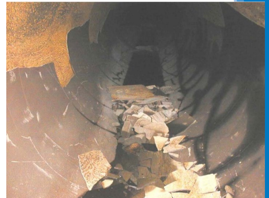
Cement Mortar pieces form debris dams reducing hydraulic capacity
