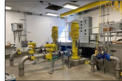
Bayfair Pumping Plant
