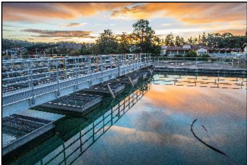
Upper San Leandro WTP
