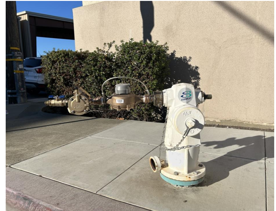
A hydrant meter with a backflow prevention assembly
