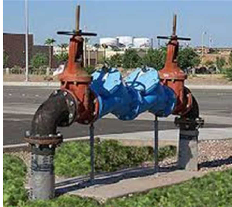
A backflow prevention assembly
