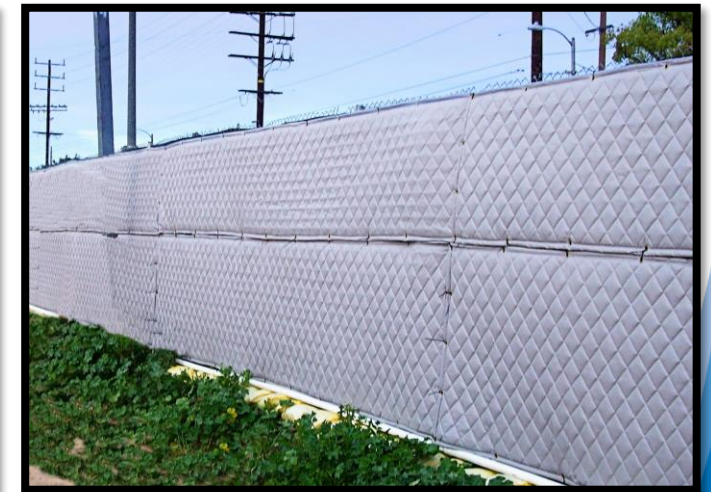
Typical-fence mounted 6-foot high sound barrier
