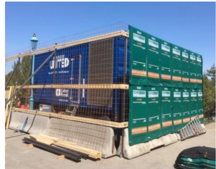
Noise dampening enclosure
