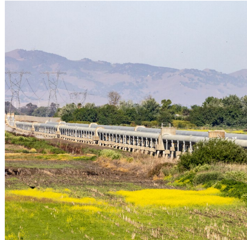
An above-ground portion of Mokelumne Aqueduct
