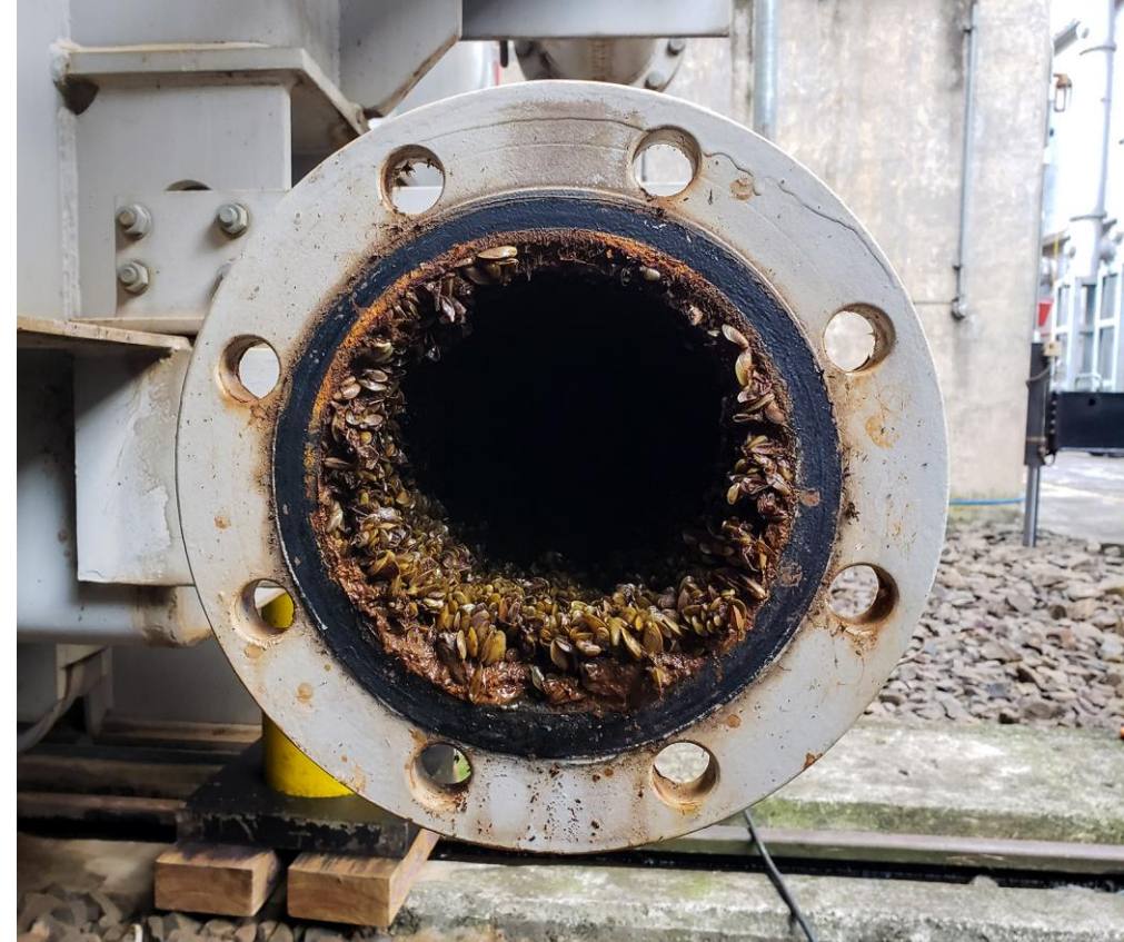
Cooling pipe at a hydroelectric plant in Brazil
