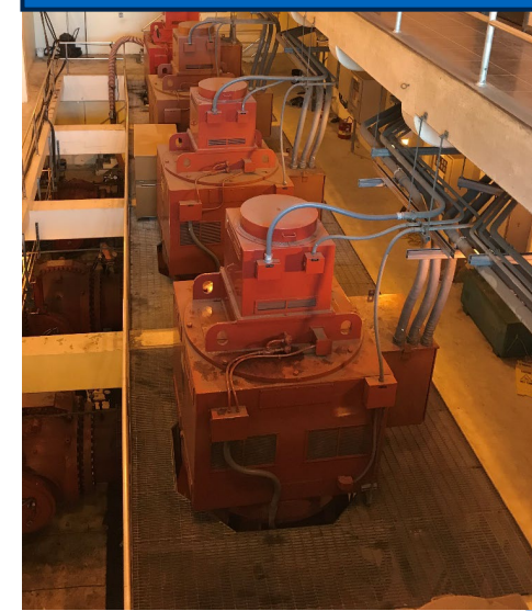
Increasingly Difficult to Maintain
