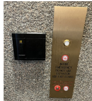
Access Card Reader Upgrades (AB and AMC)
