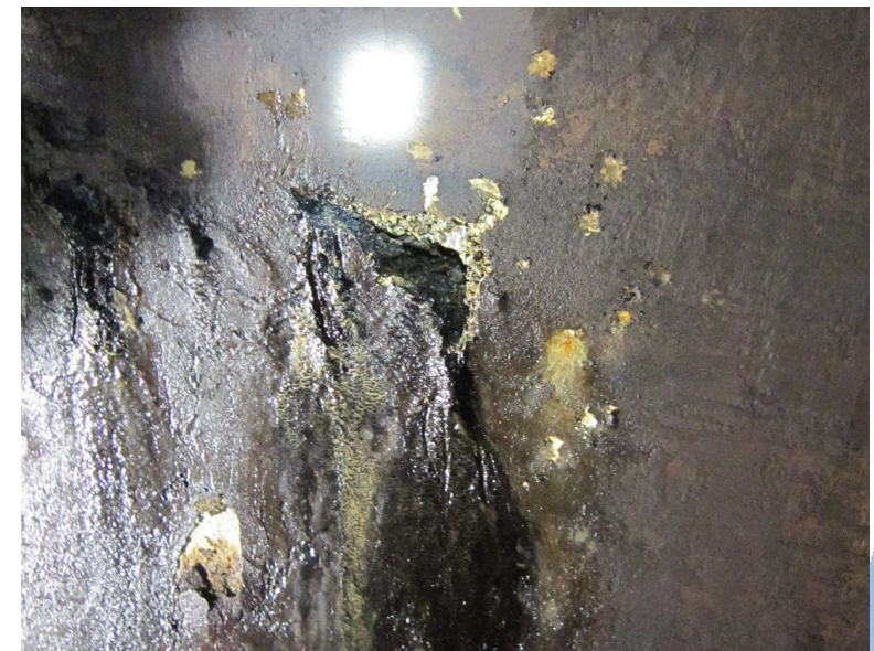
Typical Tunnel Lining Defect
