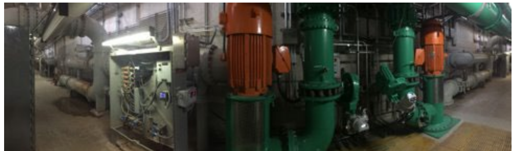
Air Scour Equipment
