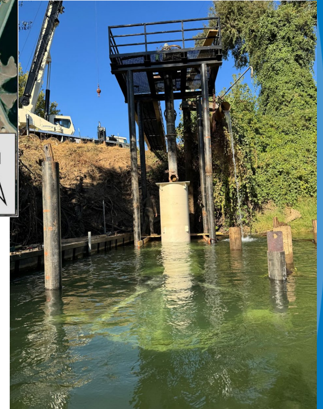
Installed Riparian Diversion Fish Screen
