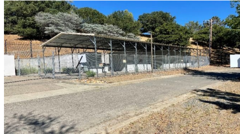
Bryant No. 2 PP existing electrical equipment
