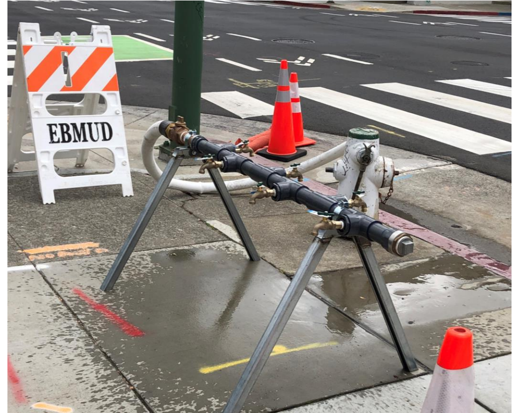
Emergency water manifold at City of Oakland Fire Station (Golden Eagle Exercise)
