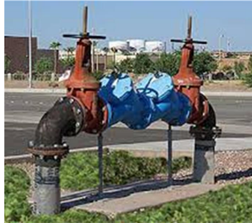
A backflow prevention assembly
