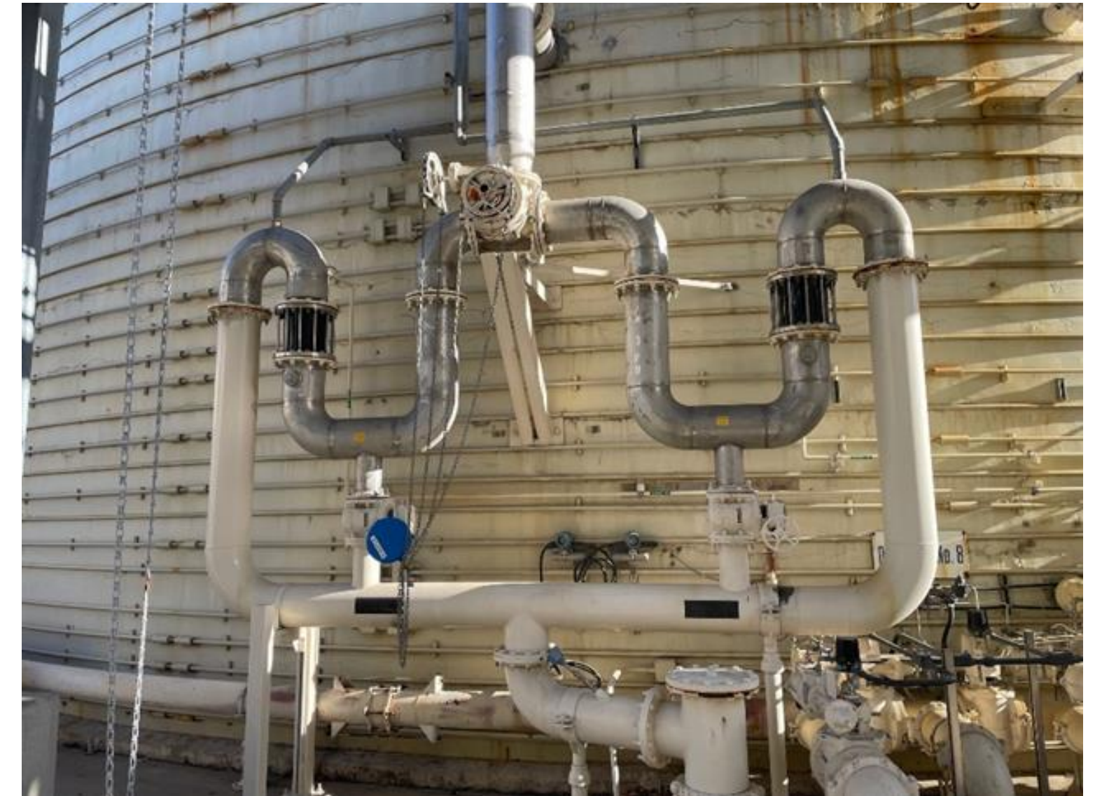
Digester tank three-way valve
