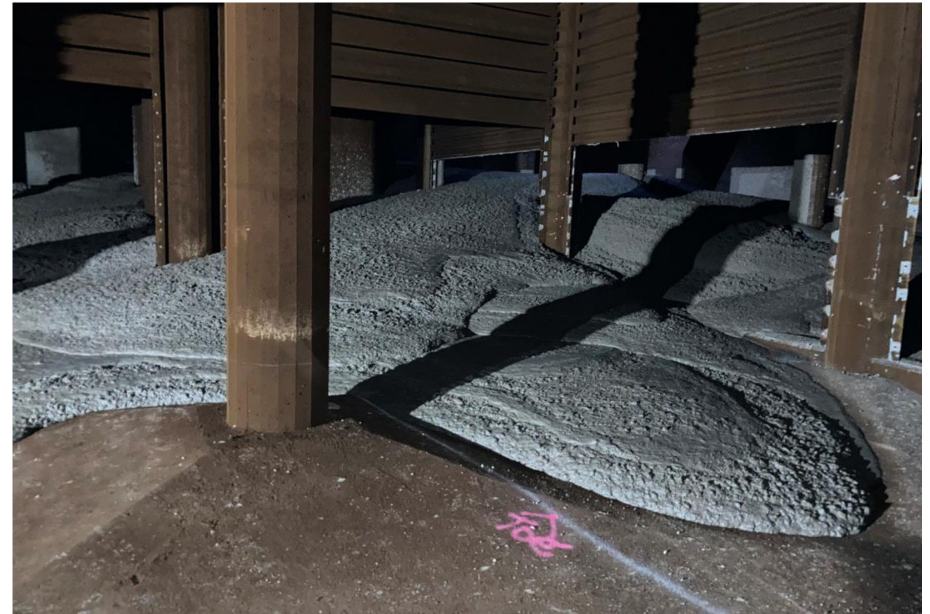
Interior view of native slurry in chlorine contact basin
