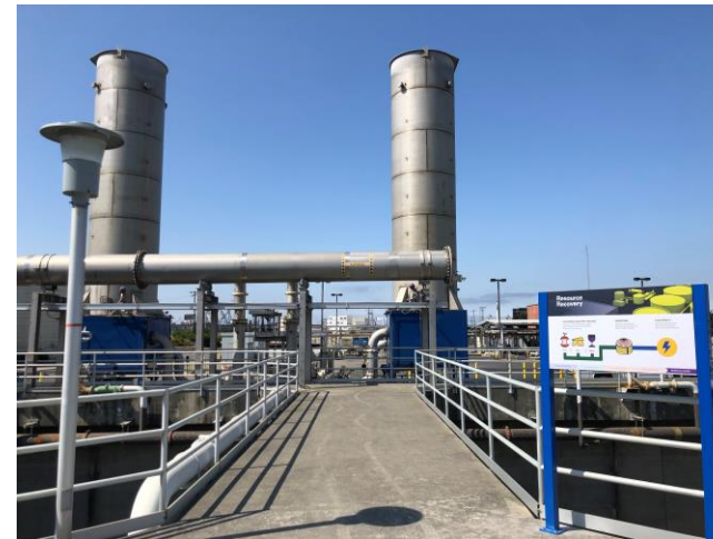
Image of treatment plant with kiosk
