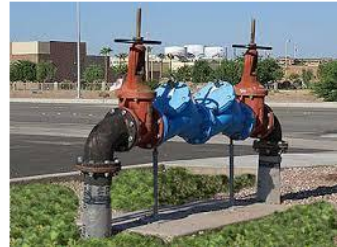
Backflow Protection Assembly (BPA)
