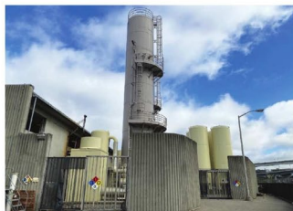
Figure B: Cryogenic oxygen generation plant for high-purity oxygen activated sludge process.
