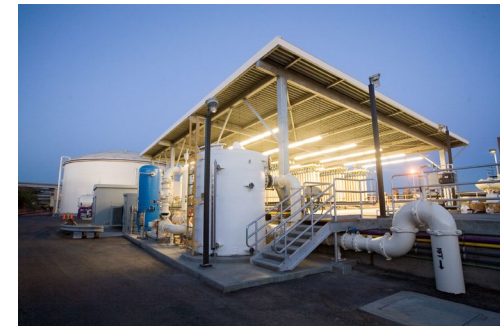
East Bayshore Water Recycling Plant
