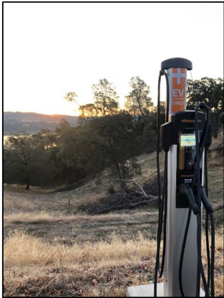
Figure 24. EV charging station with Pardee Reservoir in background.
