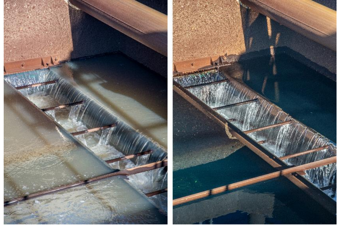
Filter undergoing backwash at Sobrante water treatment plant
