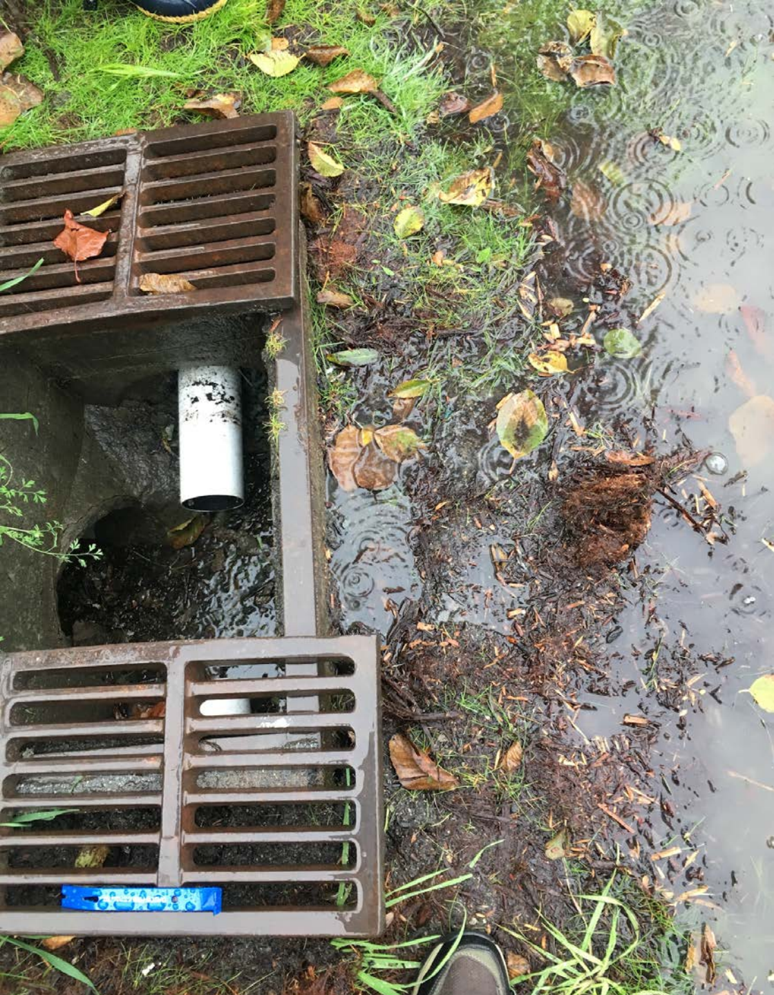
Storm drain overflow
